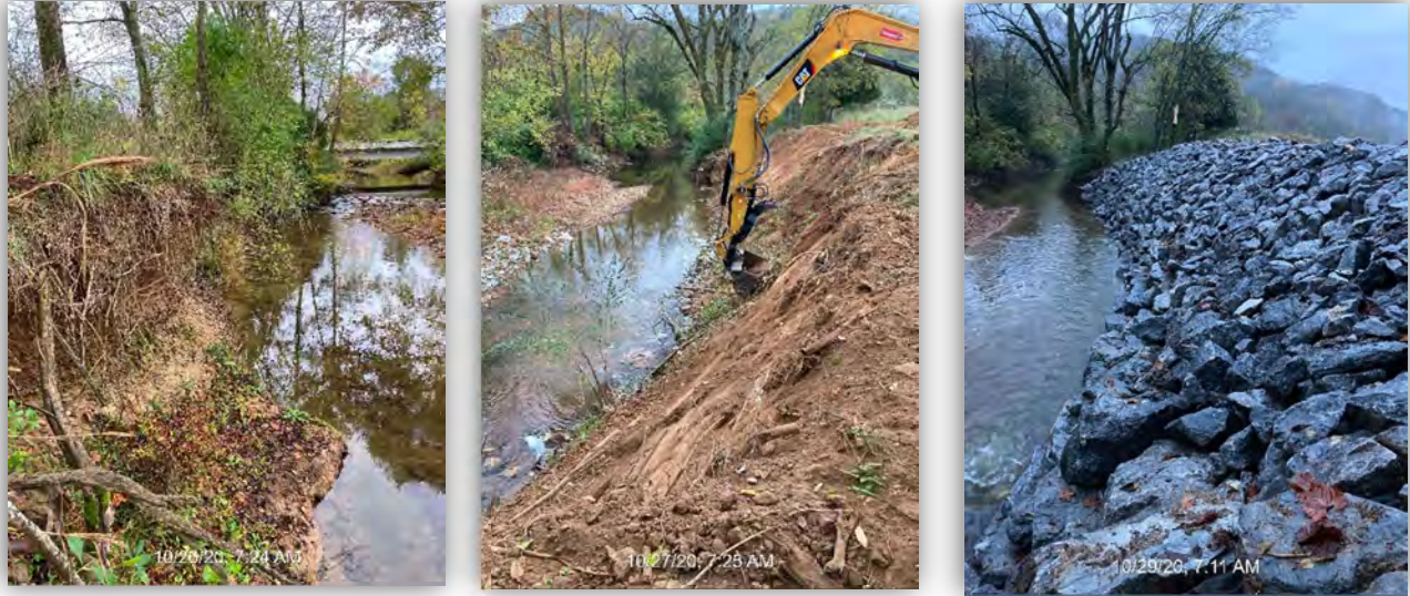
Photographs of the Whites Creek Bank Stabilization Project Before and During Construction
