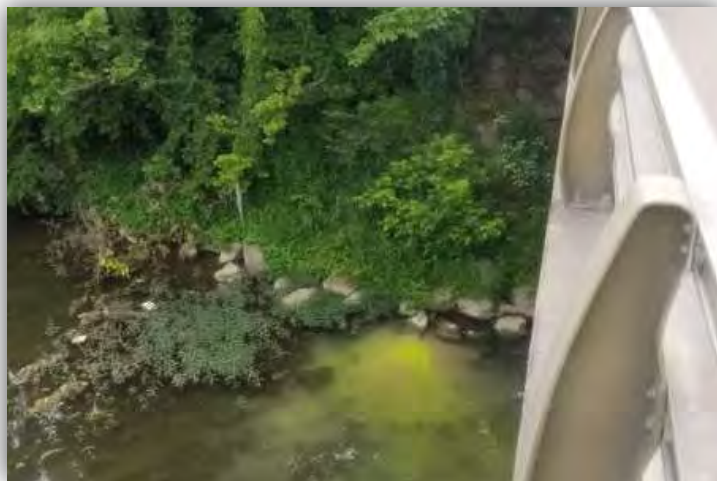
Photographs of the Dye Trace Sanitary Sewer Seep
