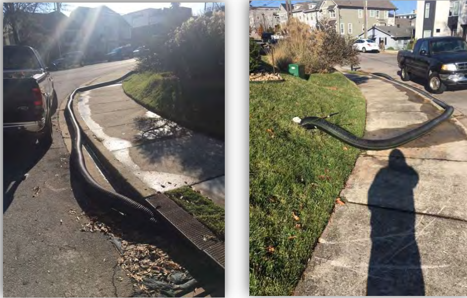
Photo of the Sanitary Wastewater Cross-Connection to the Storm Drain
