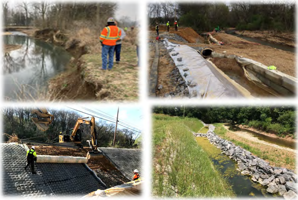
Photographs of the Mankers Creek Bank Stabilization Project Before, During and After Construction
