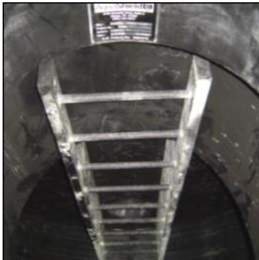
A permanent ingress/egress ladder provides access to filtration chamber. Note metal product identification plate above ladder.
