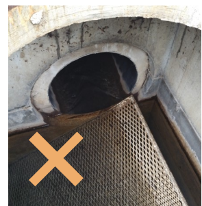
Trash screen displaced
