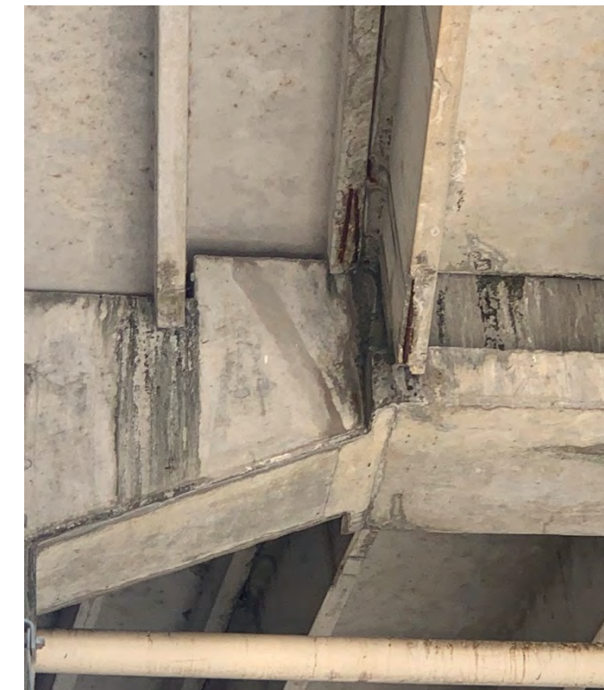
Exposed corroding rebar at precast concrete stems
