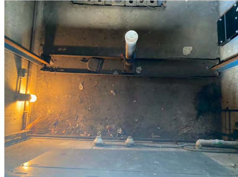
Pits have trash and debris and need additional cleaning
