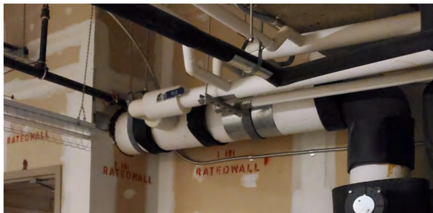
Fire proof caulking not observed at plumbing penetrations through rated walls
