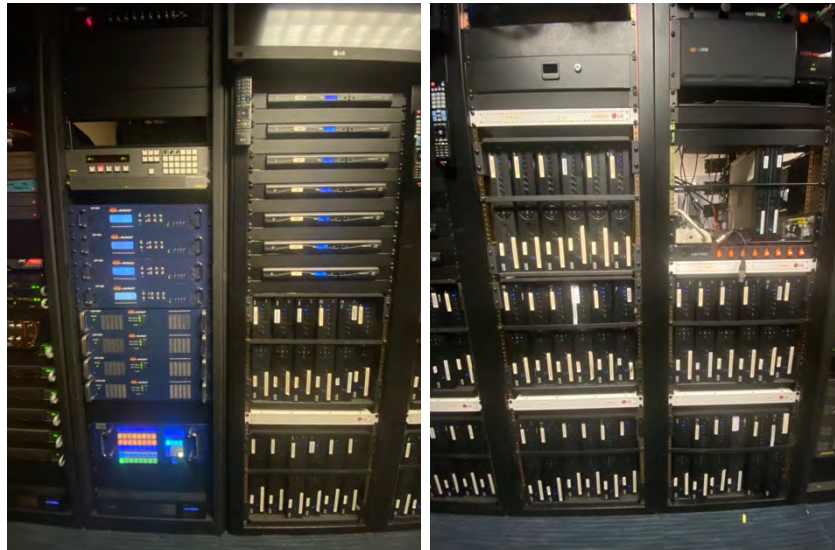
MATV headend components and cable set top boxes
