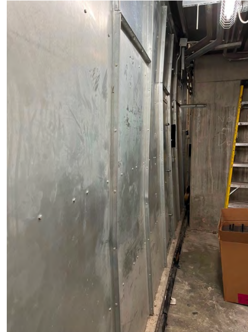
Buckled return air plenum AHU 3B1
