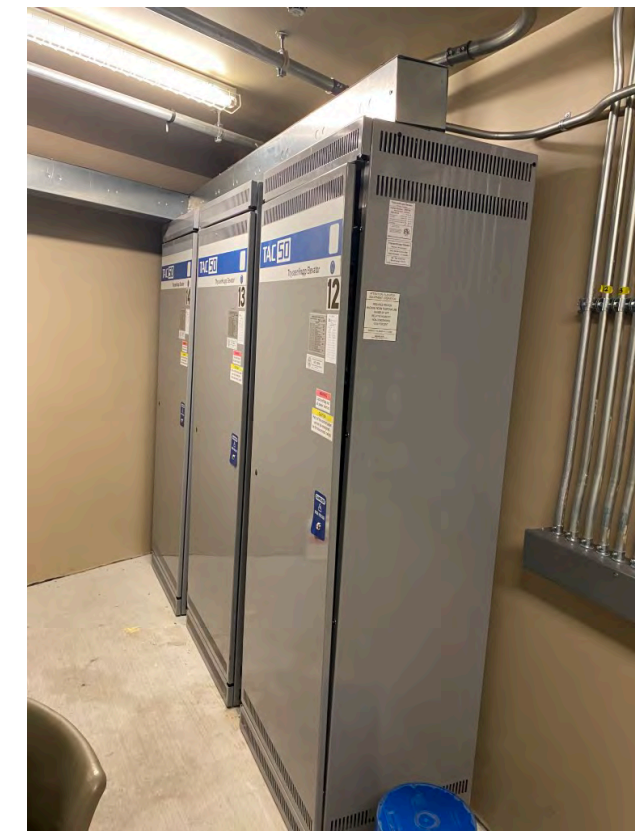
Typical controller layout in the controller rooms
