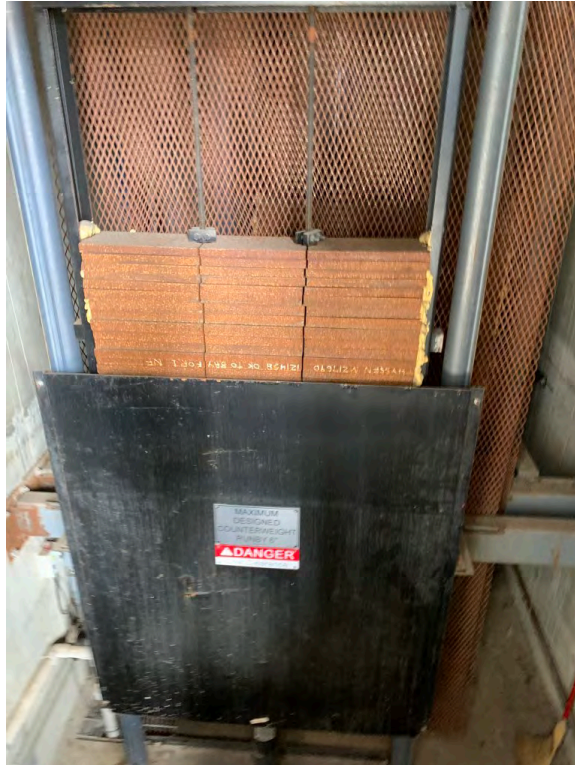
Counterweights and equipment are rusting due to high moisture levels in the hoistway
