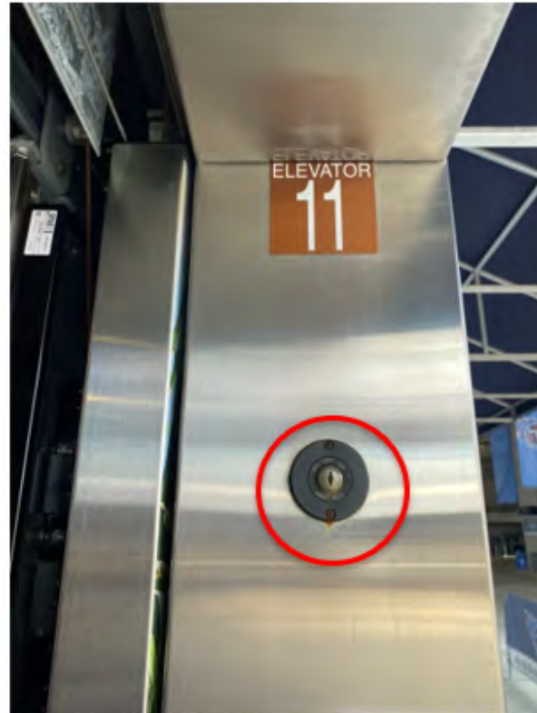
Access key switches are showing signs of rusting
