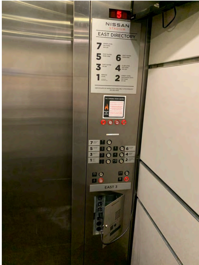
Typical car operating panel for elevators #1-#8
