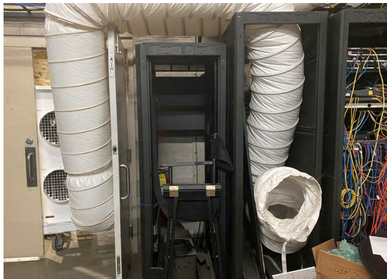
Truck dock head end room with portable HVAC
