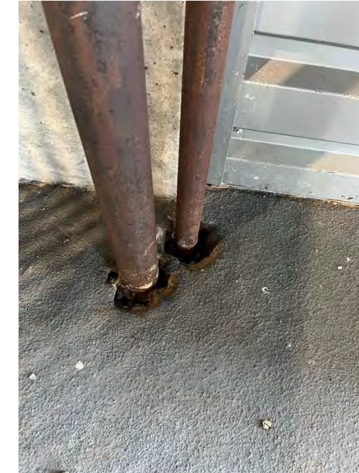
Corrosion on piping exterior and missing slab penetration sleeve/collar
