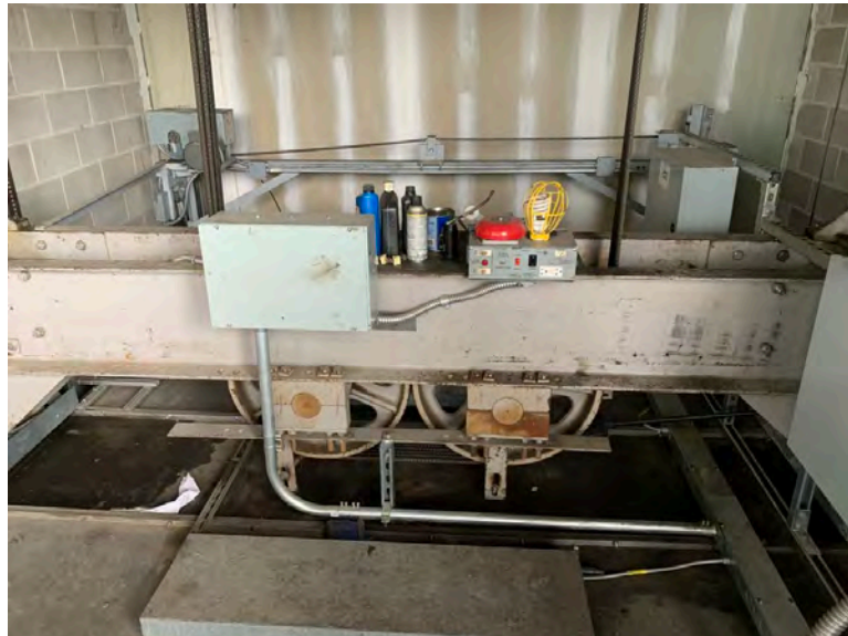
Freight elevator #5 cartop has material and parts stored on top
