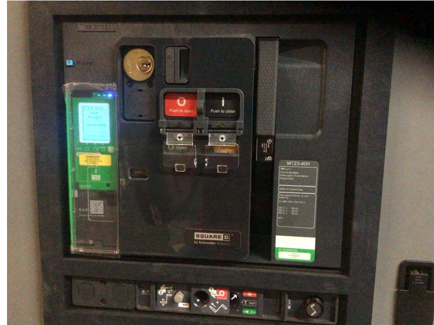
New main circuit breaker
