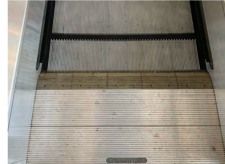
Comb plates on all units have faded and are non-contrasting in color
