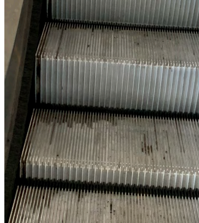
Escalator steps have residual oil leaking from step chain lubrication
