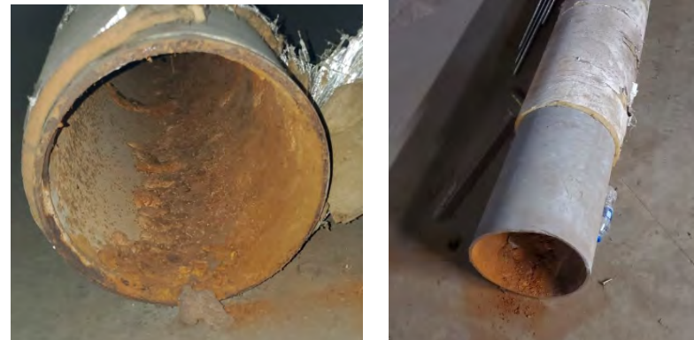
Domestic water galvanized steel pipe corrosion
