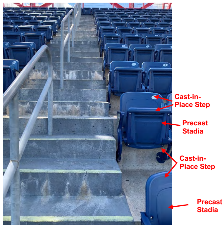
Upper bowl infill step deterioration prevalence
