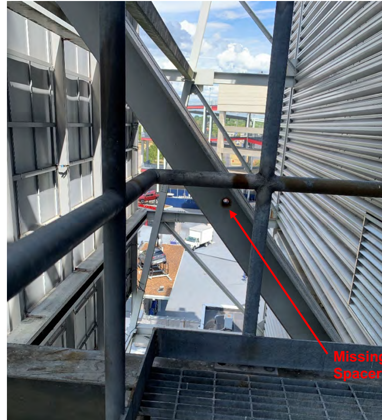
Missing spacer bolt at angle bracing
