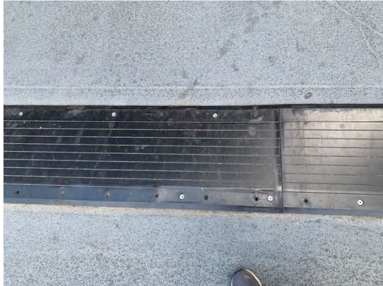
Expansion joint cover anchored at both sides of joint
