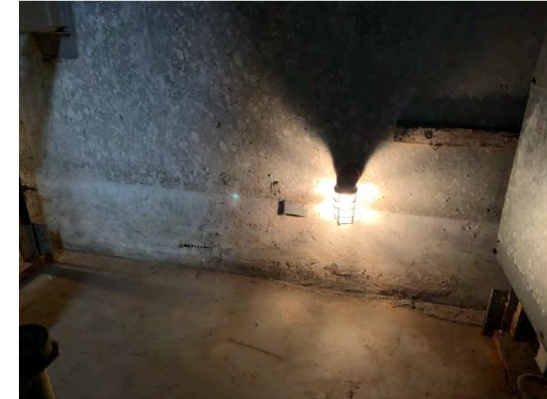
The pit equipment is showing signs of rust
