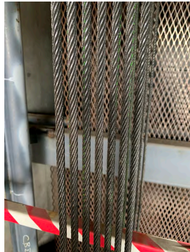
Hoist ropes have slight crown wear and tensioning, and lubrication is needed
