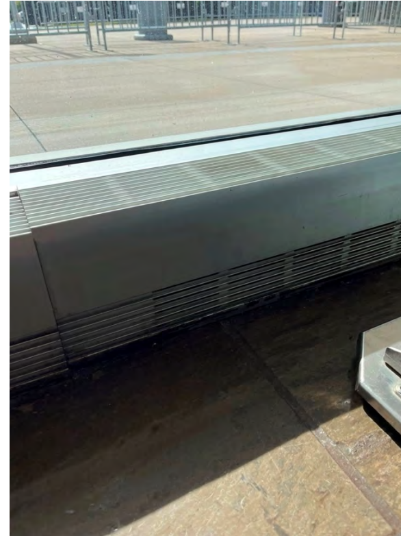
Baseboard heaters in Quad A
