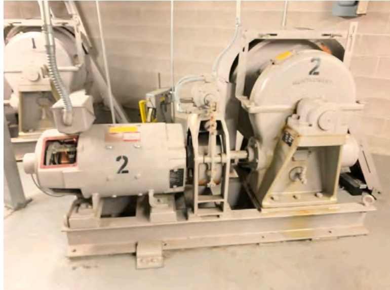
Original Montgomery/KONE 1996 Hollister Whitney 63-OH geared machines
