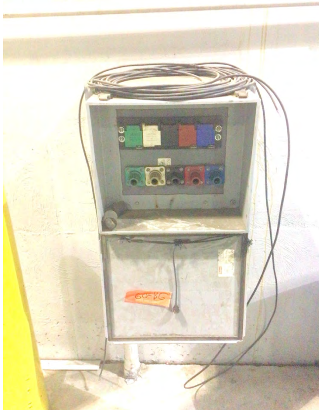
Existing show power panel
