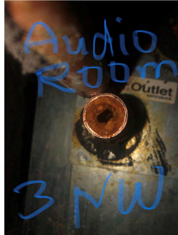
Chilled water scaling build-up within fan coil unit
