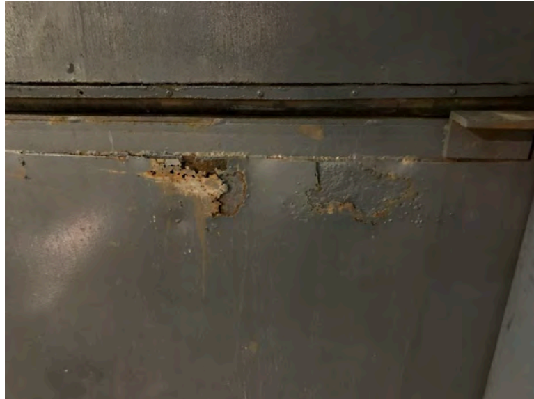
Freight elevator #4 bottom landing door is rusted, and the metal is separating
