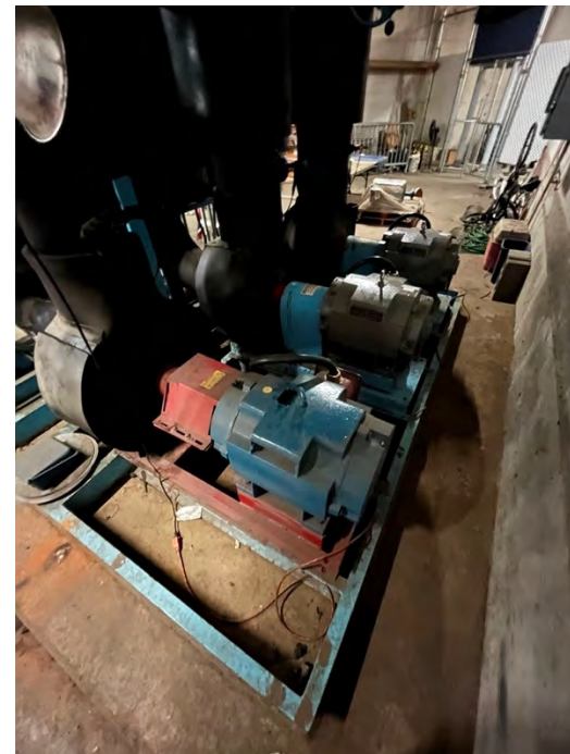
Chilled water pump skid
