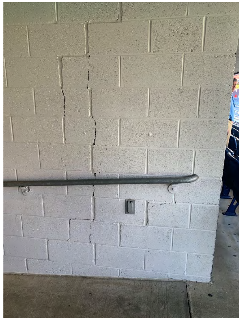
Cracking in CMU vomitory wall at main concourse
