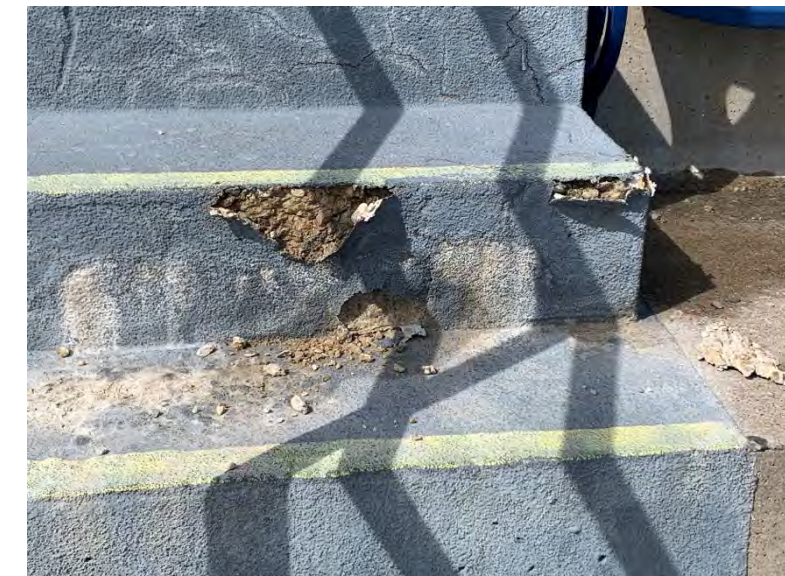
Seating bowl infill step deterioration
