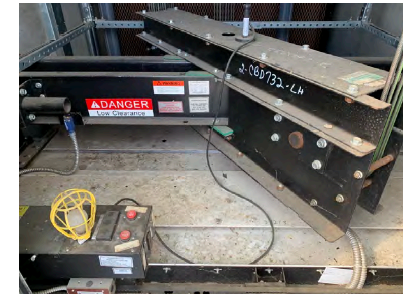
Car tops are dirty and in need of cleaning and rusted surfaces should be painted
