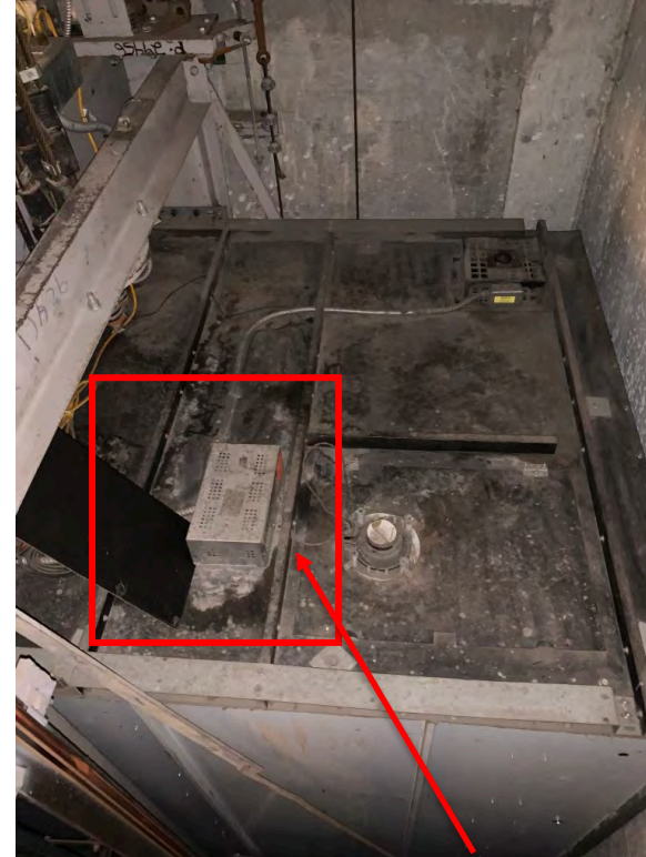
Passenger elevator #1 has signs of water damage and dust cover is being stored on the cartop and should be reinstalled
