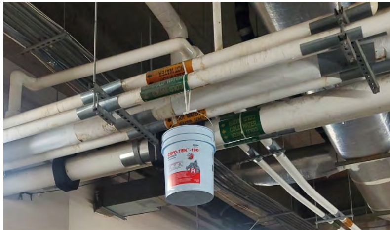
Lack of shutoff valves on domestic water branches
