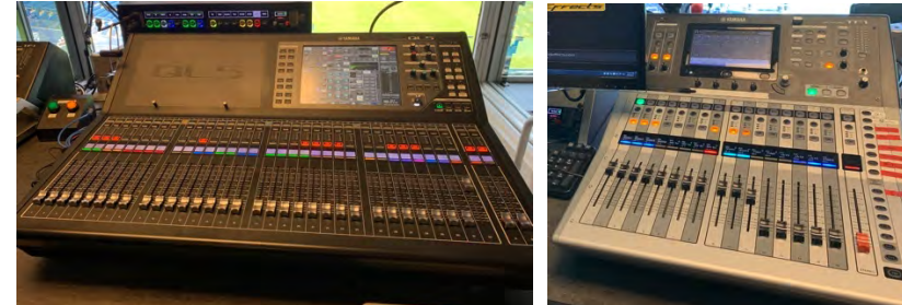
Audio consoles located in audio control room
