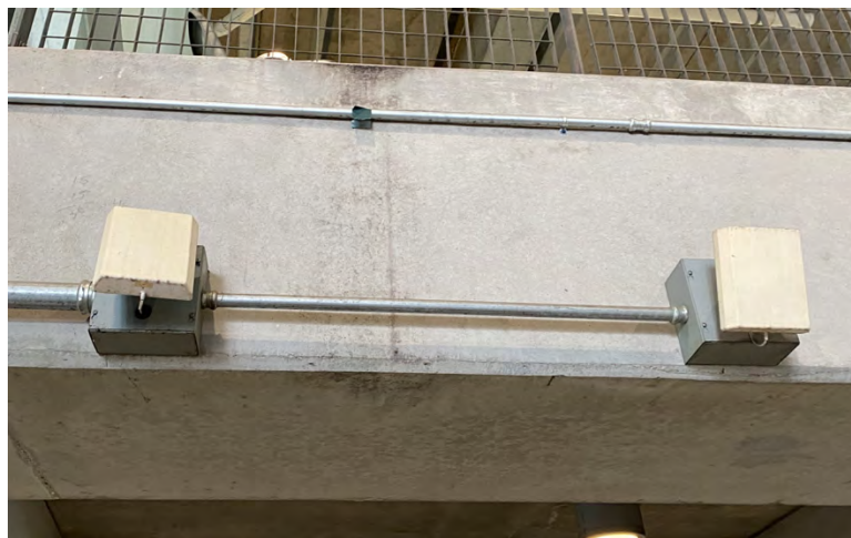
Existing DAS antennas with carrier responsible for upgrades
