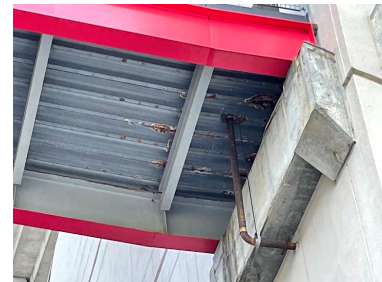
Corrosion of metal deck at access ramps
