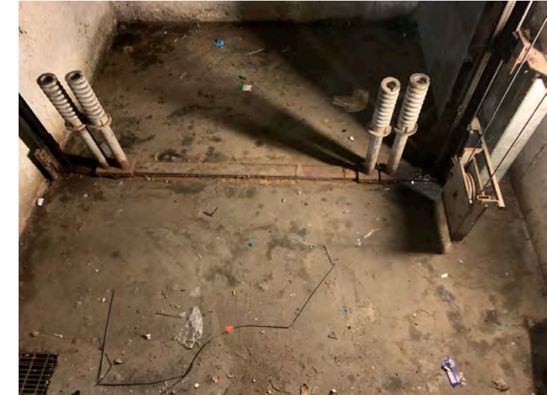
Elevator #4 pit area has signs of water related issues and equipment is rusting
