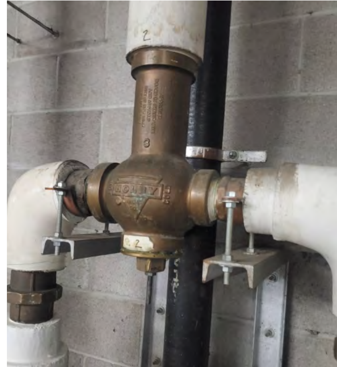
Domestic water galvanized steel pipe corrosion
