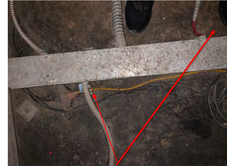
Extension cord is laying on cartop and greenfield is pulled loose from the duct fitting
