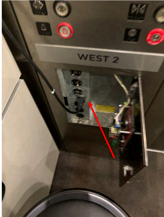
Fans are plugged into the car operating panel behind inspection doors
