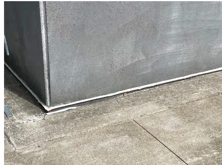
Plaza slab settlement at exterior wall
