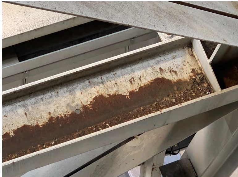
Corrosion at scoreboard signage girt
