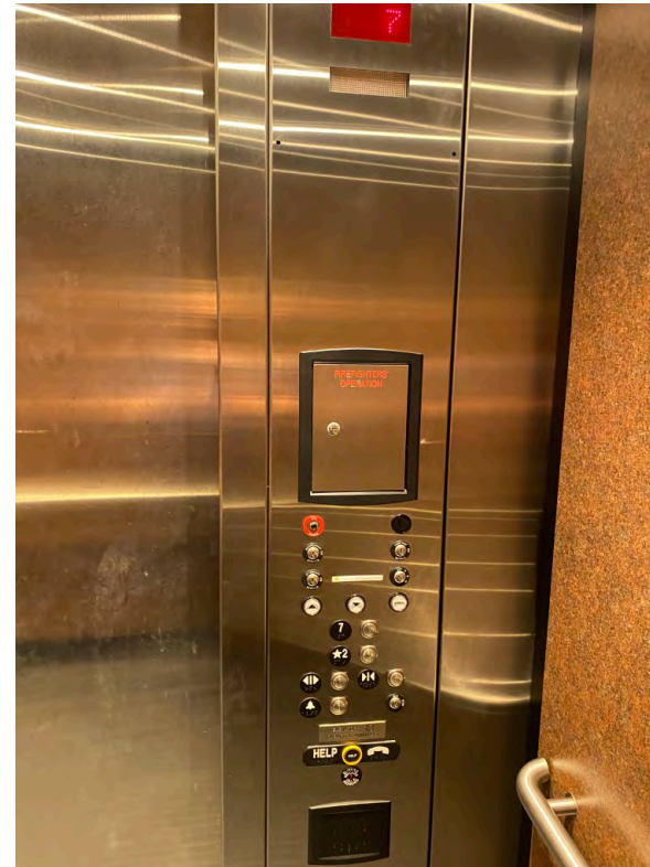
Typical car operating panel and fixtures for these elevators
