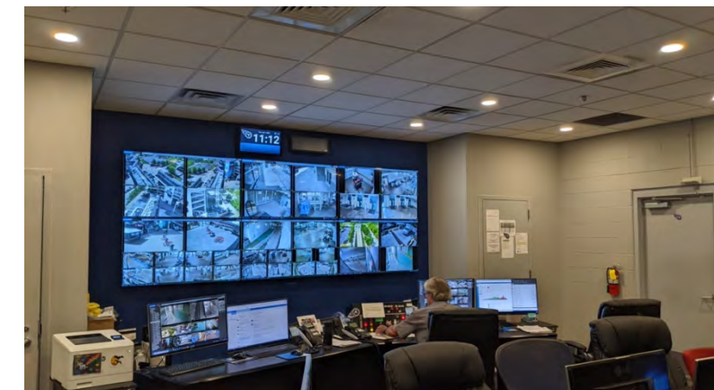
Main security control room with video wall and individual workstations
