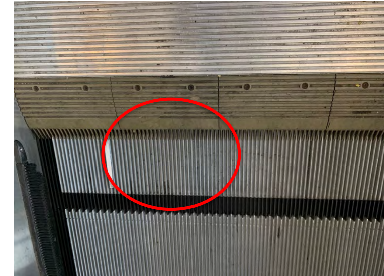
Upper landing comb plates gap to steps in excess of 5mm and plates have faded color and are non-contrasting which is required by code
