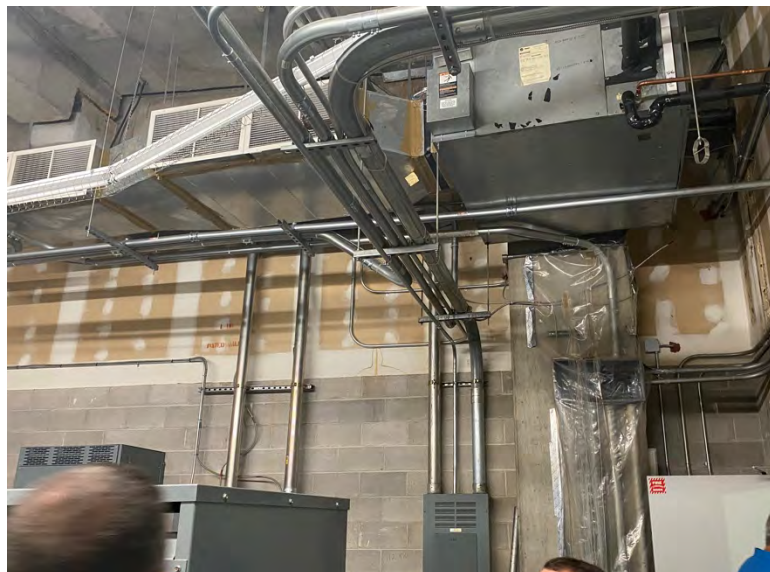
Expansion joint above electrical equipment
