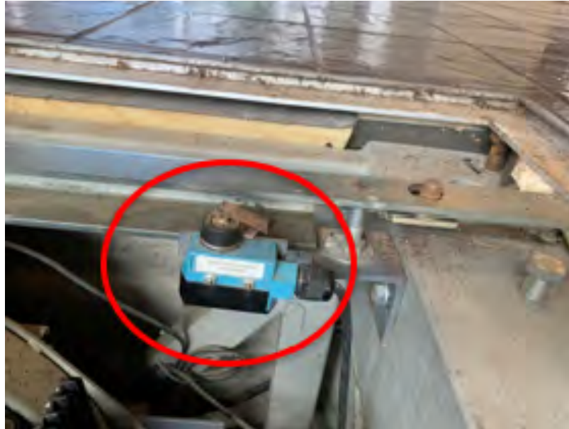
Microswitches inoperable due to metal shim depressing the plungers
