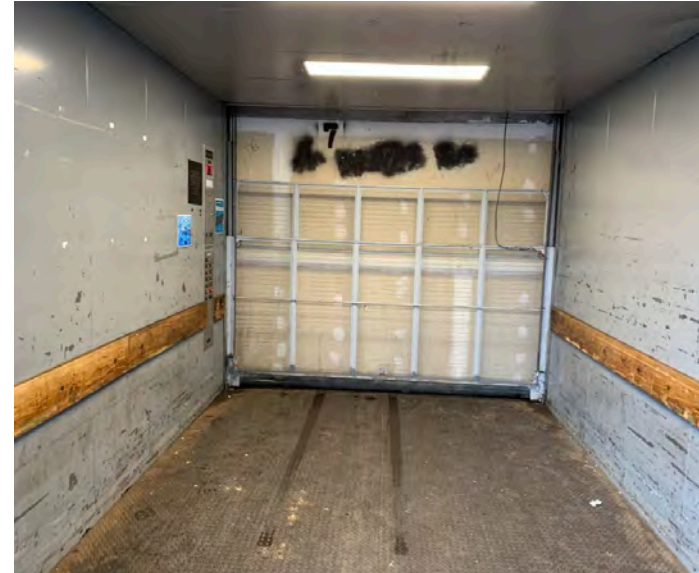
Freight elevator #4 cab enclosure
