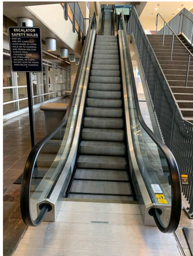
Escalator view from the 2 nd landing looking up to long unit above
