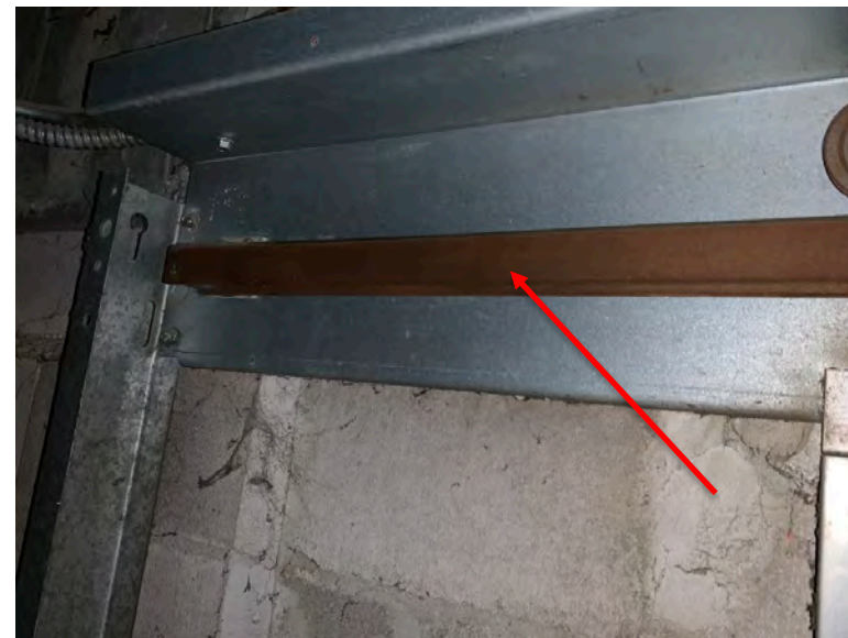
Hoistway door tracks are showing signs of rust
