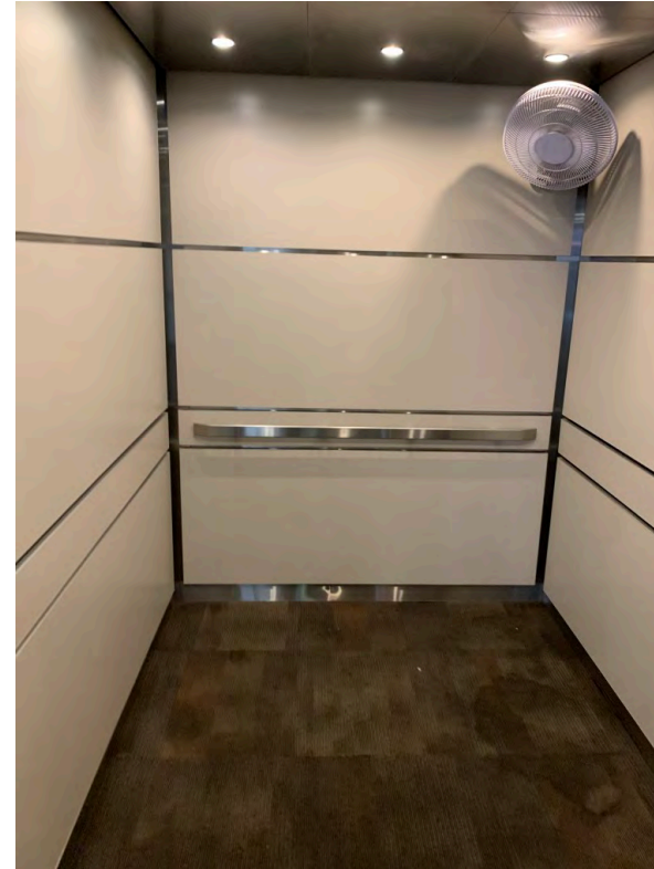
Temporary fans have been installed in the elevator cabs and are used during warm conditions
