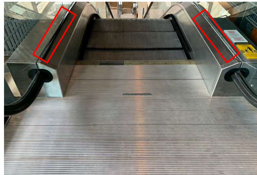
Upper landing plastic skirting cover on the right side is missing and damaged on the left side
