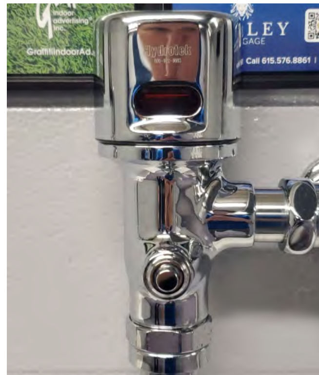
Hydrotek sensor flush valves serving water closets and urinals
