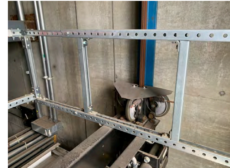
Car tops are equipped with handrails and roller guides roughly operating
