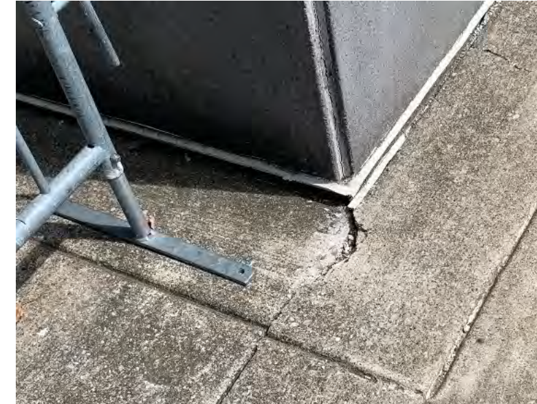
Plaza slab settlement at exterior wall
