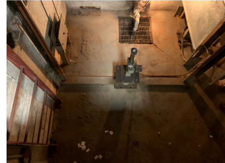
No counterweight run by data tags in place and trash was found on pit floor
