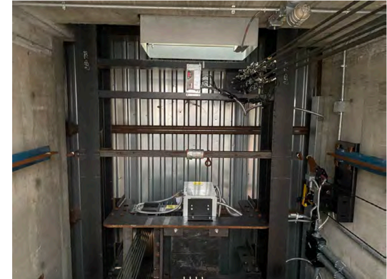
Typical rust on equipment in overhead on express cars
