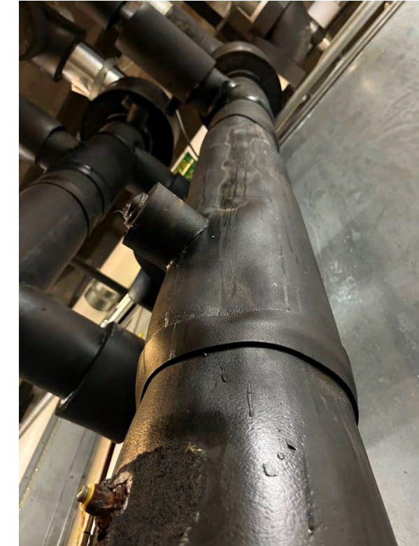
Compromised chilled water insulation
