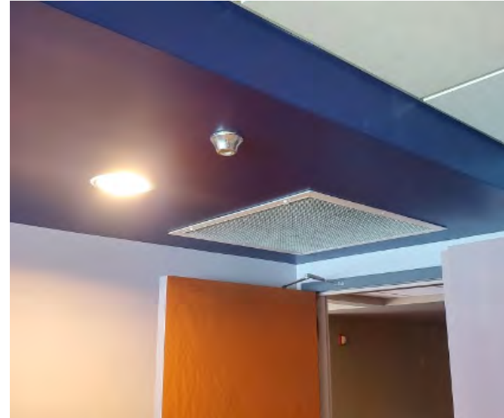
Auxiliary condensate terminations above suite entrances and lavatories
