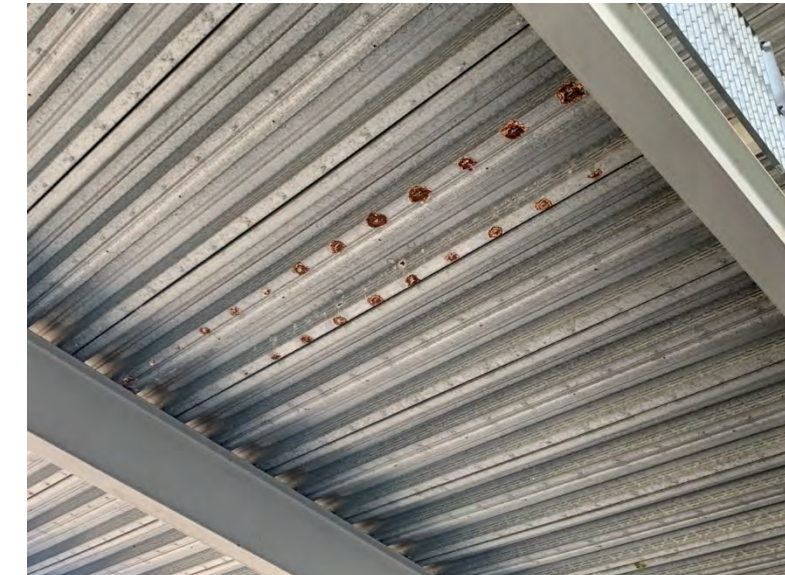
Corrosion of metal deck at access ramps
