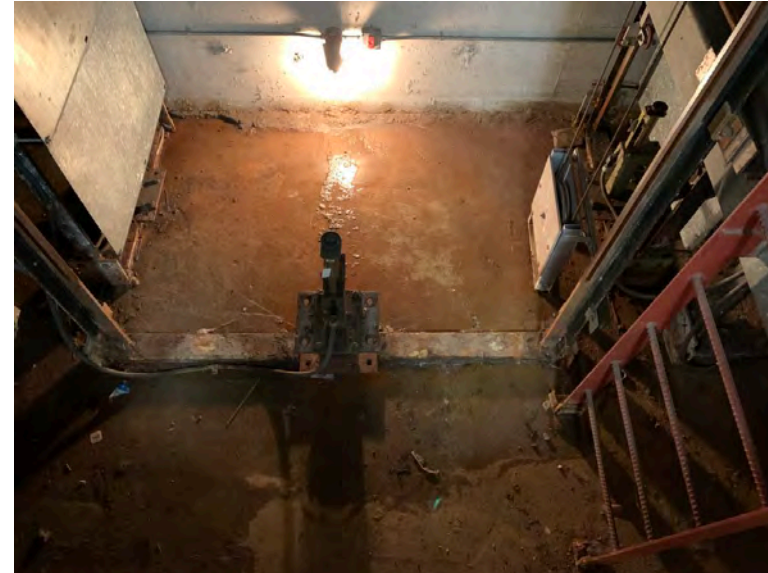
Elevator #6 pit has standing water and the equipment is rusting
