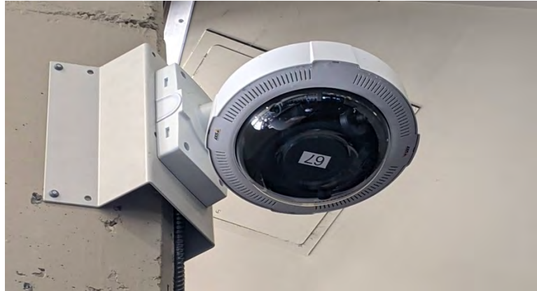
Security camera with corner mounted multi-imager
