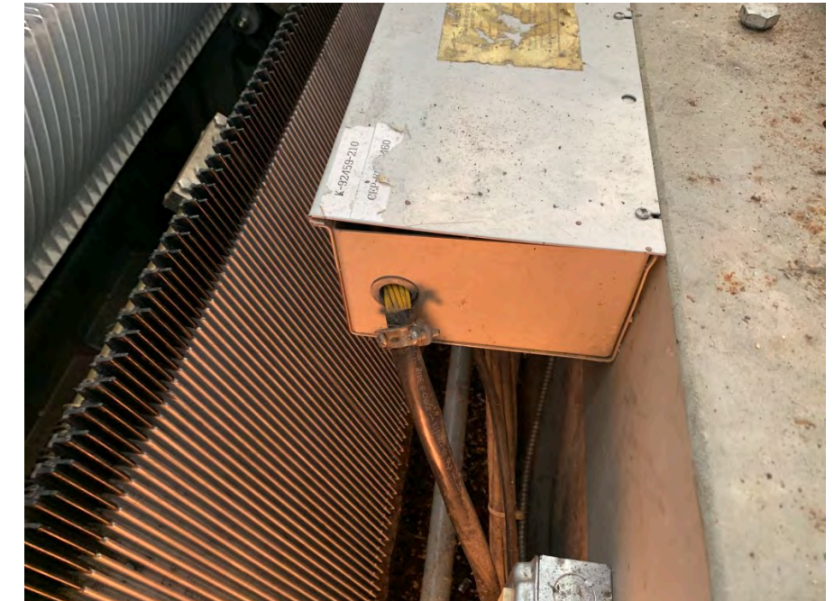
Wiring pulled loose from junction box at the lower end pit
