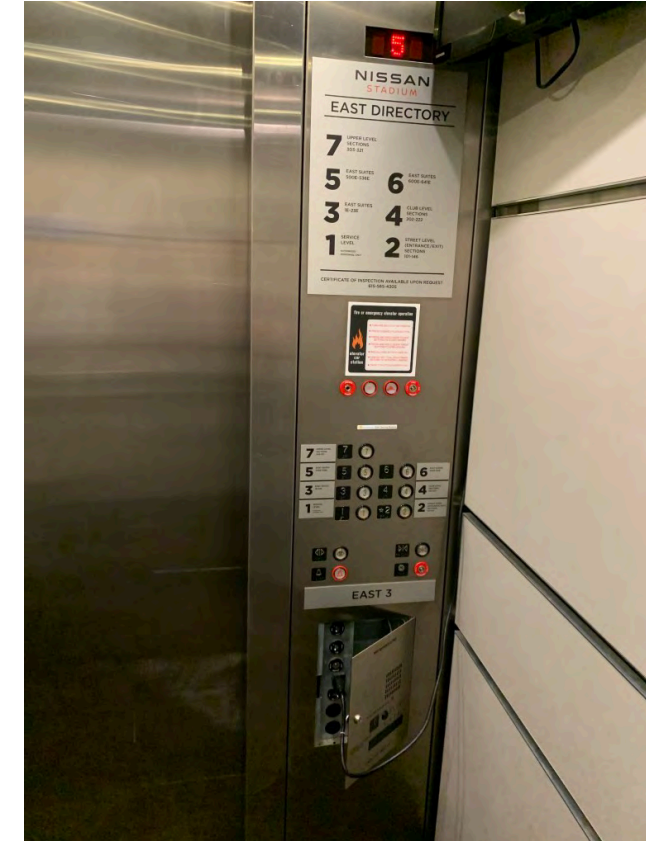
Typical car operating panel for elevators #1-#8
