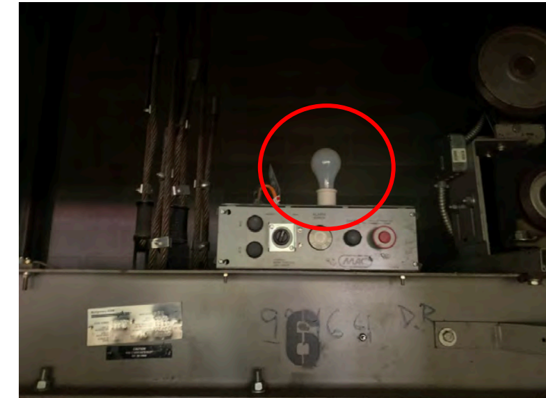
Light bulb guard missing from inspection station
