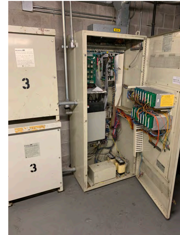
Original Montgomery/KONE 1996 controller and drive
