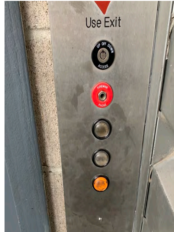
The top floor hall door station plastic button covers are discolored making it hard to read the door open and close buttons
