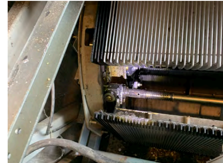
Step chains appear to be well lubricated, and no damaged rollers or step axles were found during the visual inspection
