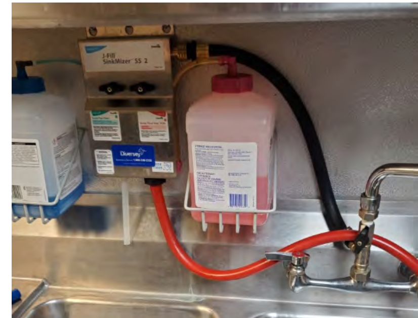
Domestic water tap serving chemical dispenser without backflow preventer
