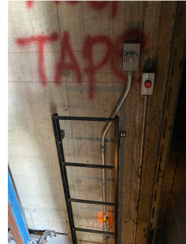
Express elevator pits are missing identification numbers
