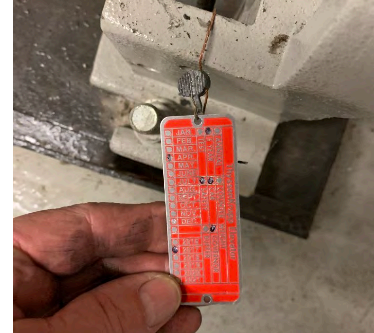
CAT 5 test was performed April 2017 and in overdue for testing
