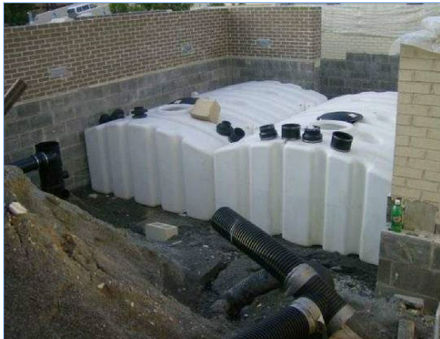
Figure 10.5. Example of two Polyethylene Cisterns (Source: VADCR, 2011)
