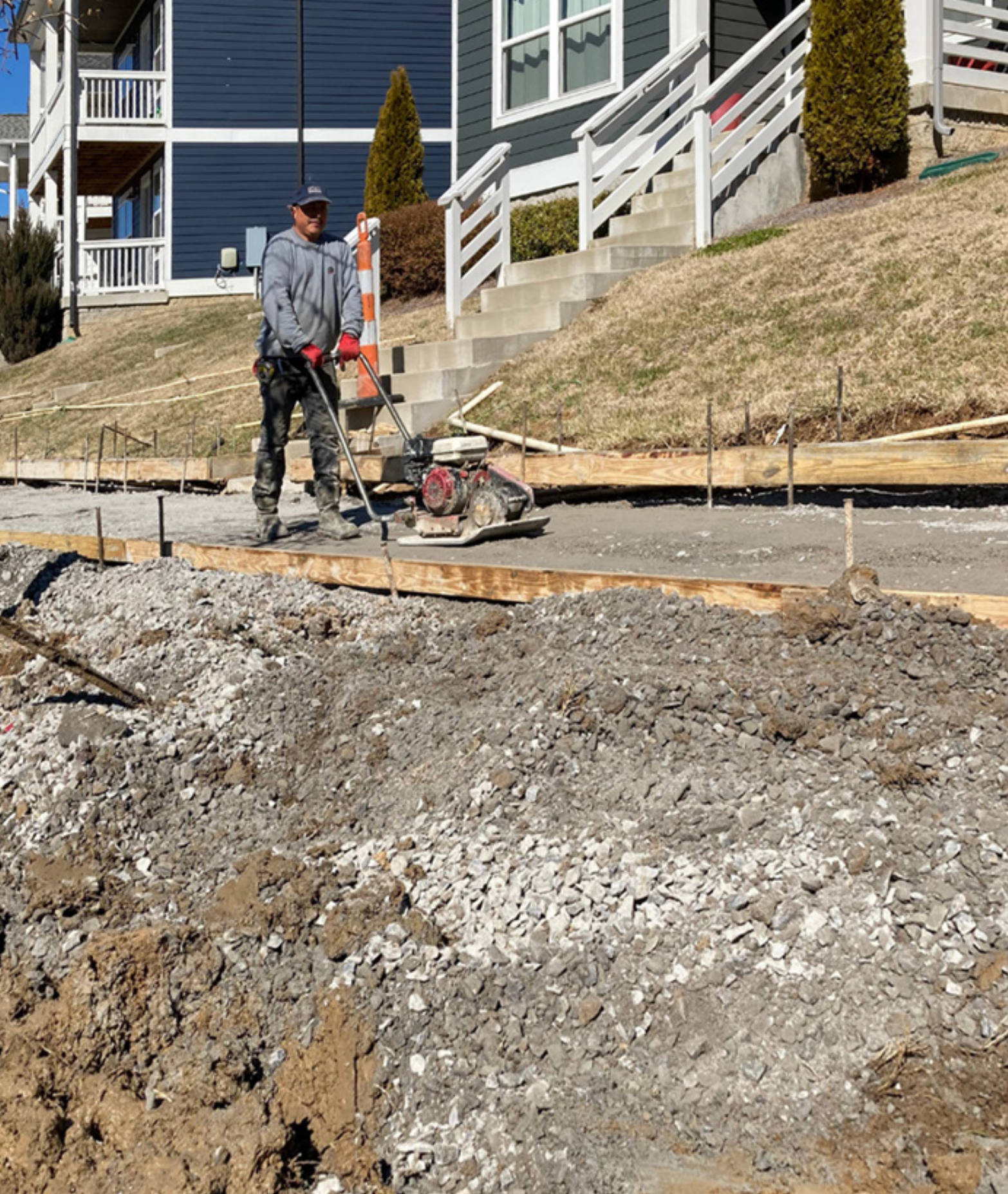
Repairing damaged sidewalks are a proposed improvement included in the TIP
