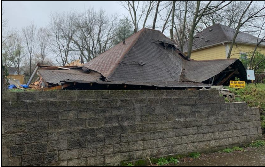
Figure 6. 1112 Boscobel Street after March 25, 2021 storm.
