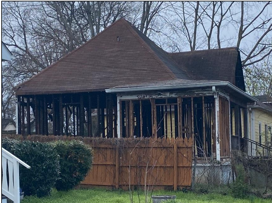
Figure 5. 1112 Boscobel Street prior to March 25, 2021 storm, undated.
