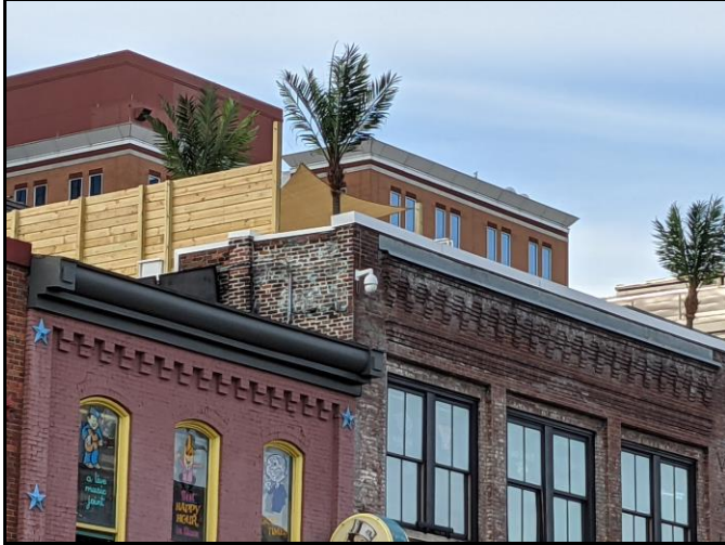
Figure 5. Wall and awning violation at 312 Broadway.
