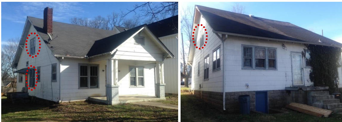
Figures 2 & 3 show the windows on the side facades that are to be replaced.
