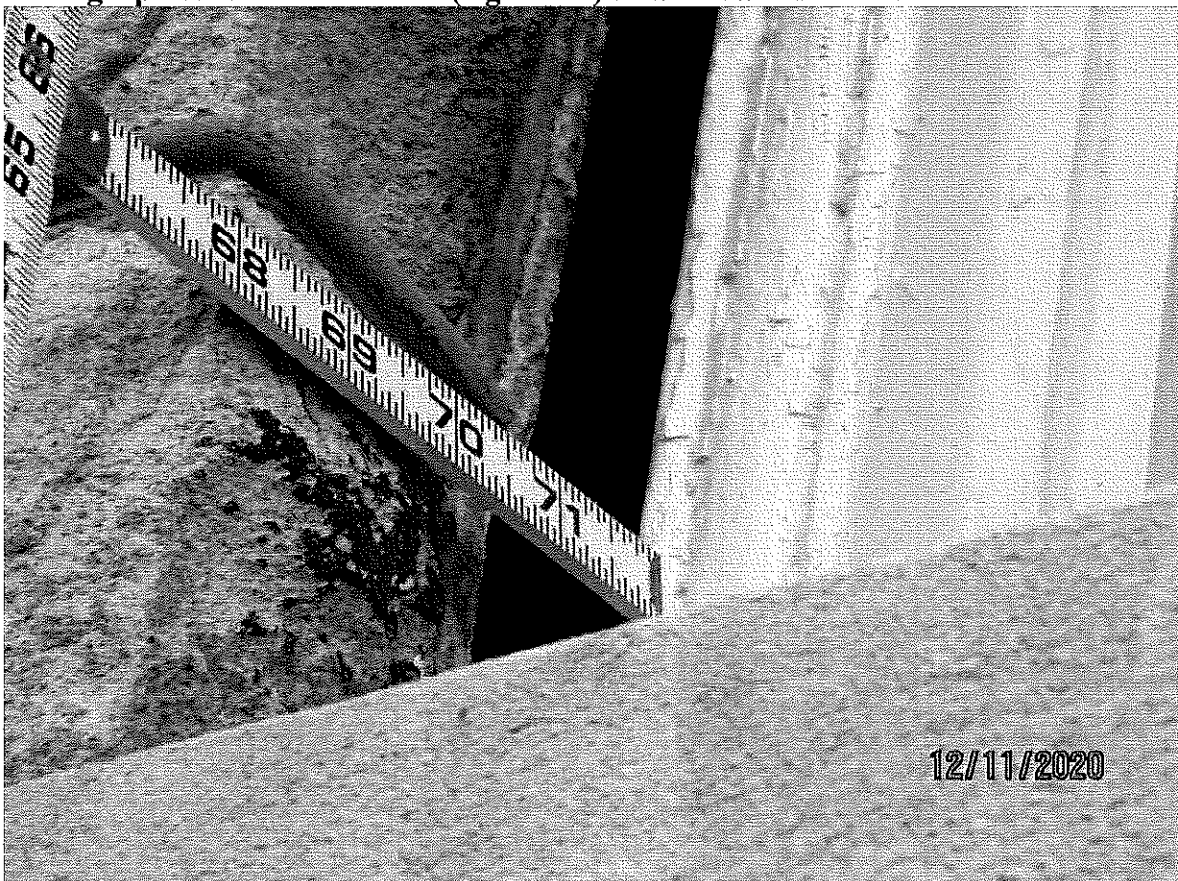
Photograph 8: Wall movement (right side) at window casement.
