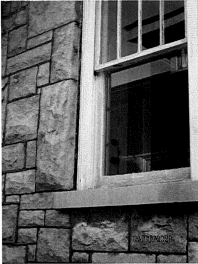
Photograph 13: Wall movement (right side) at window casement.
