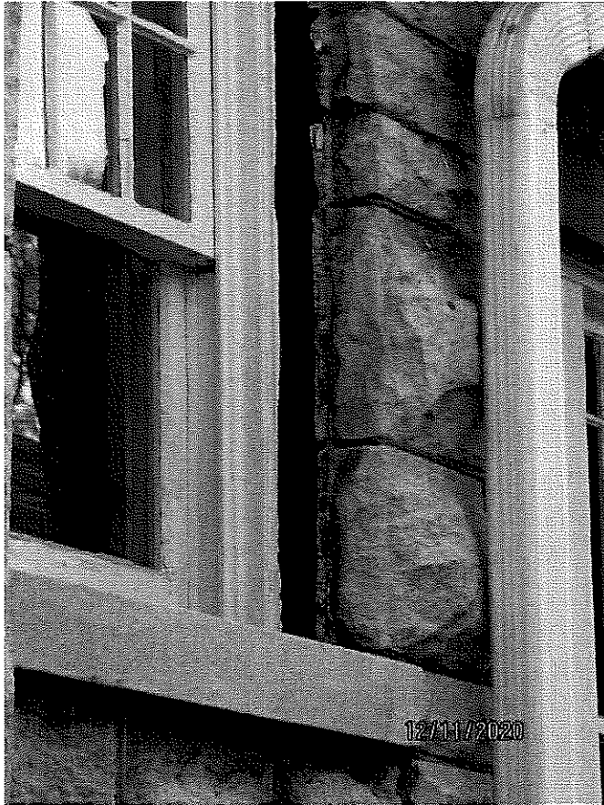
Photograph 9: Wall movement (right side) at window casement.
