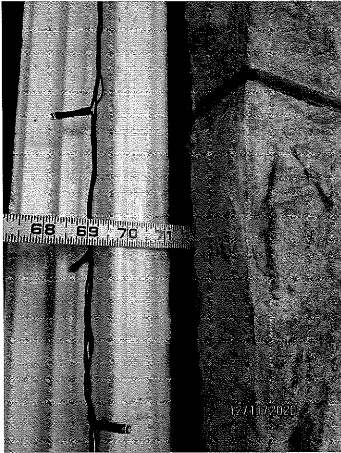
Photograph 5: Wall movement at front wall (right window).
