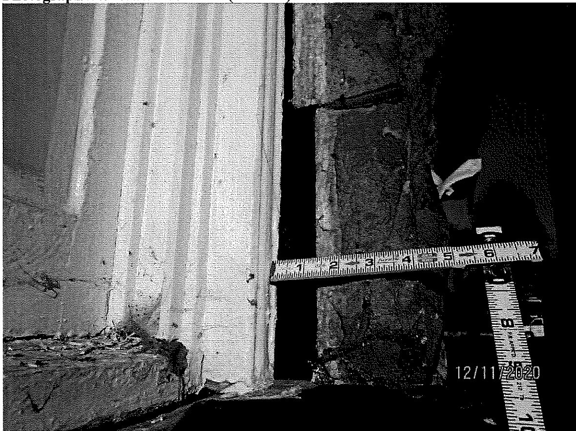
Photograph 24: Wall movement (left side) at window casement.
