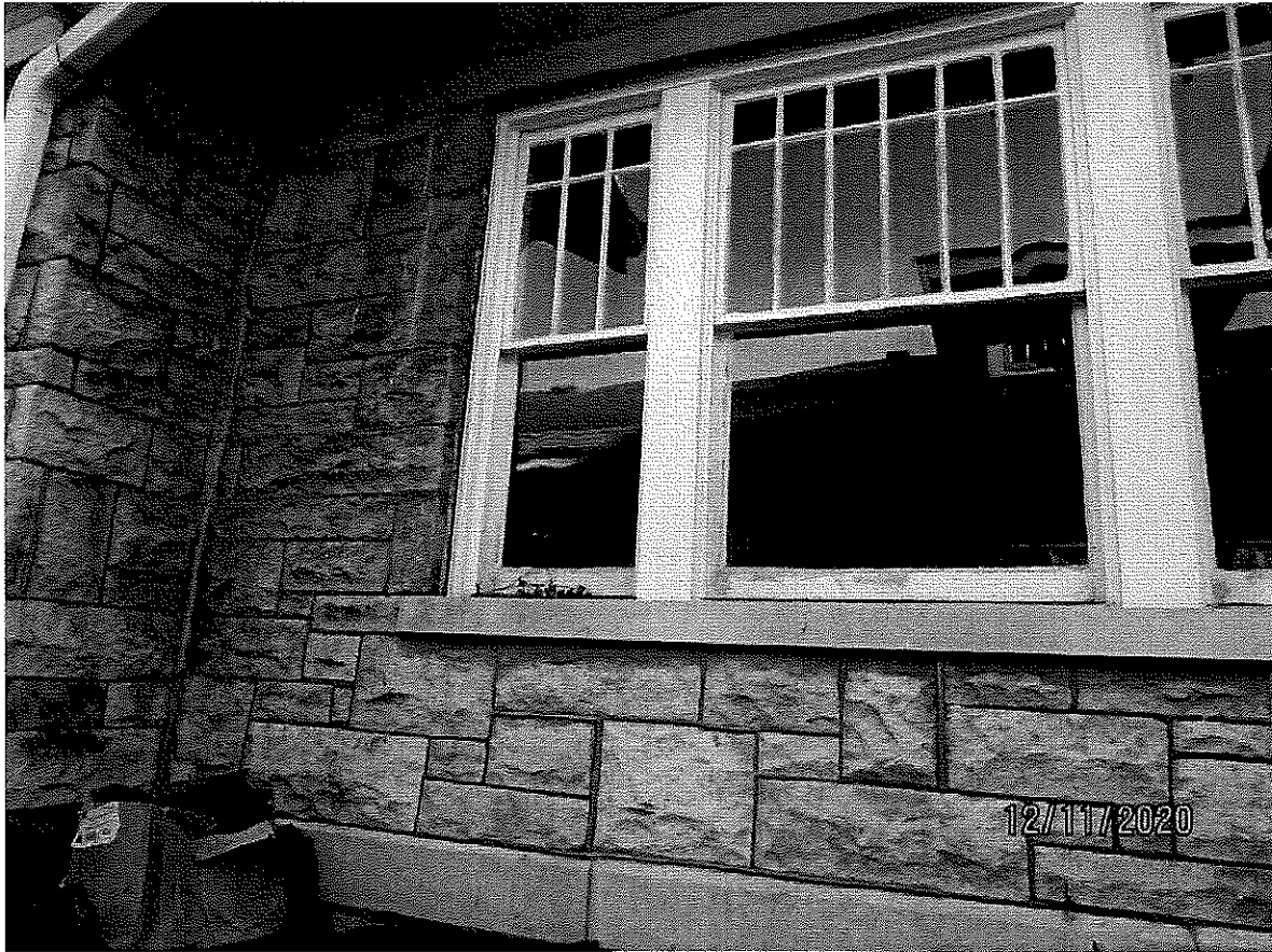
Photograph 11: Wall movement (right side) at window casement.
