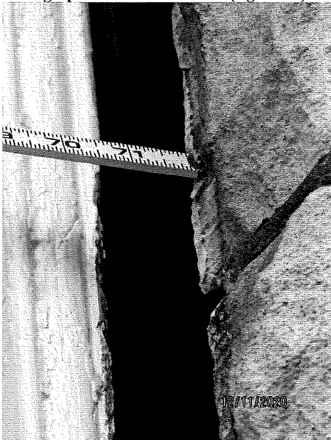
Photograph 10: Wall movement (right side) at window casement.
