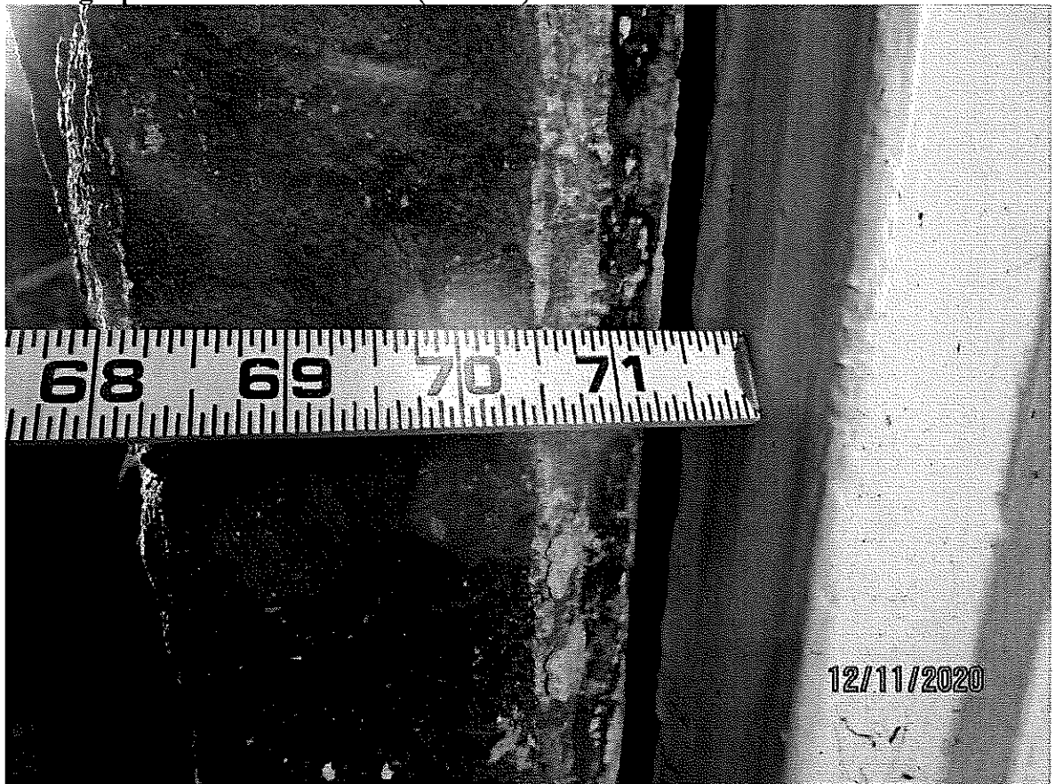
Photograph 22: Wall movement (left side) at window casement.
