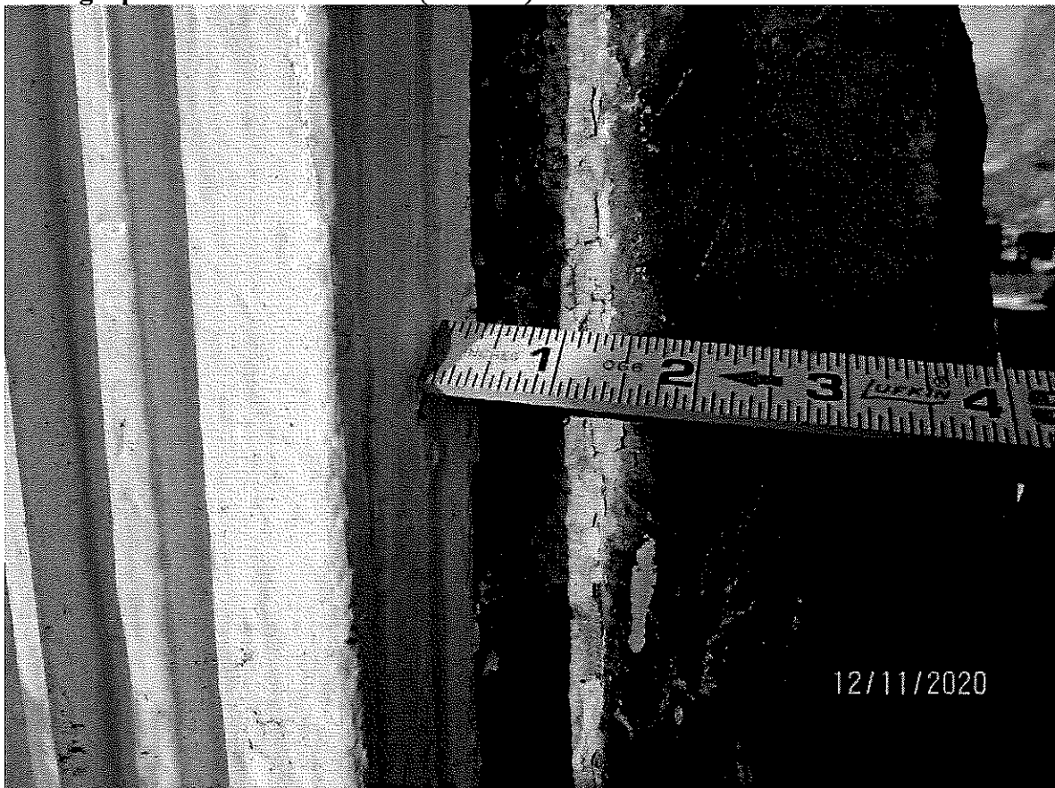
Photograph 20: Wall movement (left side) at window casement.
