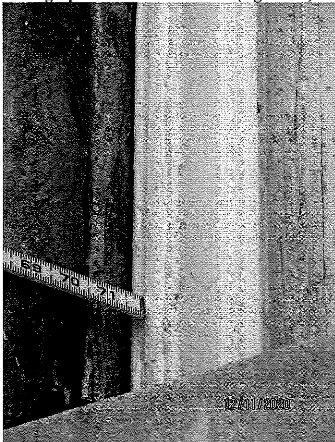
Photograph 12: Wall movement (right side) at window casement.
