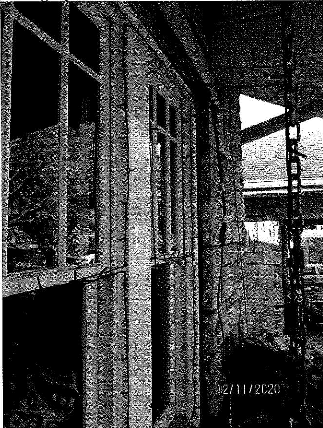
Photograph 4: Wall movement at front wall (right window).
