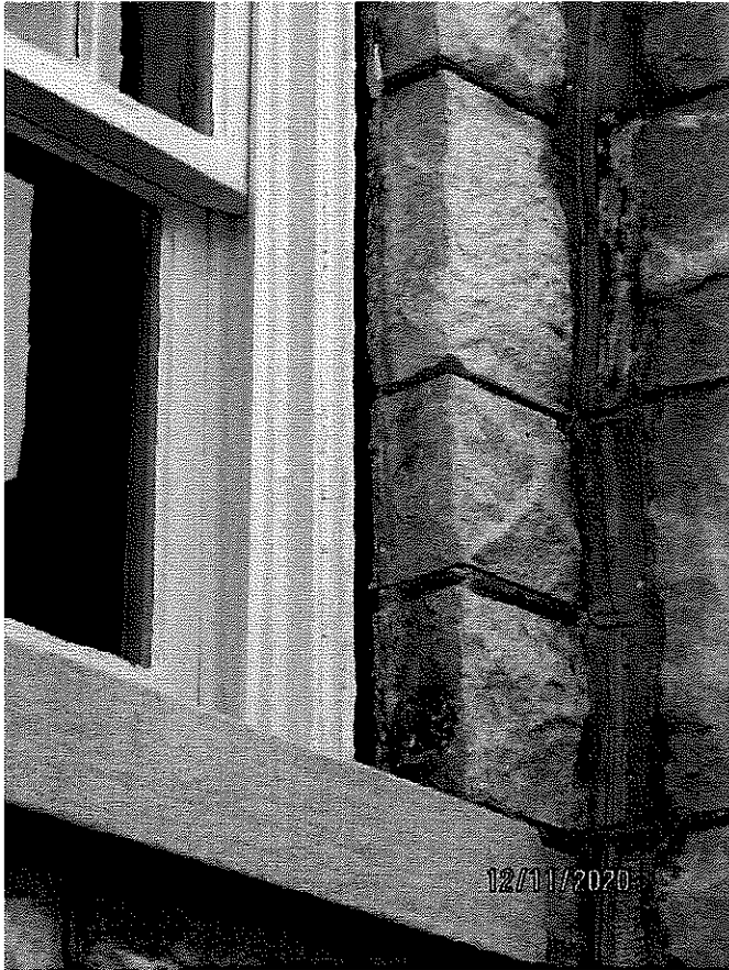
Photograph 7: Wall movement (right side) at window casement.
