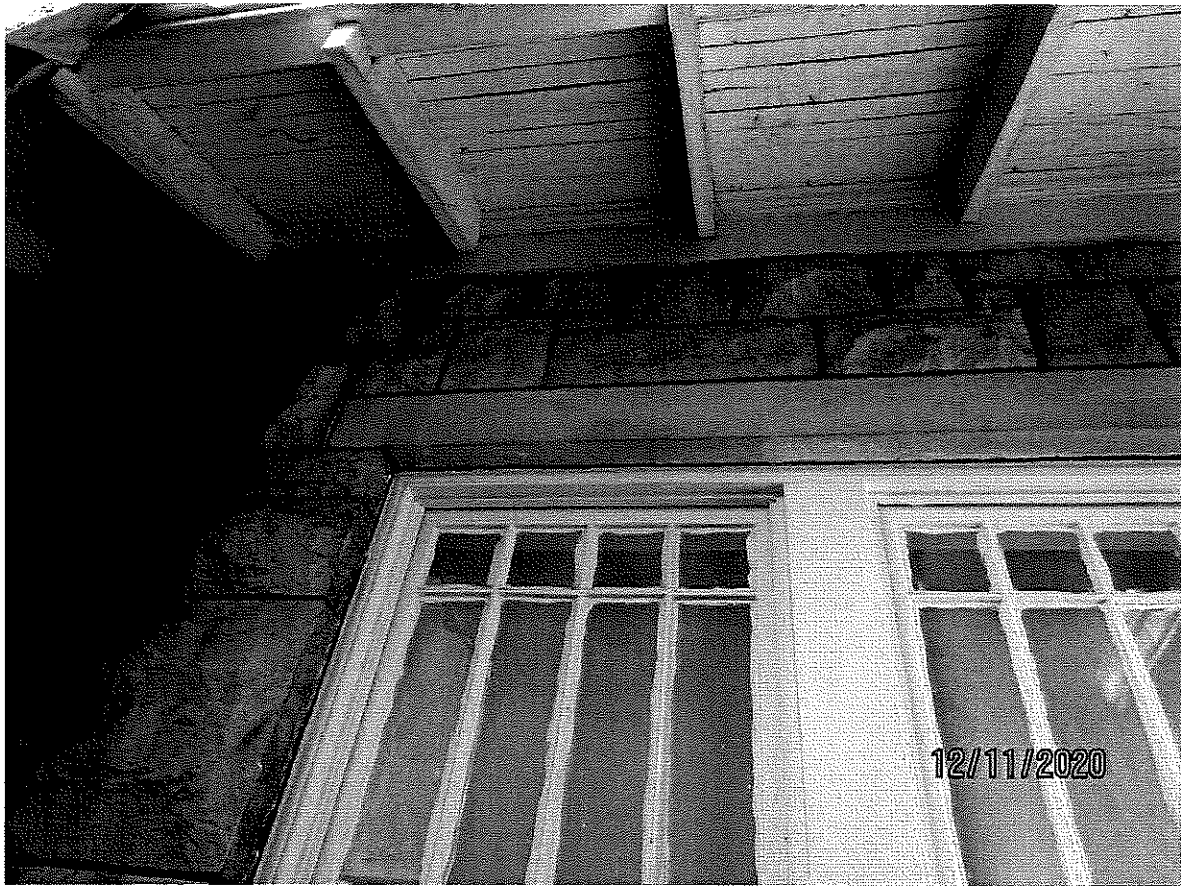
Photograph 25: Wall movement (left side) at window casement.
