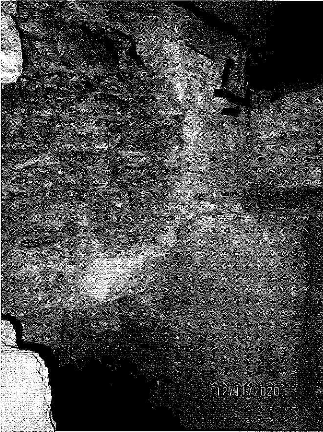
Photograph 33: Typical altered foundation wall.
