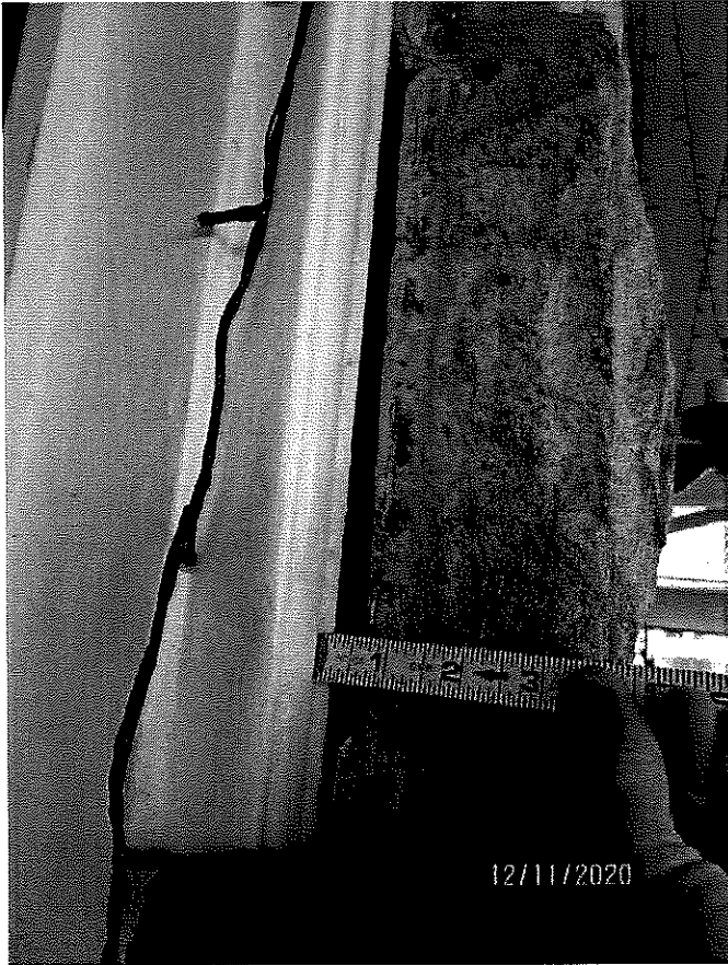
Photograph 3: Wall movement at front wall at doorway.
