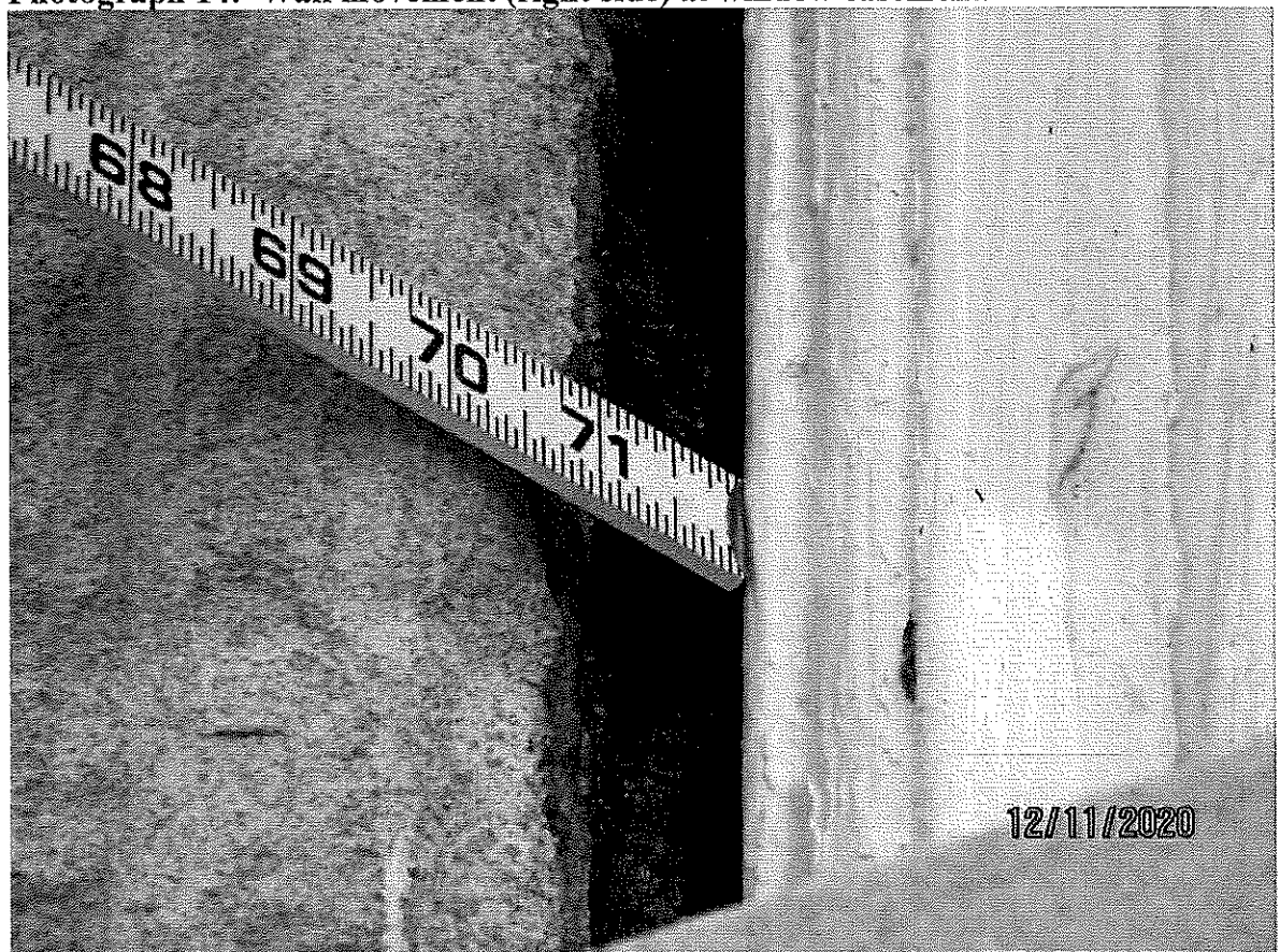
Photograph 14: Wall movement (right side) at window casement.
