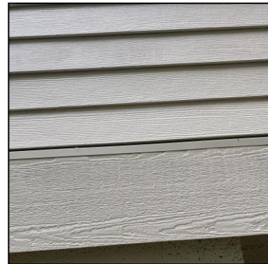
Figure 2: Installed lap siding has a faux grain, specifically called out in the design guidelines as an inappropriate material.
