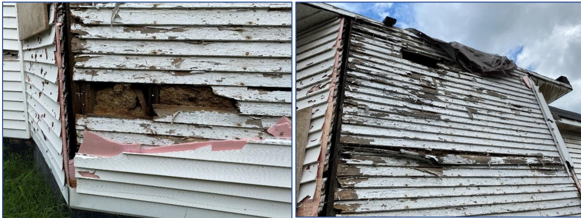
Figures 19 & 20. Some of the exposed historic siding on the left façade is in poor condition.
