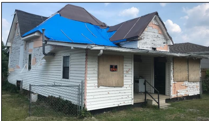
Figure 3. The shed roof portion of the rear of the house will be removed as part of the project.
