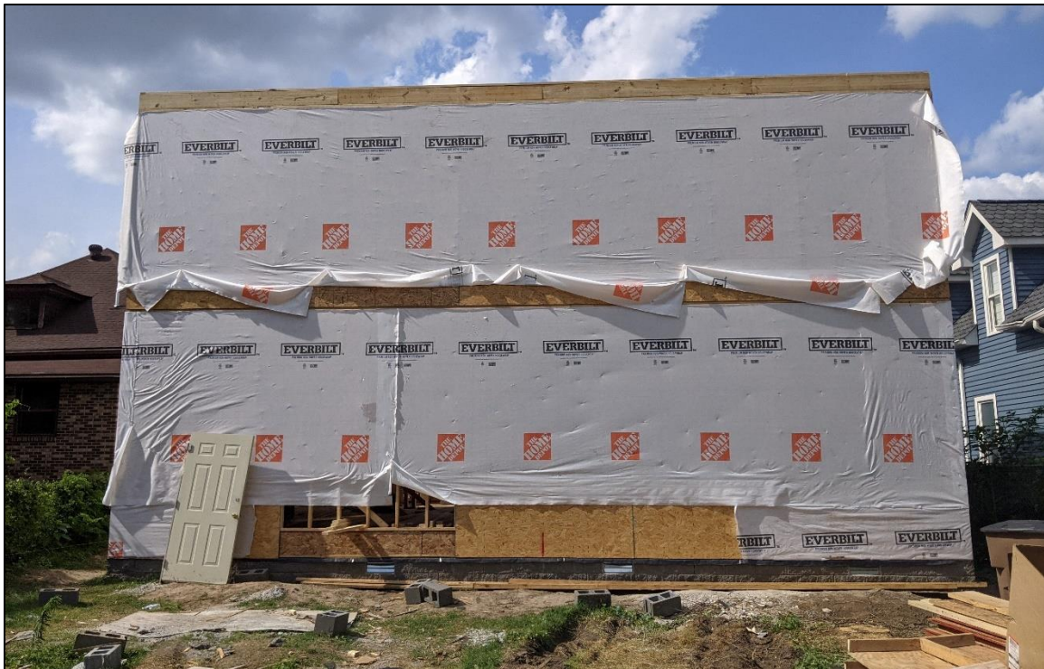
View of the rear wall of the unpermitted addition. (June 24, 2021)
