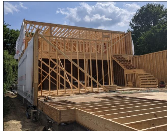
Figure 5: Photo of the unapproved two-story addition, viewed from the rear-left corner of the historic house.
