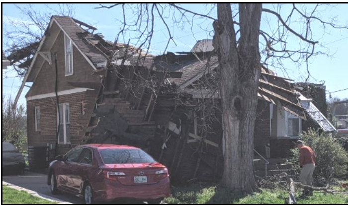
Figure 1. Condition of 1500 Holly Street after the March 2021 storm
