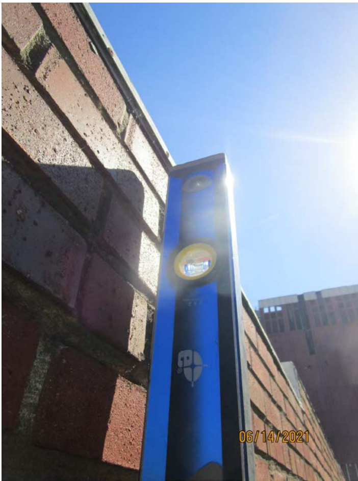
Photograph 93: Out-of-plumb left-side wall of Building 170.
