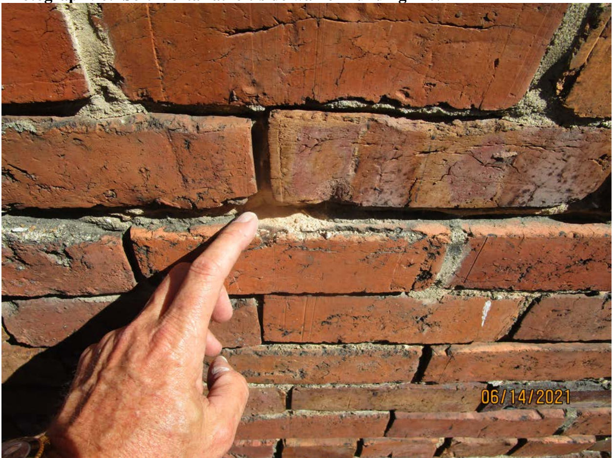
Photograph 96: Soft mortar at left-side wall of Building 170.
