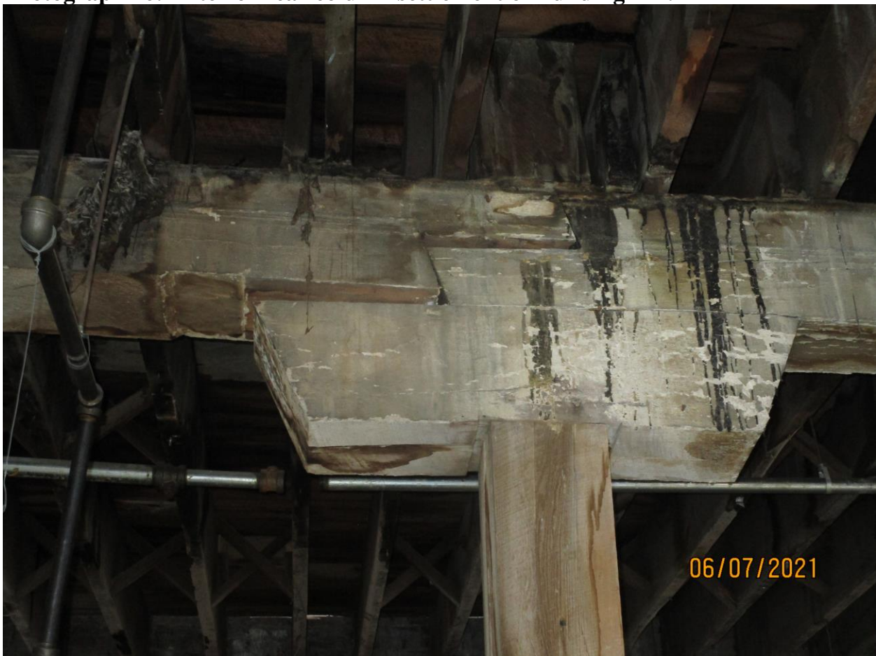
Photograph 26: Interior rear column settlement of Building 174.
