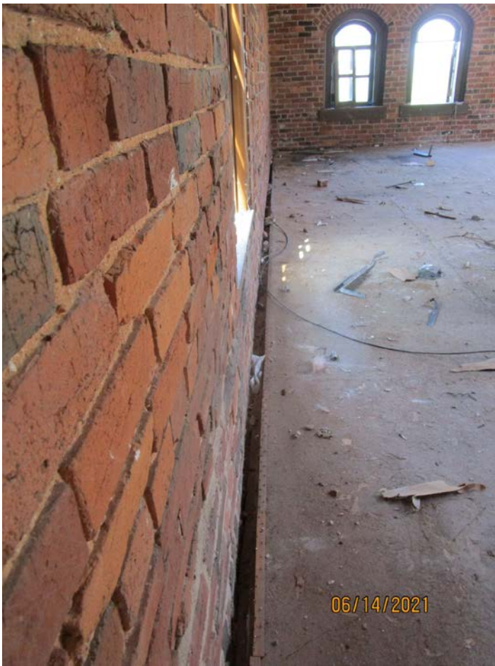
Photograph 75: Third floor left-side wall movement (Building 170).
