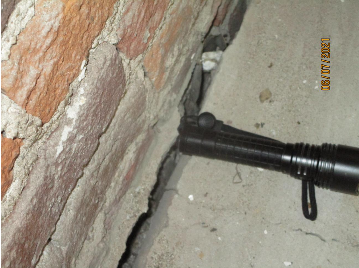
Photograph 58: Rear wall second floor Building 176 (3/4" ± movement since concrete topping).
