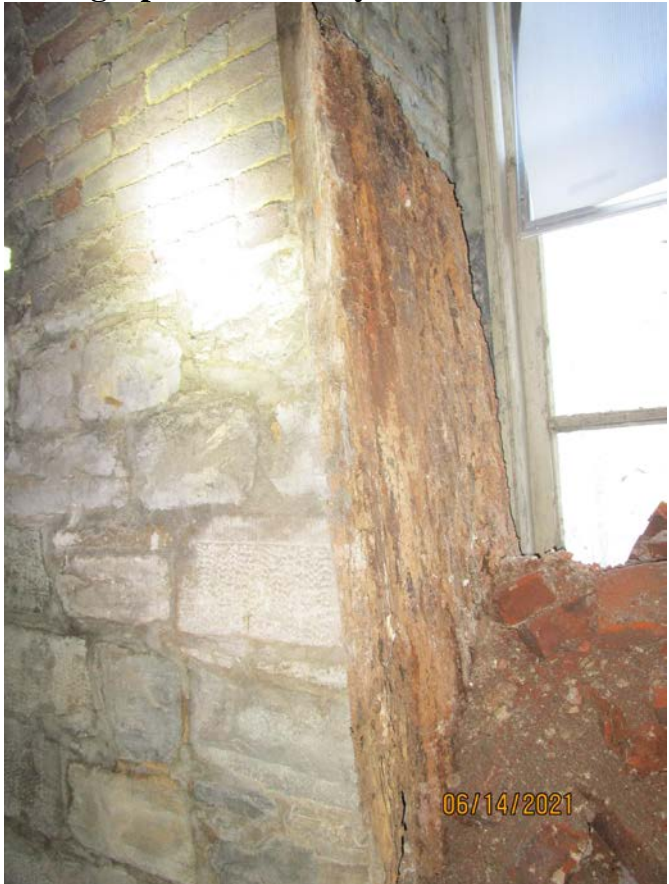
Photograph 90: Recently fallen bricks at Building 176 (EMC photo #53 6/7/2021).
