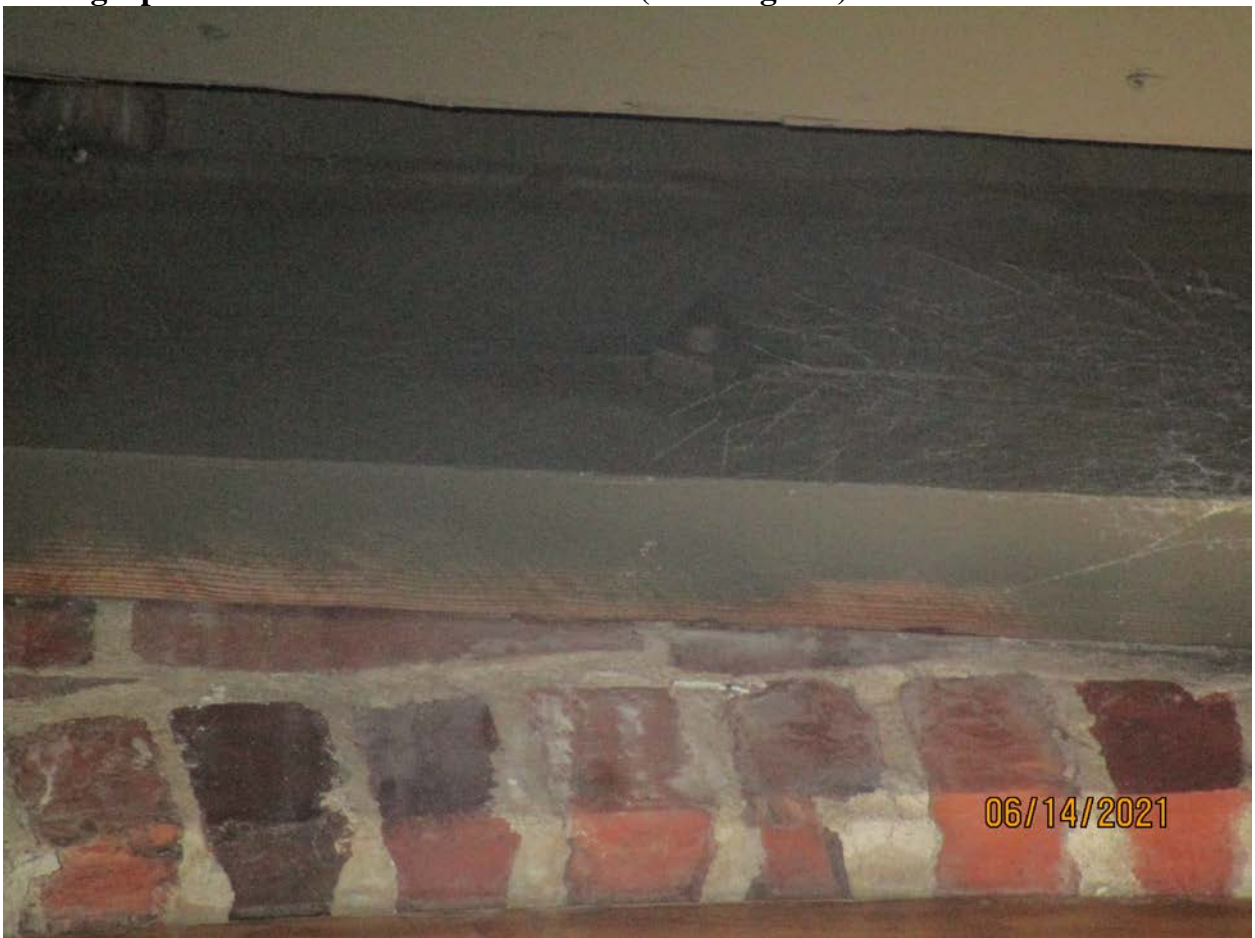
Photograph 50: Rear wall at second floor (Building 170).
