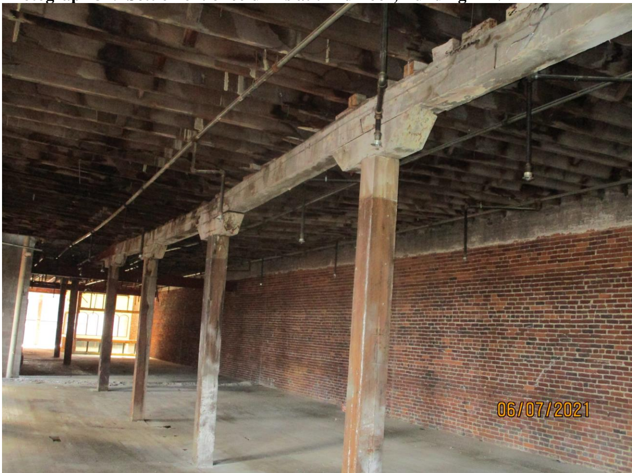
Photograph 34: Settlement of columns at third floor, Building 174.
