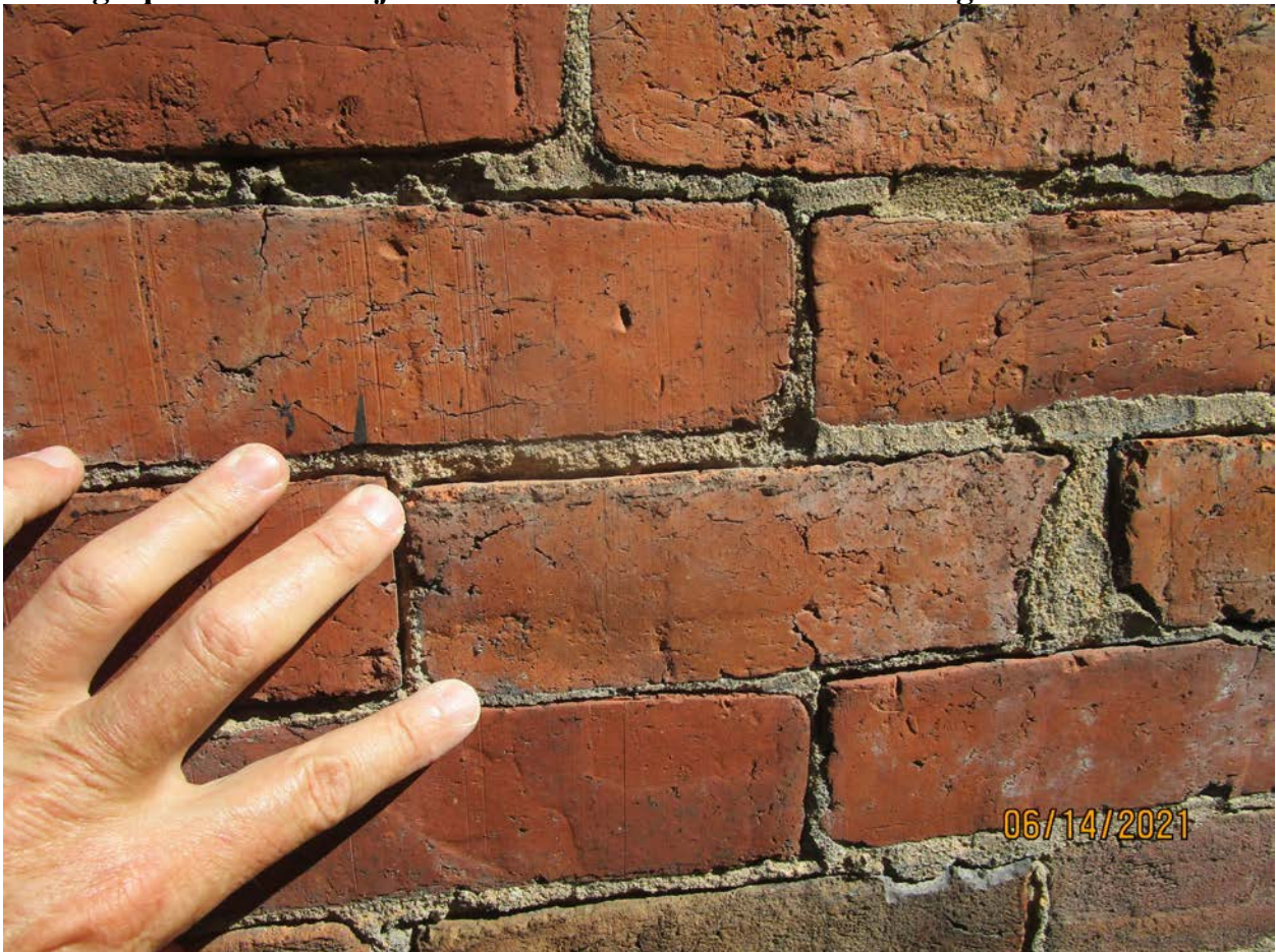
Photograph 98: Mortar joint condition at left-side wall Building 170.
