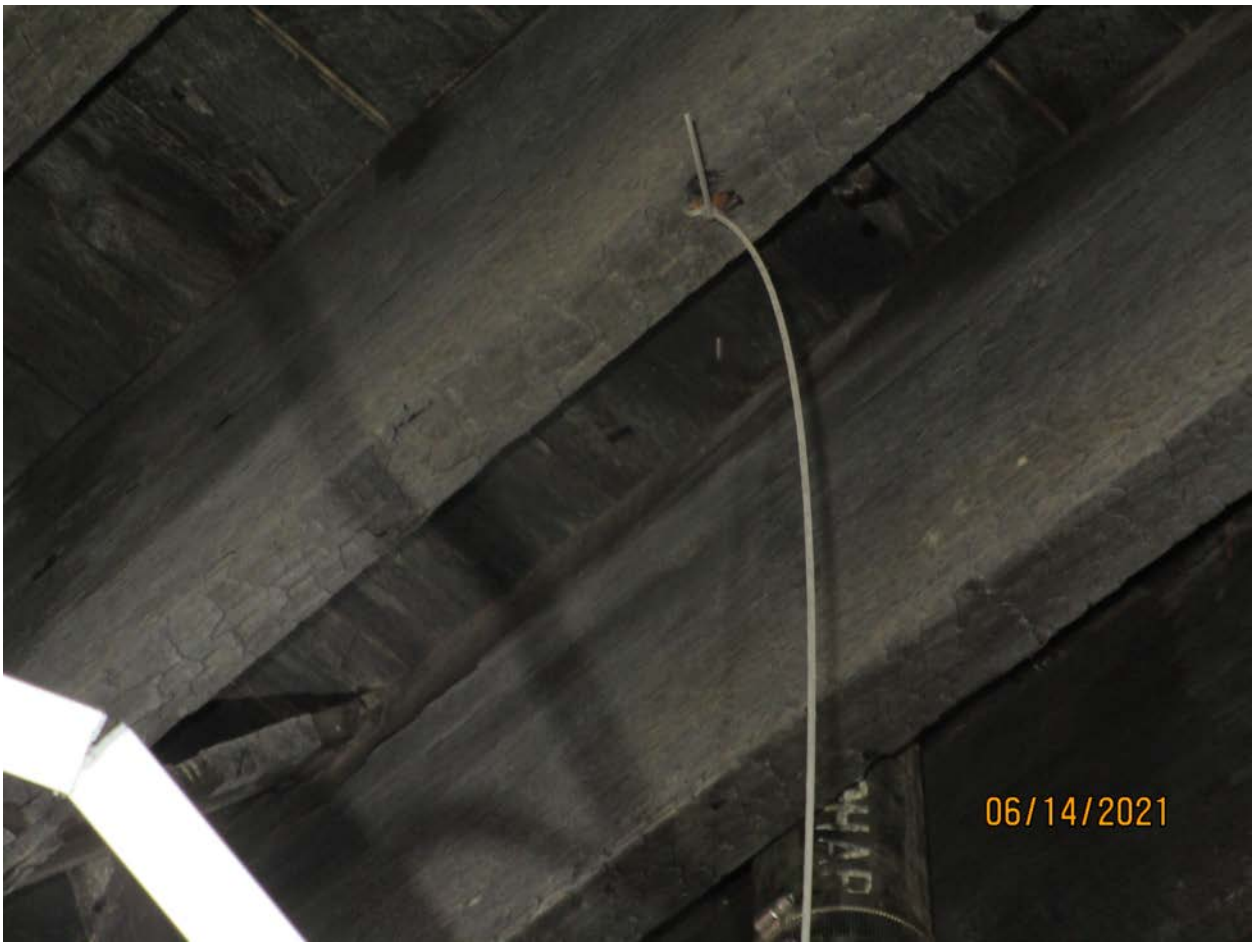
Photograph 15: Fire-damaged wood floor joists at Building 172.
