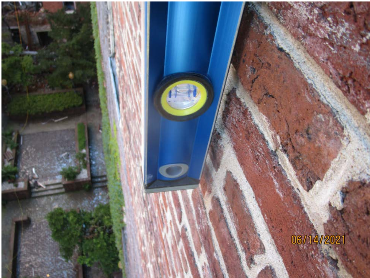
Photograph 105: Near-plumb right-side wall of Building 174.
