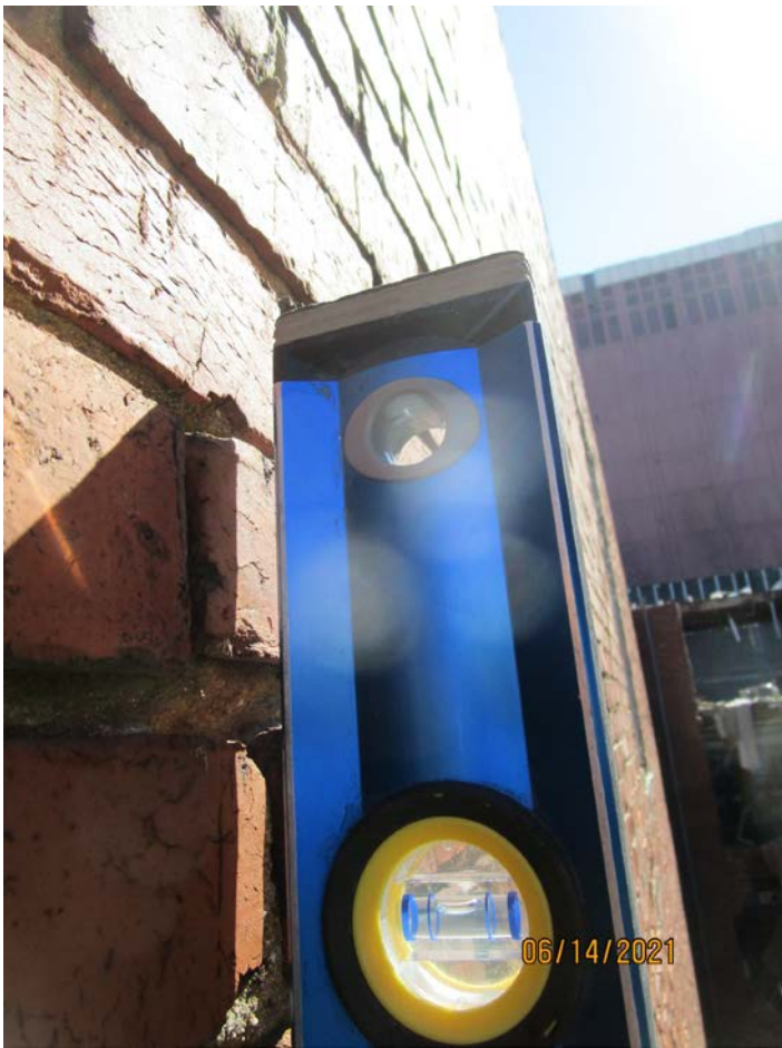
Photograph 95: Out-of-plumb left-side wall of Building 170.
