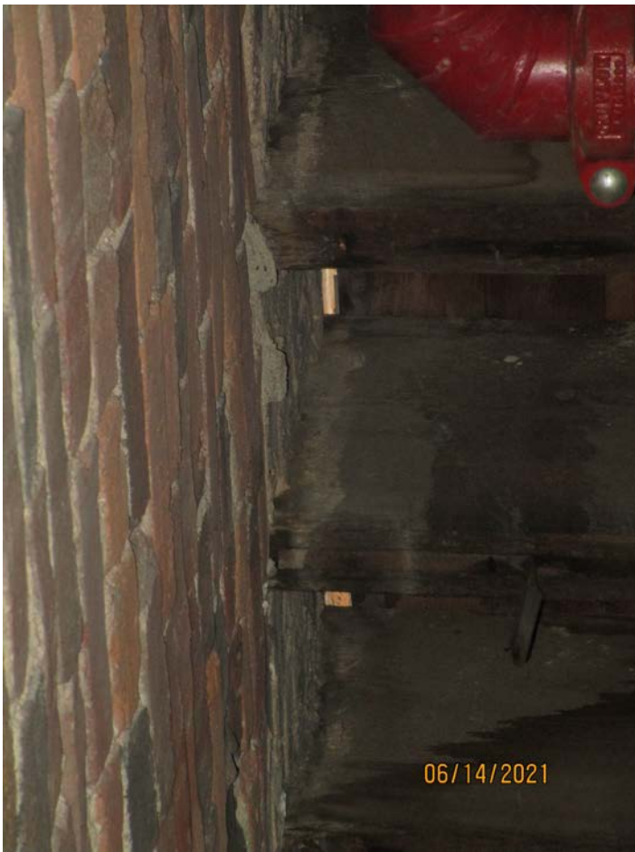
Photograph 35: Second floor joist movement (left wall) of Building 170).
