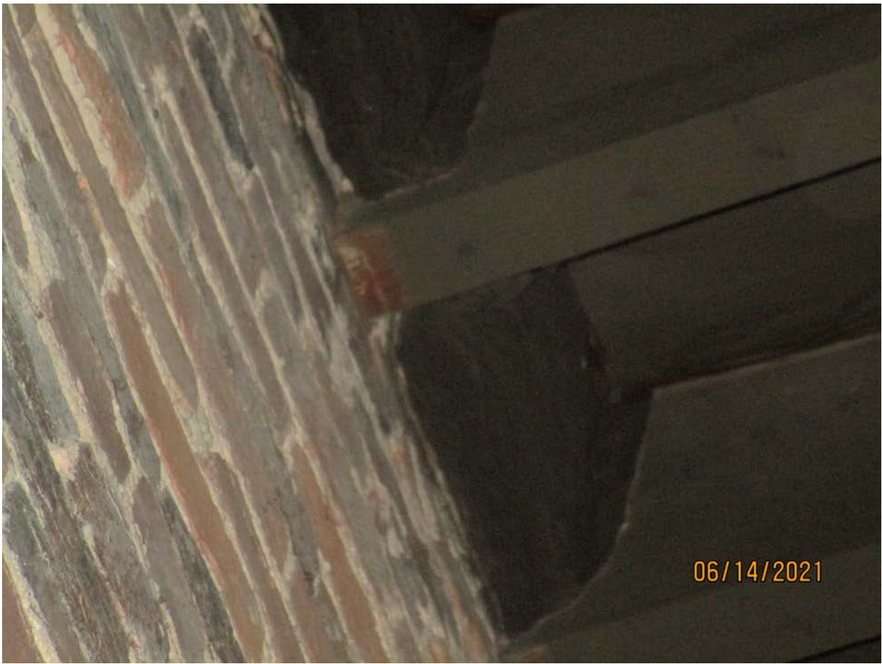
Photograph 43: Second floor left-side wall movement (Building 170).
