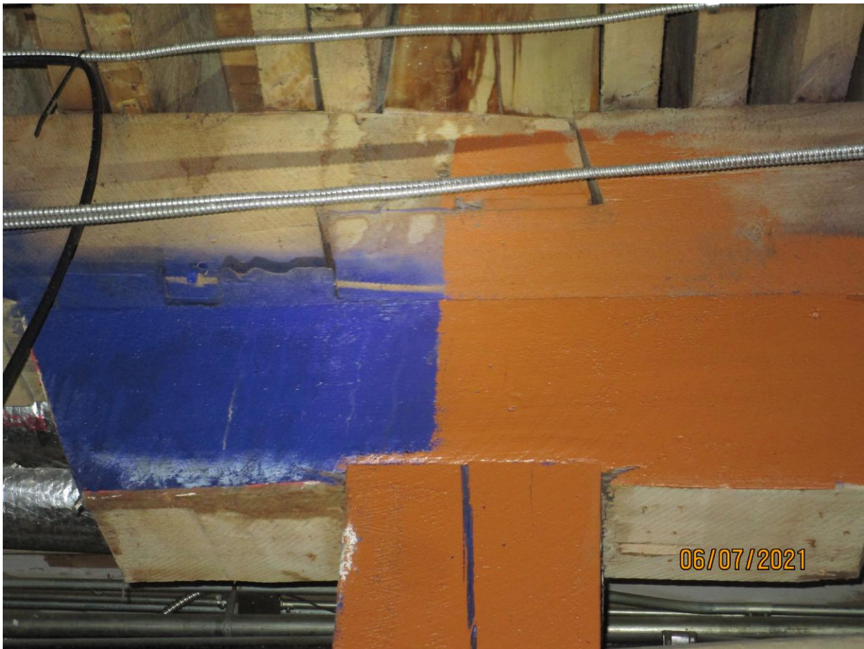
Photograph 51: Broken wood beam in basement/settlement Building 174.
