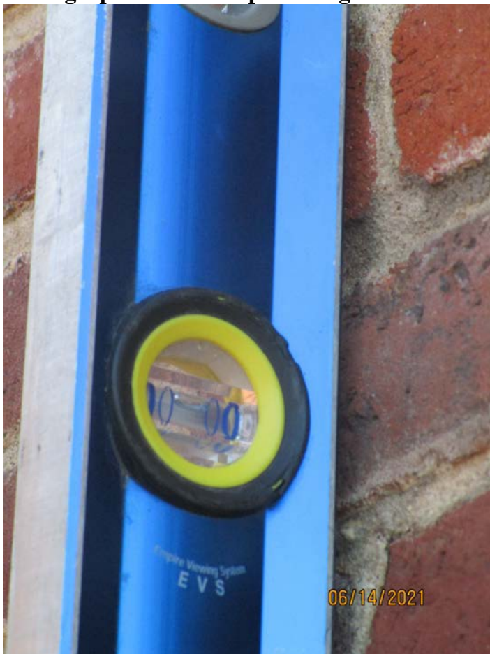
Photograph 106: Near-plumb right-side wall of Building 174.
