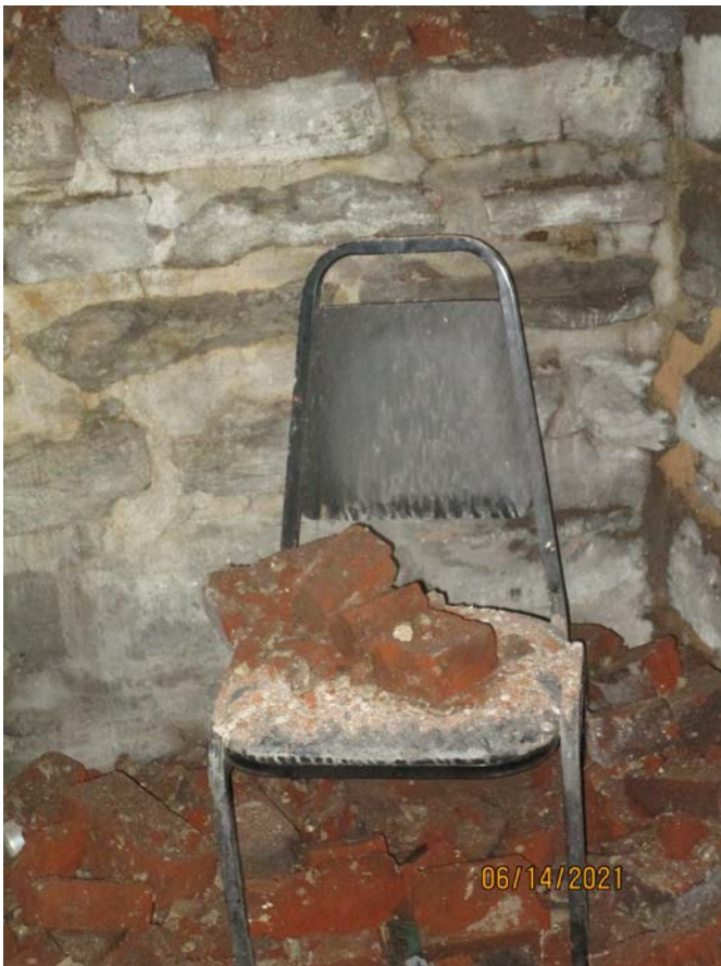
Photograph 87: Recently fallen bricks at Building 176 (EMC photo #53 6/7/2021).
