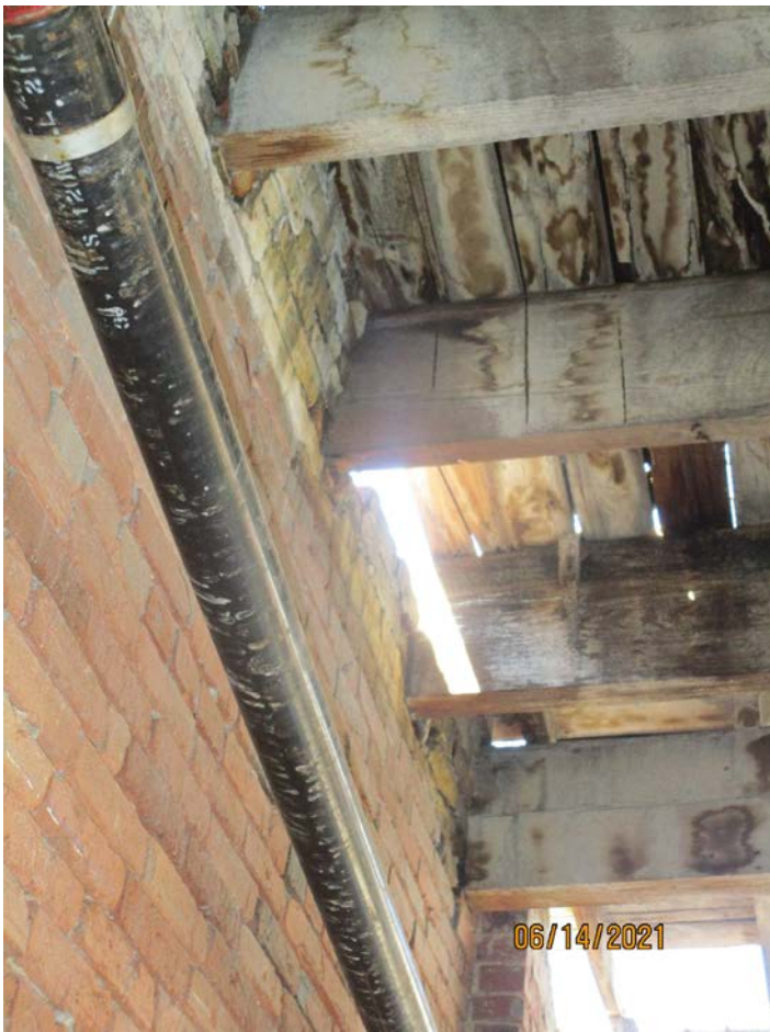
Photograph 83: Roof joist movement at Building 172.
