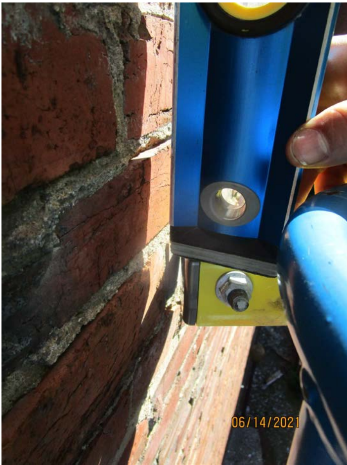
Photograph 97: Out-of-plumb left-side wall of Building 170.
