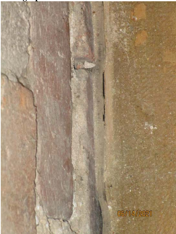
Photograph 42: First floor movement at left-side wall (Building 170).
