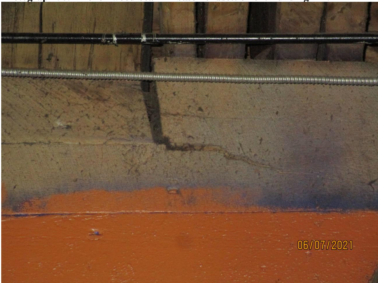
Photograph 50: Broken wood beam in basement/settlement Building 174.
