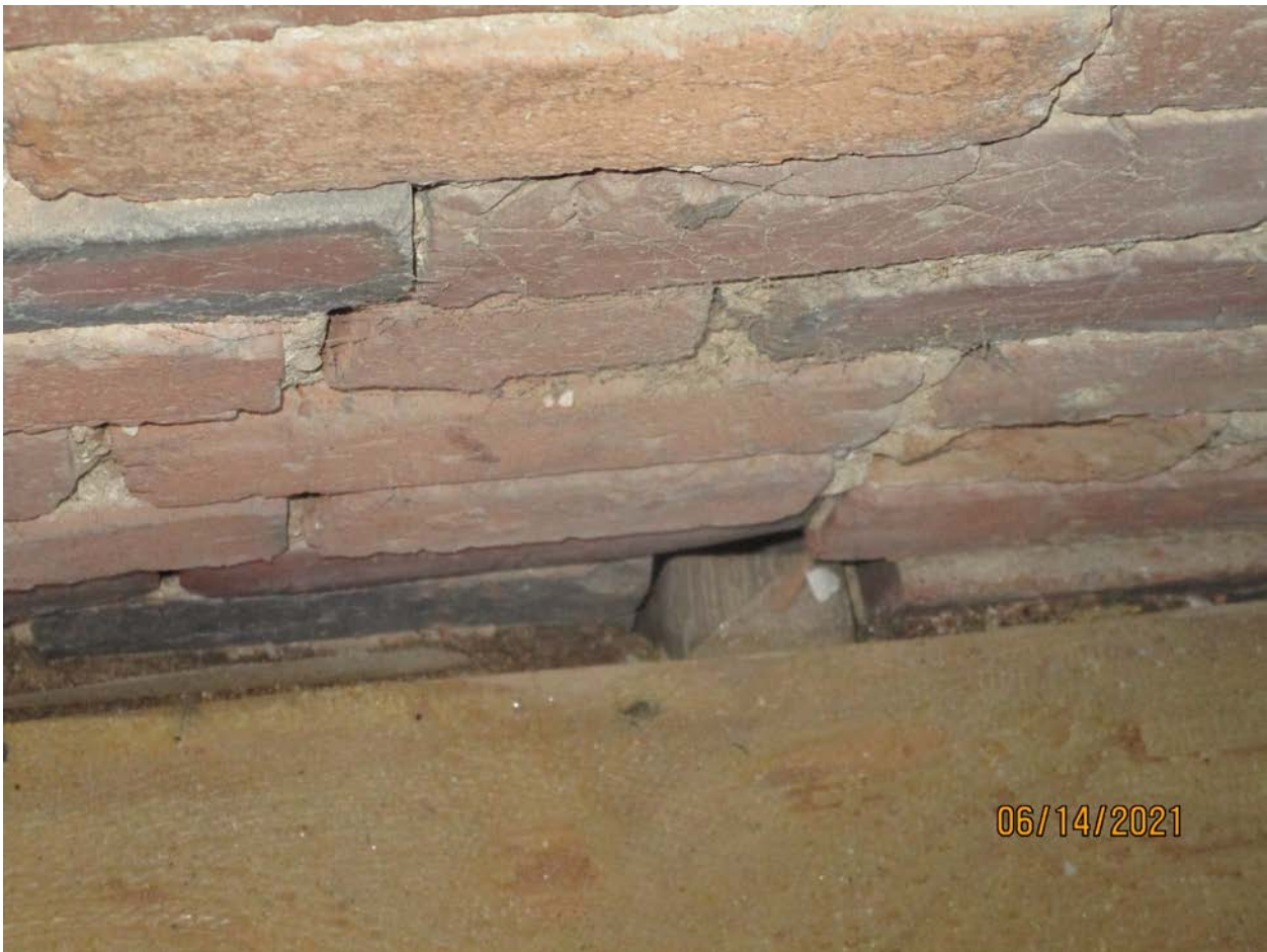
Photograph 67: Floor joist movement at second floor (Building 170).
