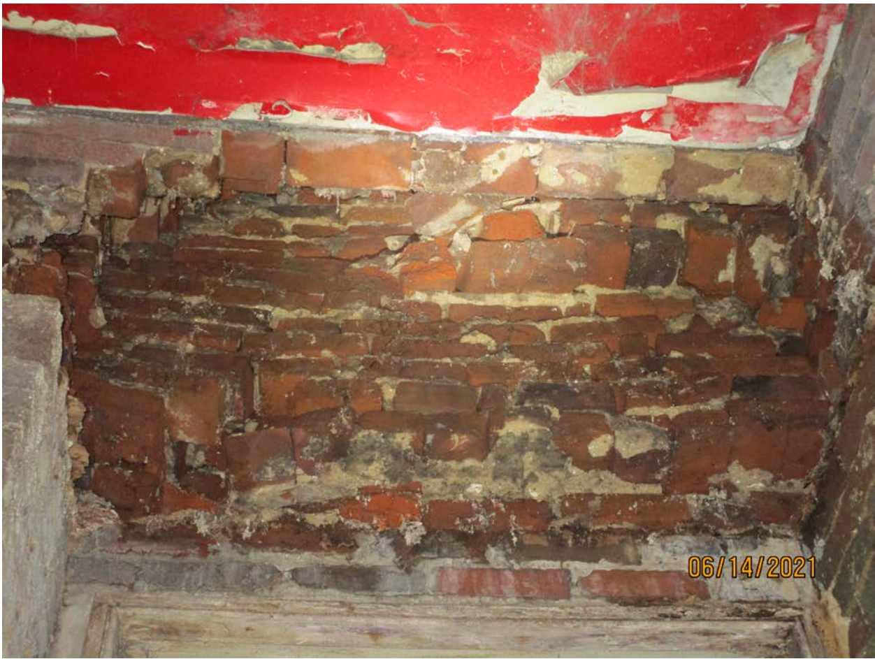
Photograph 89: Recently fallen bricks at Building 176 (EMC photo #53 6/7/2021).
