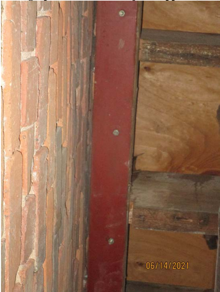
Photograph 64: Third floor joist support (left-side wall) at Building 170).
