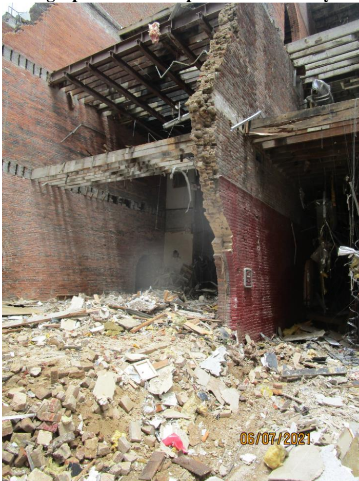
Photograph 12: Close-up of failed masonry arch at Buildings 170/172.
