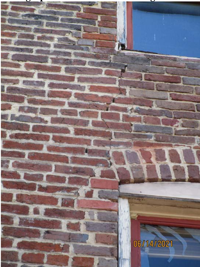
Photograph 100: Brick cracks at right-side wall of Building 174.
