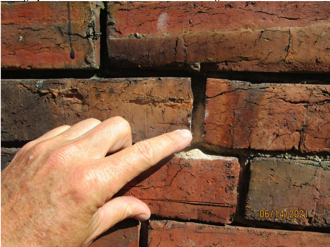
Photograph 94: Soft mortar at left-side wall of Building 170.
