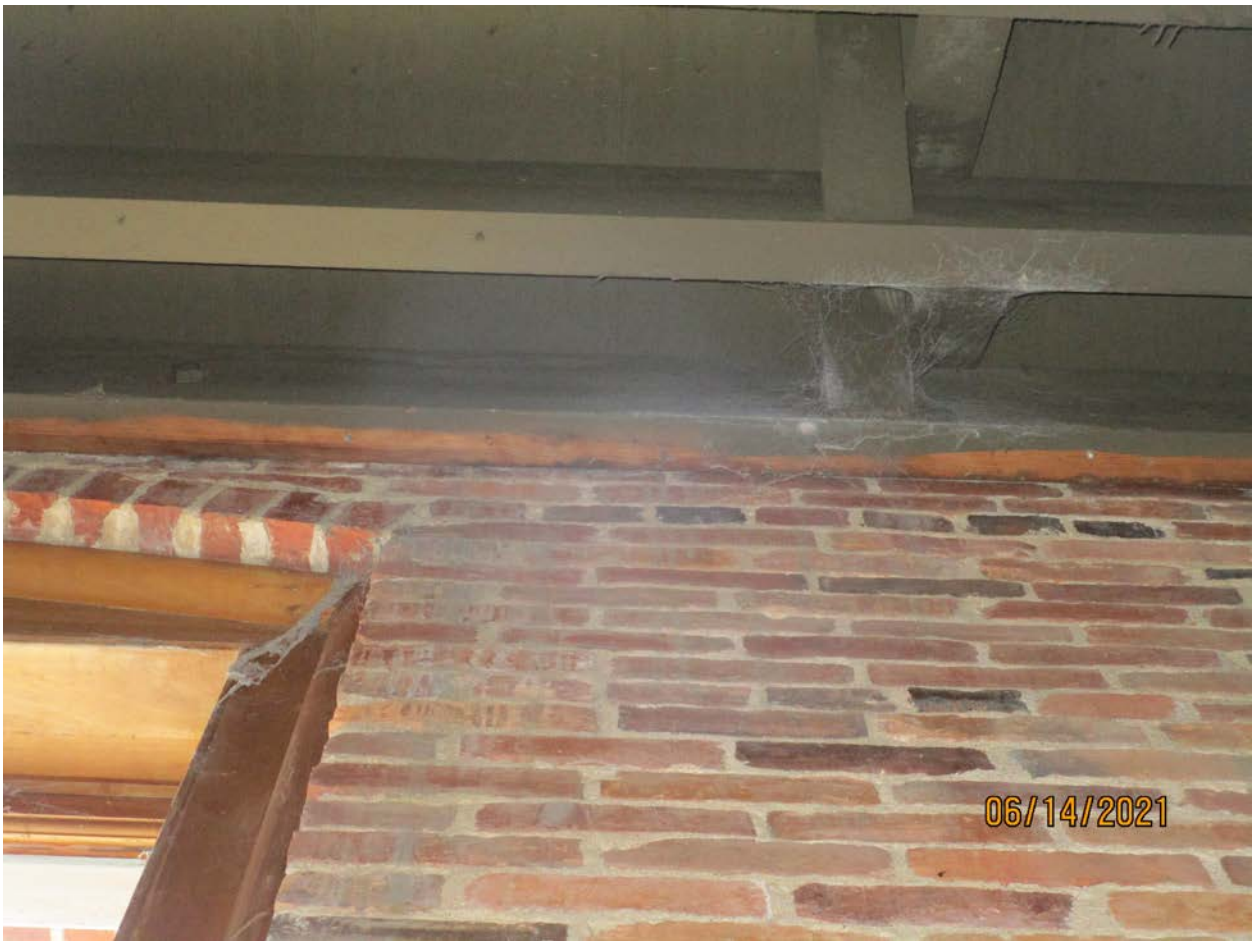
Photograph 49: Rear wall at second floor (Building 170).
