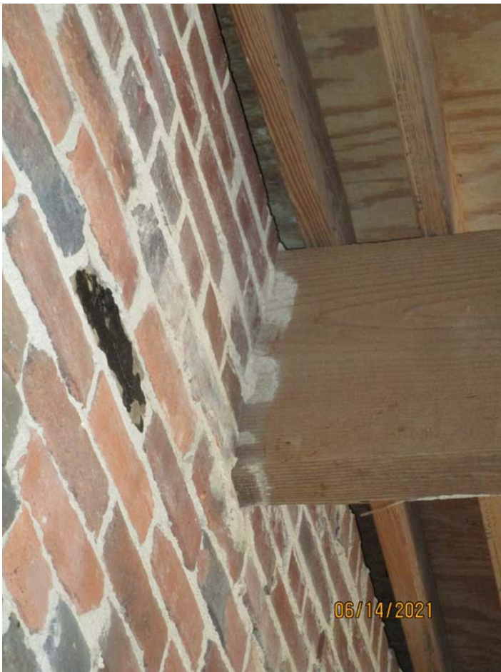
Photograph 73: Roof rafter movement at left-side wall (Building 170).
