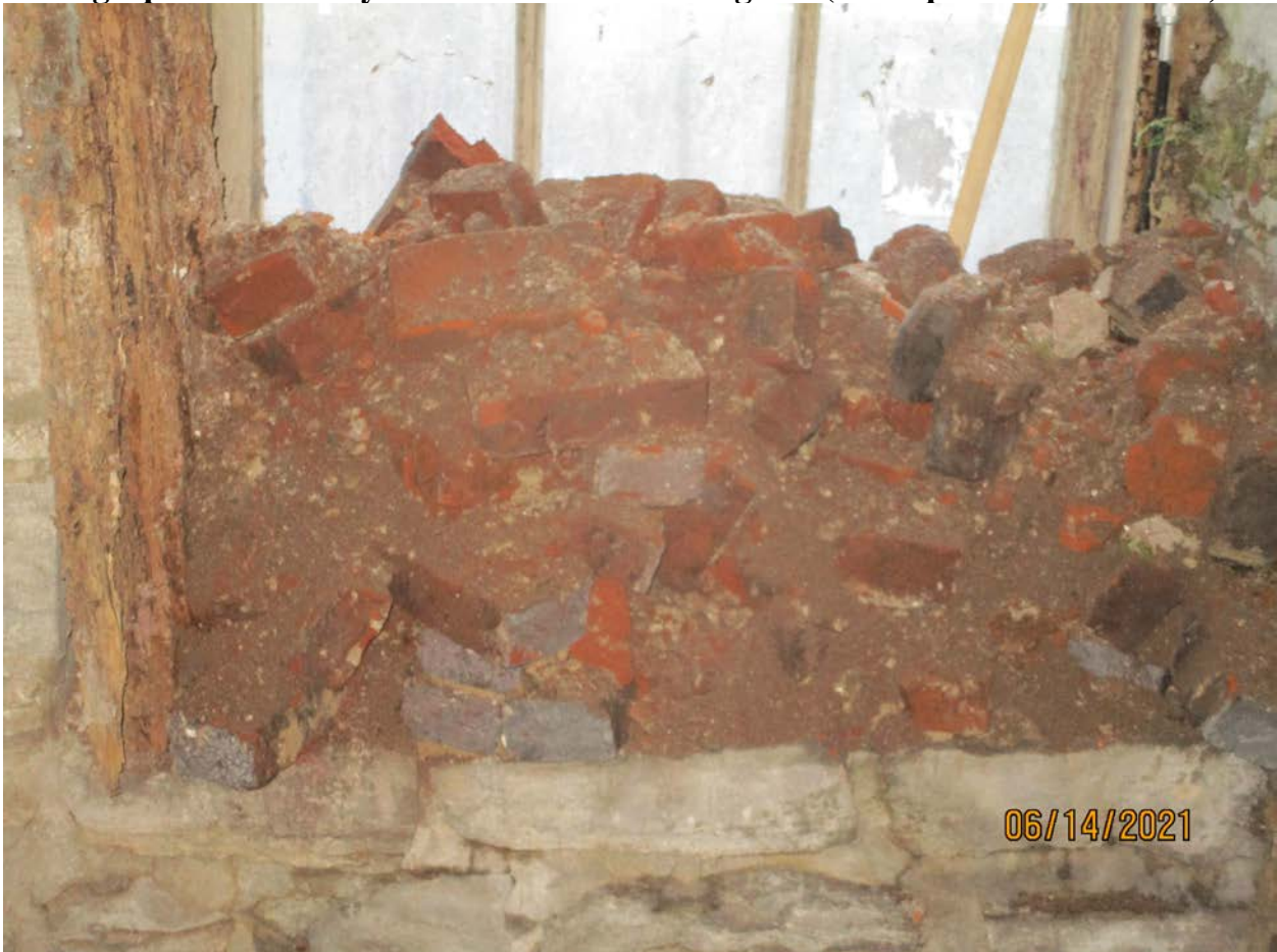
Photograph 88: Recently fallen bricks at Building 176 (EMC photo #53 6/7/2021).
