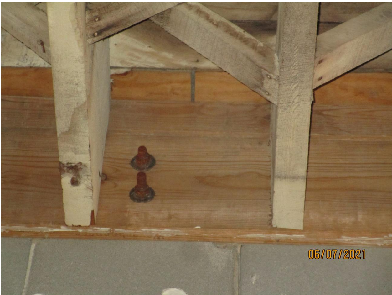
Photograph 65: Bolted ledger board at right-side wall of third floor, Building 176.
