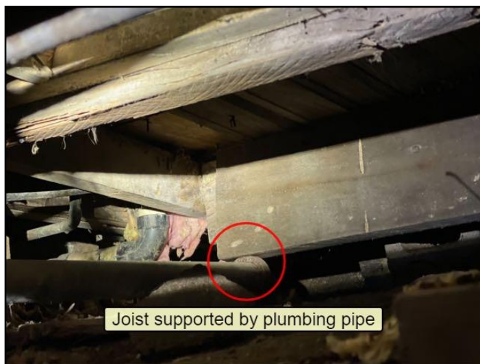
71. Improper joist support
