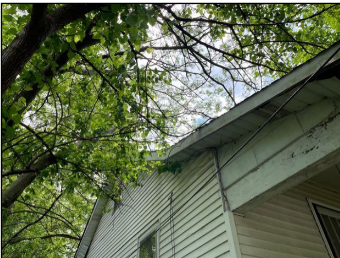
31. Trees or shrubs too close to building
