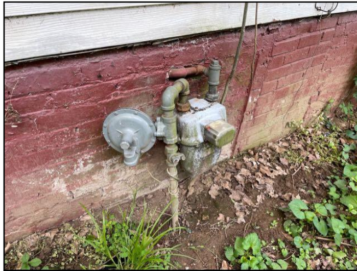
92. The gas was shut off at the meter. This...
