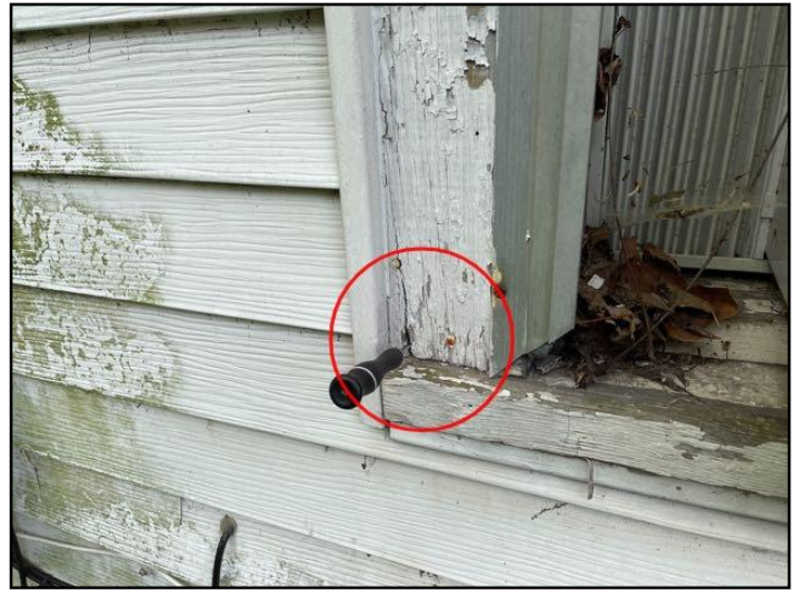
12. Rot in window trim
