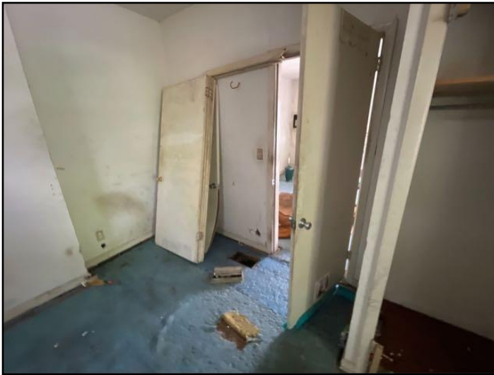
131. Doors not installed
