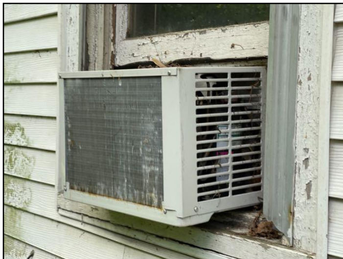
98. Window cooling system
