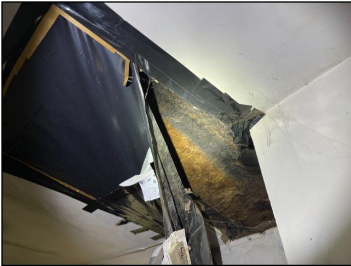
119. Hole in ceiling (moisture in roof sheathing)
