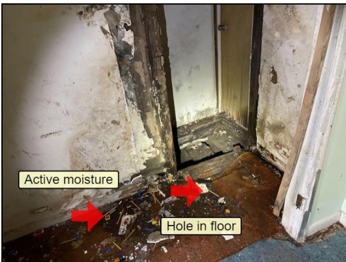
125. Hole in floor
