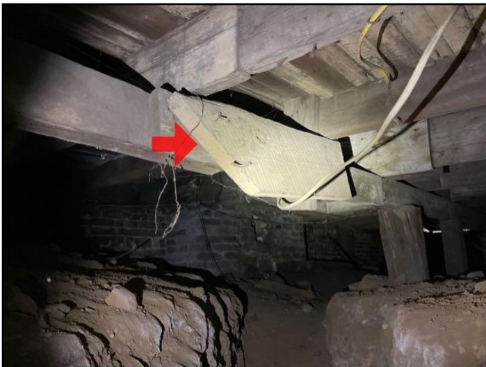
67. Improperly spliced beam
