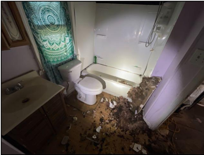
123. Wet insulation in bathroom from active leak
