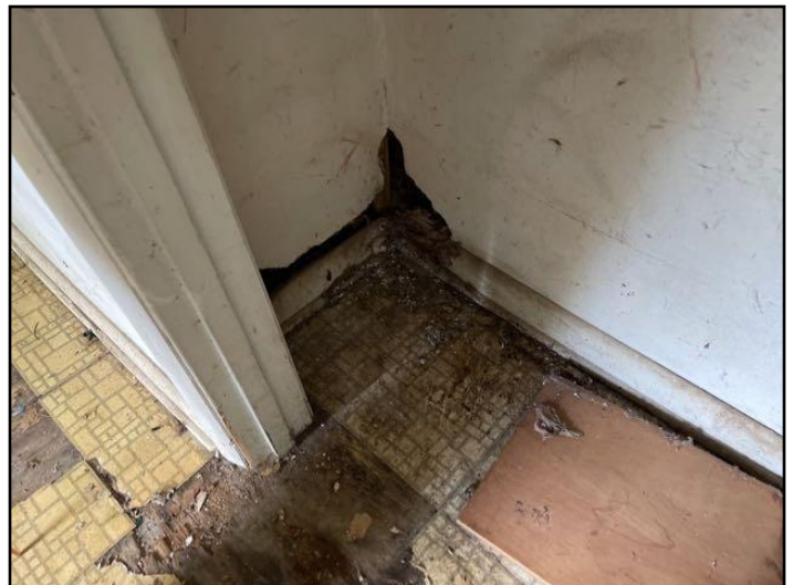
122. Damage to wall
