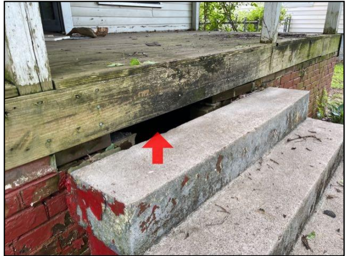
44. Hole in foundation wall
