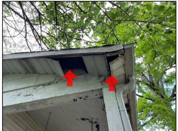
10. Soffit and fascia damaged or missing
