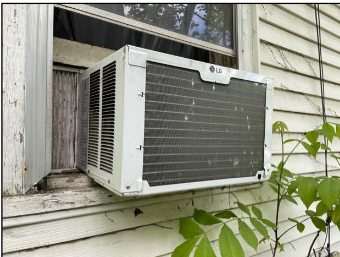
97. Window cooling system
