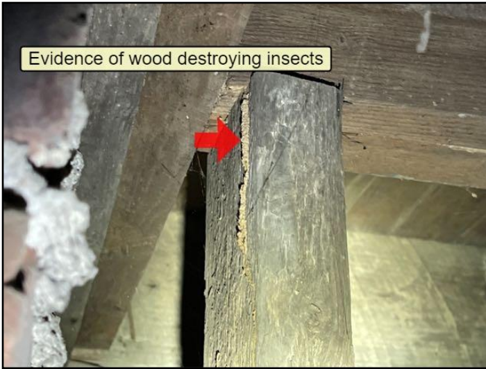
61. Evidence of wood destroying insects
