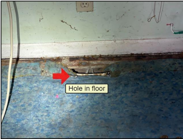
127. Hole in floor
