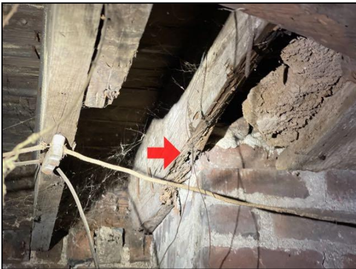
69. Excessive insect damage
