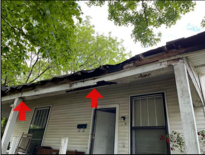
7. Heavy rot and deterioration
