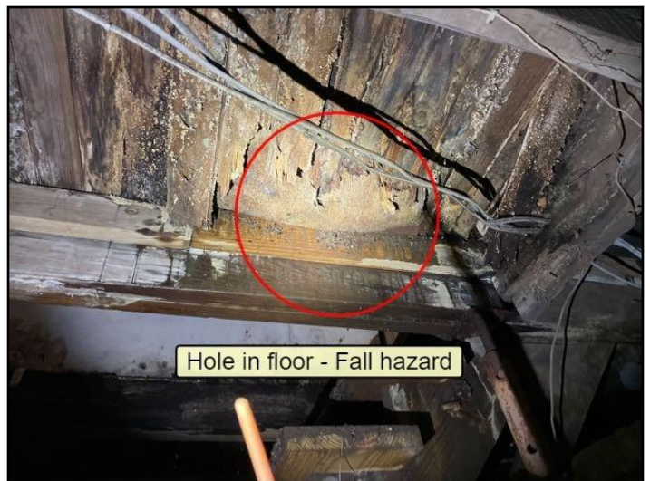
48. Hole in floor sheathing from rot
