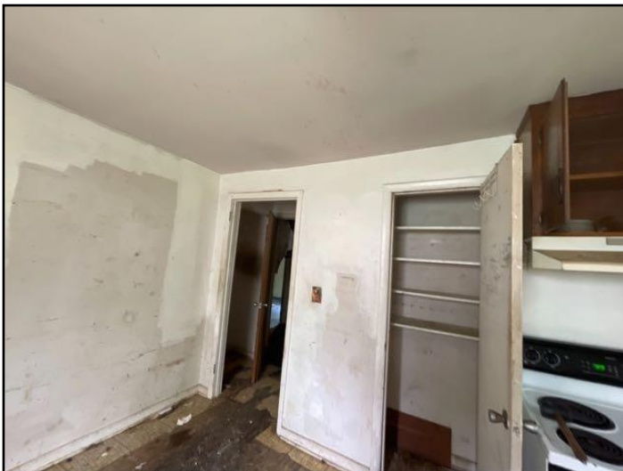
121. General poor condition
