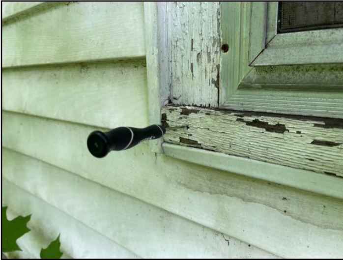
15. Rot in window trim
