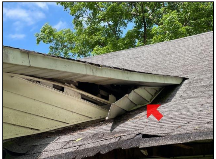
18. Vinyl siding falling off home
