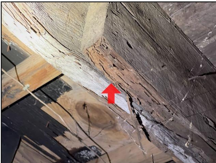
59. Extensive insect damage
