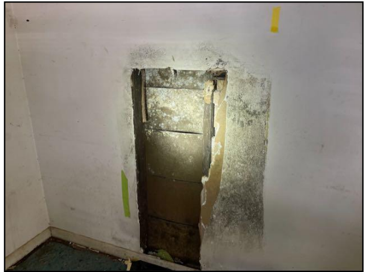
128. Damage to wall
