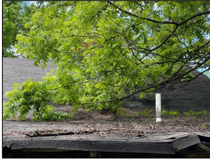
33. Trees or shrubs too close to building
