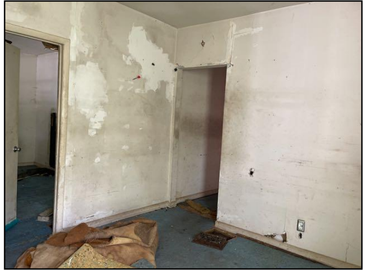
108. Generally poor condition
