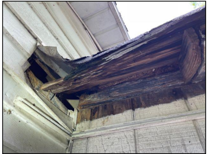
73. Rafter tails and sheathing deteriorated
