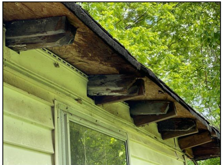
79. Active moisture on rafter tails and sheathing
