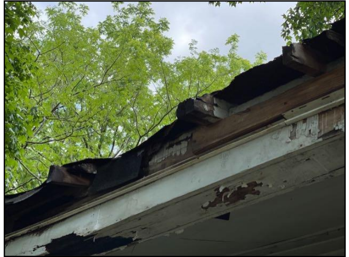
77. Deteriorated sheathing and rafter tails
