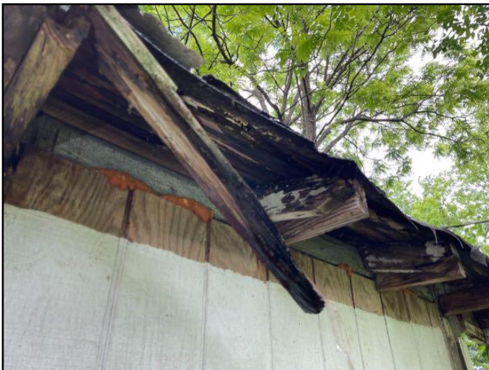
74. Rafter tails and sheathing deteriorated
