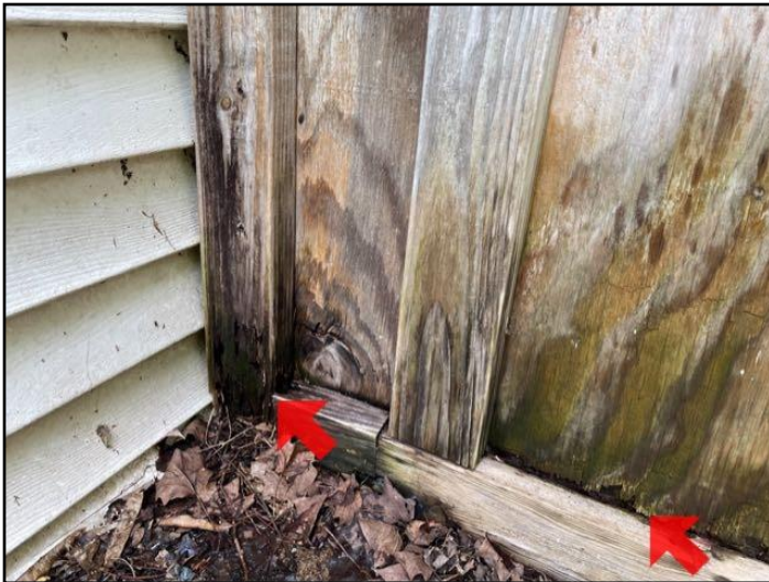
19. Heavy deterioration in wood siding
