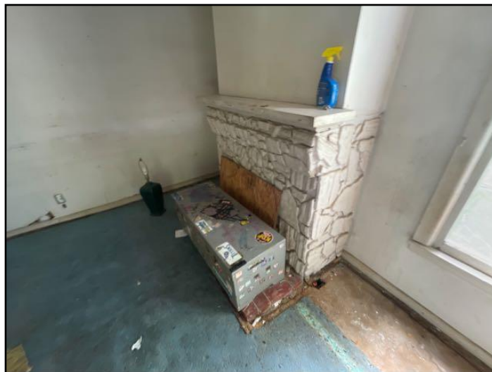
93. Storage preventing inspection
