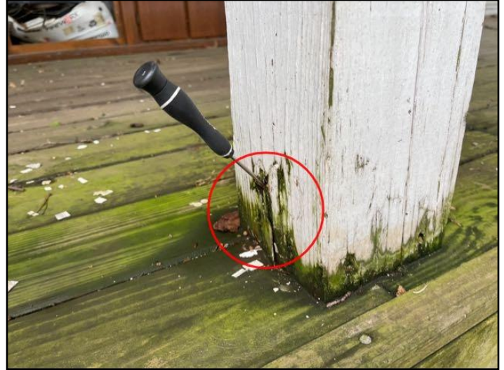
8. Rot in front porch posts
