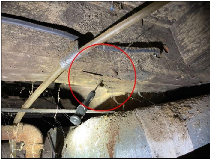
57. Rot in built-up beam
