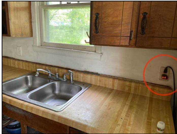
89. No GFCI/GFI (Ground Fault Circuit...
