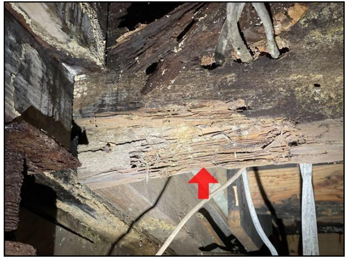
46. Extensive insect damage in floor framing
