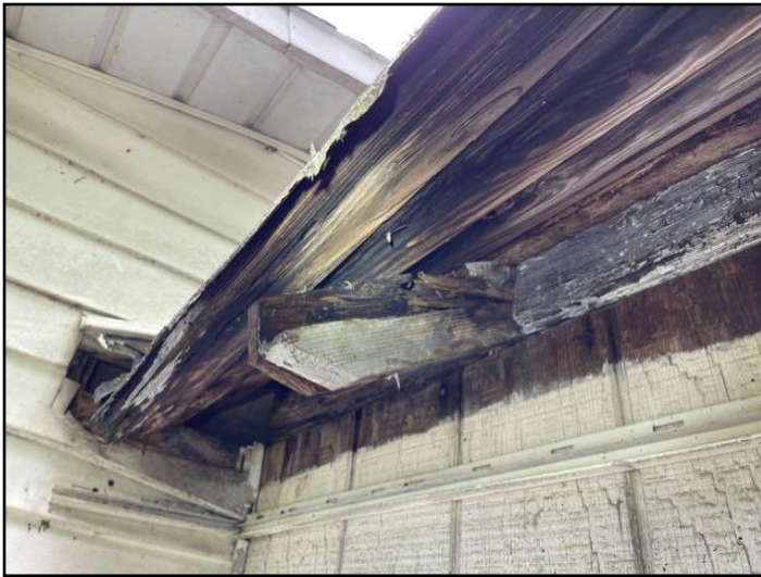
72. Rafter tails and sheathing deteriorated
