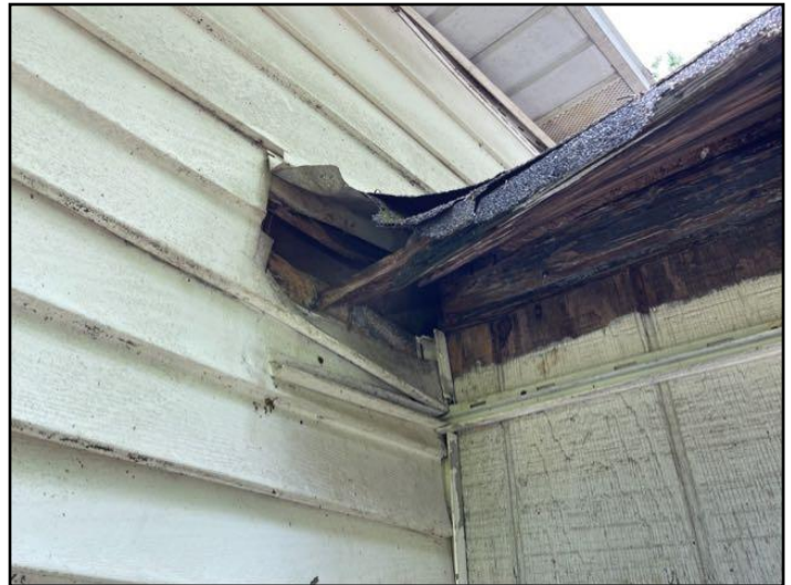
20. Holes in siding
