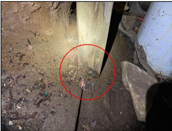
51. Column in contact with dirt
