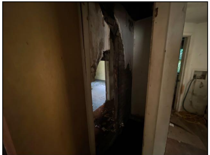
118. Hole through wall framing
