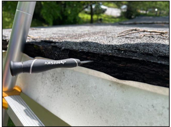
81. Rot in sheathing
