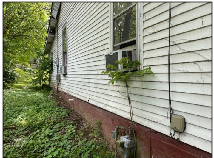
32. Trees or shrubs too close to building
