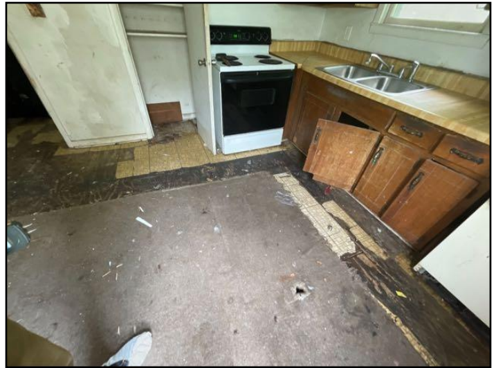
120. General poor condition
