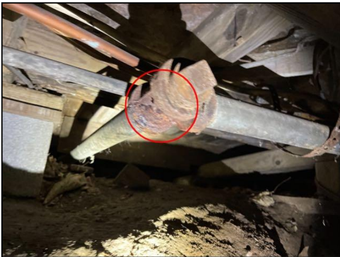
105. rust on cast iron
