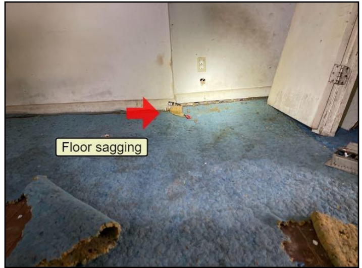
132. Floor system sagging
