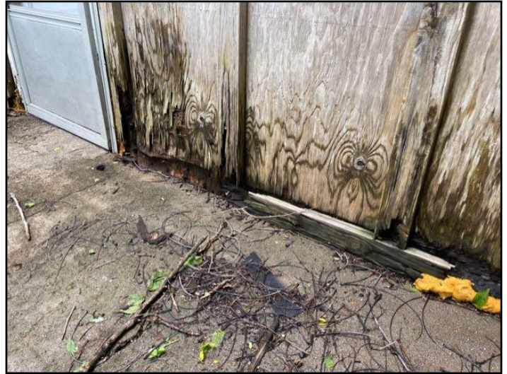
16. Heavy deterioration in wood siding
