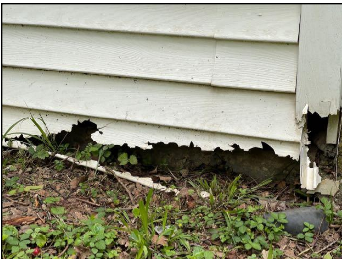
21. Damaged vinyl siding
