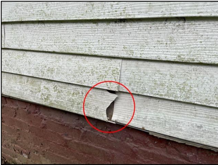
11. Vinyl siding damaged
