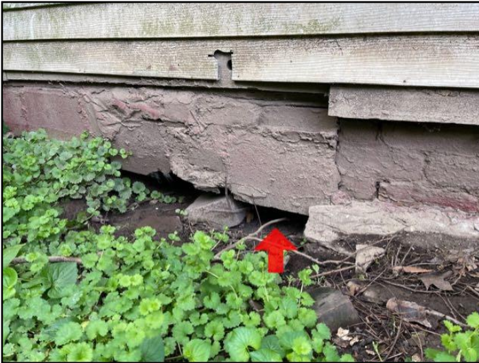
43. unsupported foundation wall
