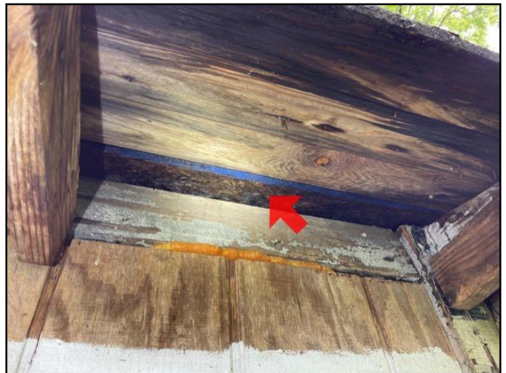
75. Active moisture in sheathing
