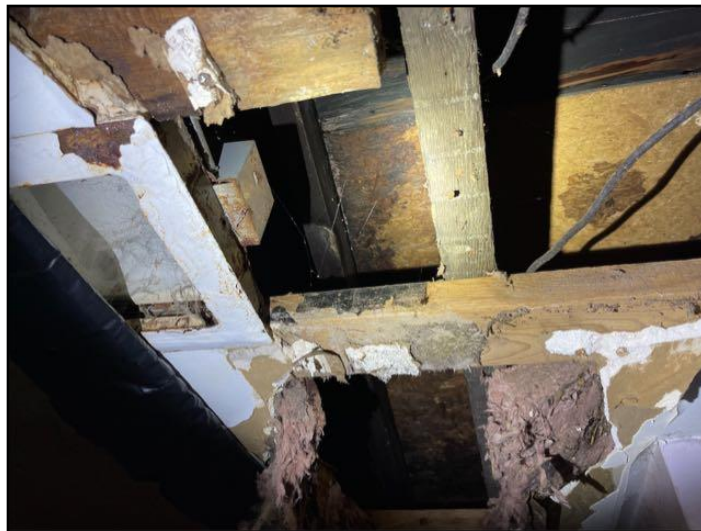
82. Active moisture in sheathing - inside home
