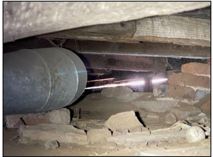
66. light visible through foundation wall
