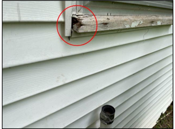
24. Rot in window trim
