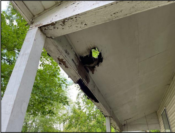
76. Hole through roof
