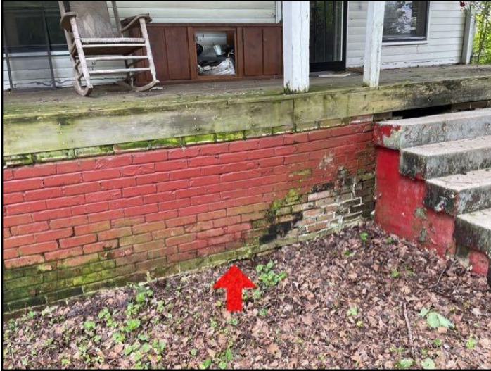
41. Movement in foundation wall
