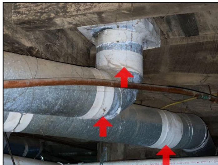
101. Possible asbestos material
