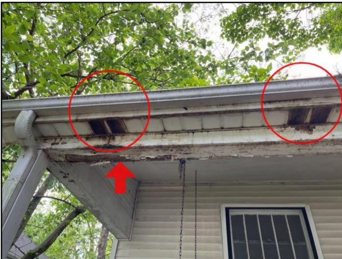
9. Rot and damage to soffit/fascia
