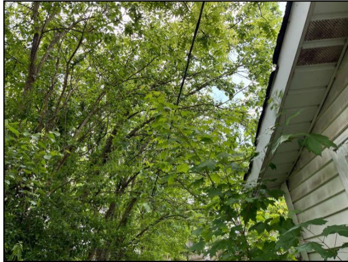
83. Branches / vines interfering with wires
