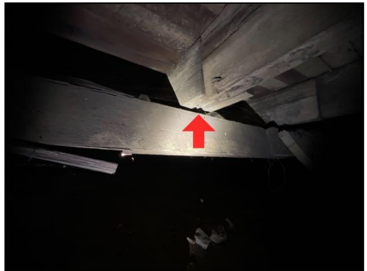
68. Beam not contacting joists
