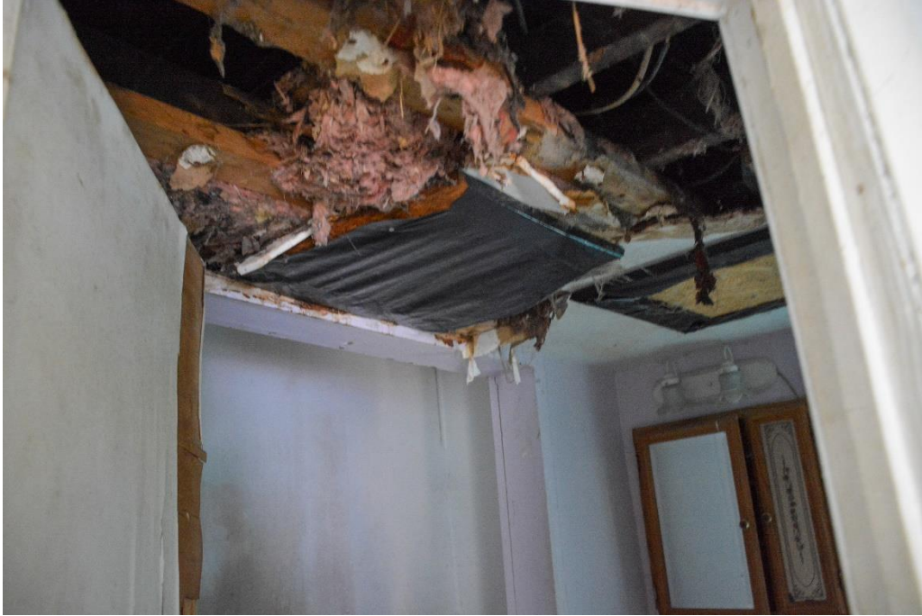
Photo 3: Interior Ceiling Condition
