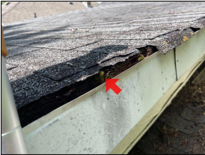
80. Rot in sheathing
