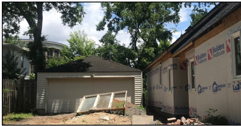
Figure 2. Garage with addition under construction. Separation measures twenty-seven and a half inches (27.5")
