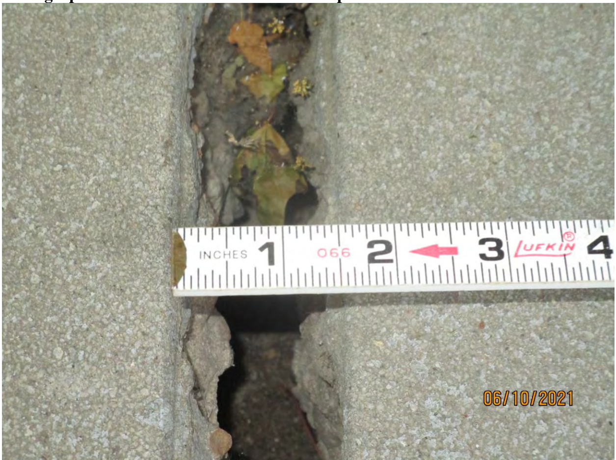
Photograph 6: Horizontal movement of front porch.
