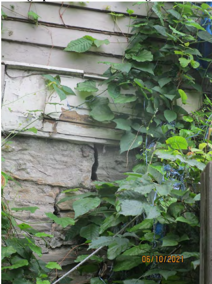
Photograph 20: Settlement of right rear corner foundation wall.
