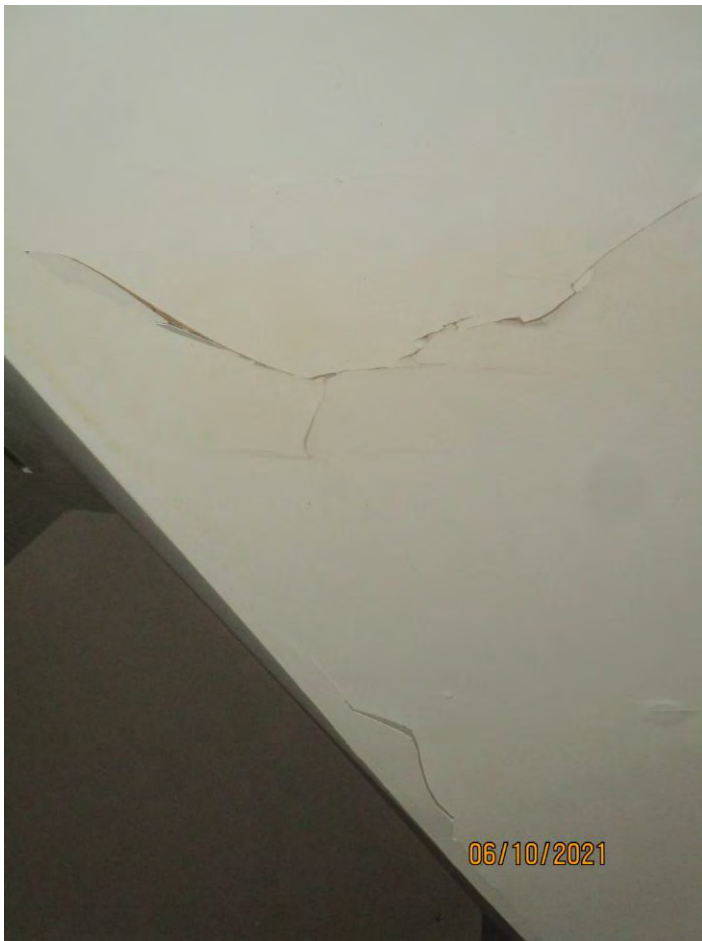
Photograph 91: Typical drywall cracks in master bedroom.
