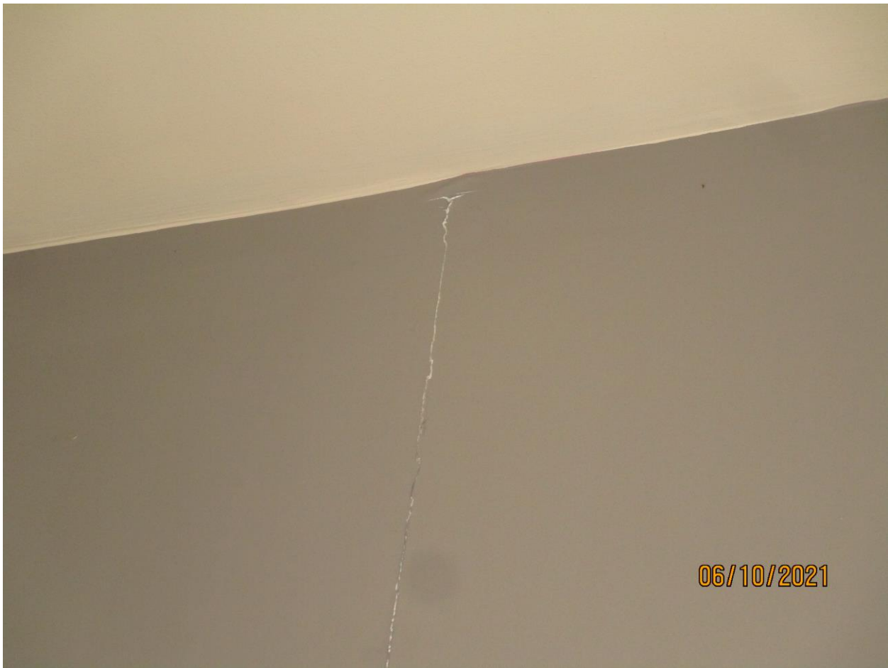
Photograph 73: Typical drywall cracks in formal living room.
