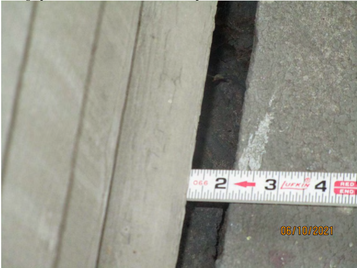
Photograph 4: Horizontal movement of front porch.
