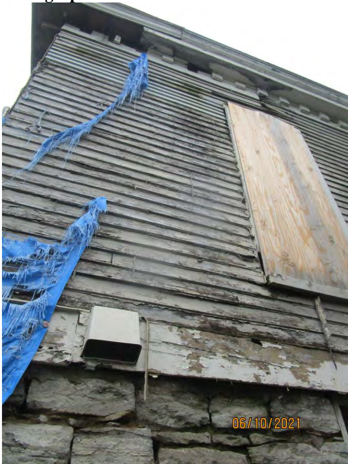
Photograph 24: Rotten soffit at left rear corner.
