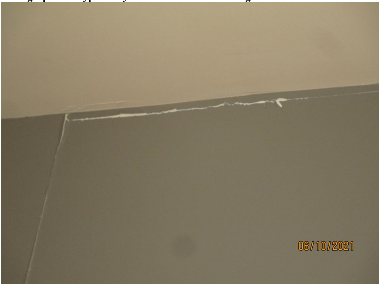
Photograph 70: Typical drywall cracks in formal living room.
