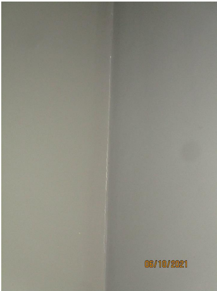
Photograph 83: Typical drywall cracks in dining room.
