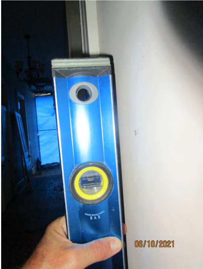
Photograph 74: Out-of-plumb right hallway wall.
