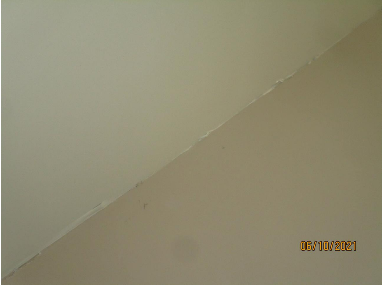
Photograph 90: Typical drywall cracks in master bedroom.
