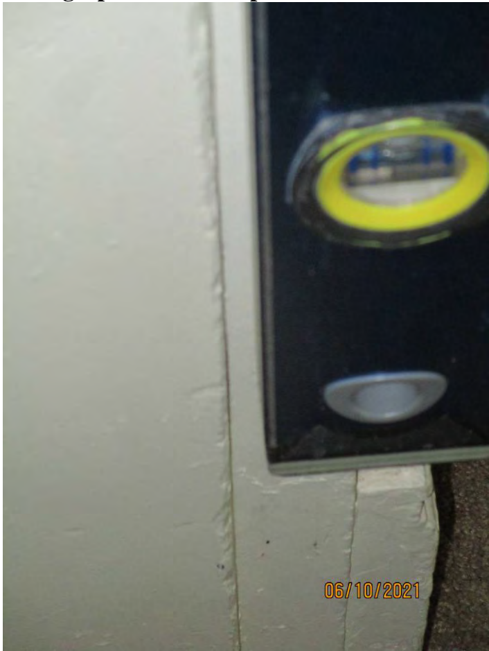
Photograph 80: Out-of-plumb door frame.
