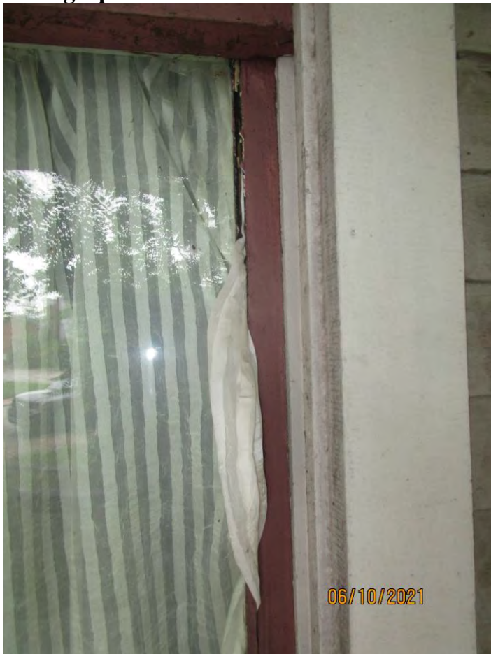
Photograph 8: Suction forces on front windows.
