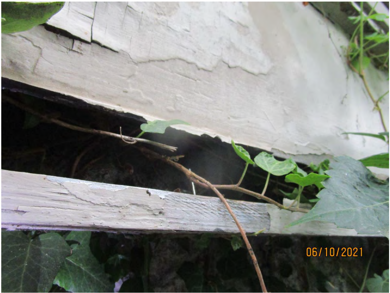
Photograph 17: Rotten band board at right side.
