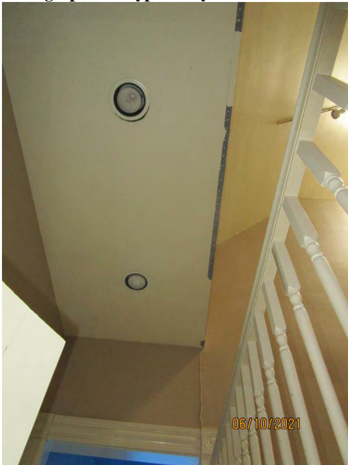
Photograph 86: Typical drywall cracks in laundry room.
