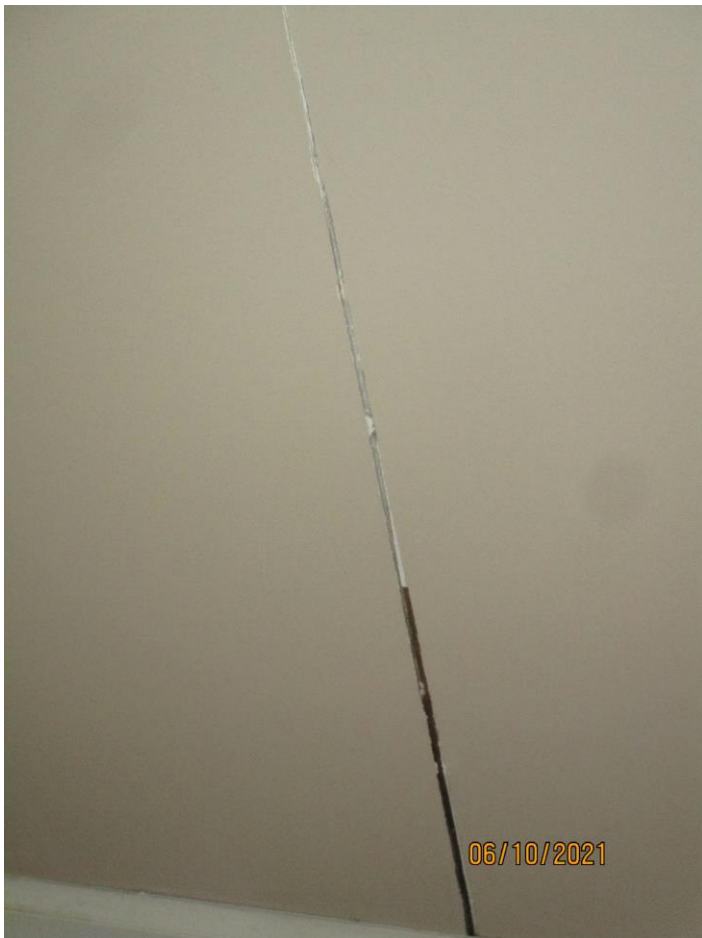
Photograph 93: Typical drywall cracks in master bedroom.
