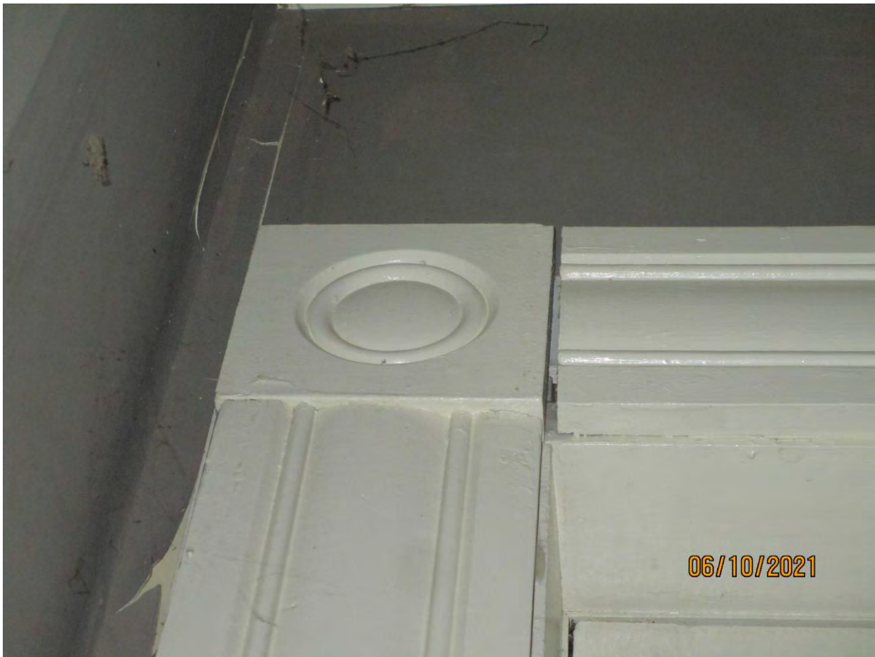
Photograph 77: Typical wood trim separating in dining room.
