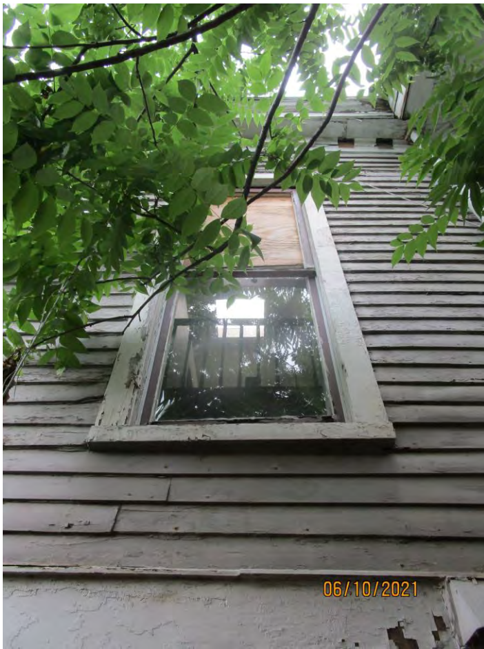
Photograph 25: Rotten soffit at left sidewall at interior gutter.
