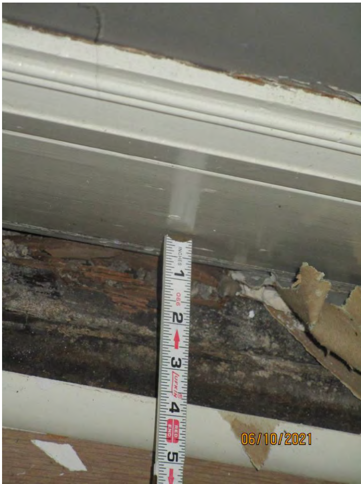
Photograph 69: Displaced left sidewall of formal living room.
