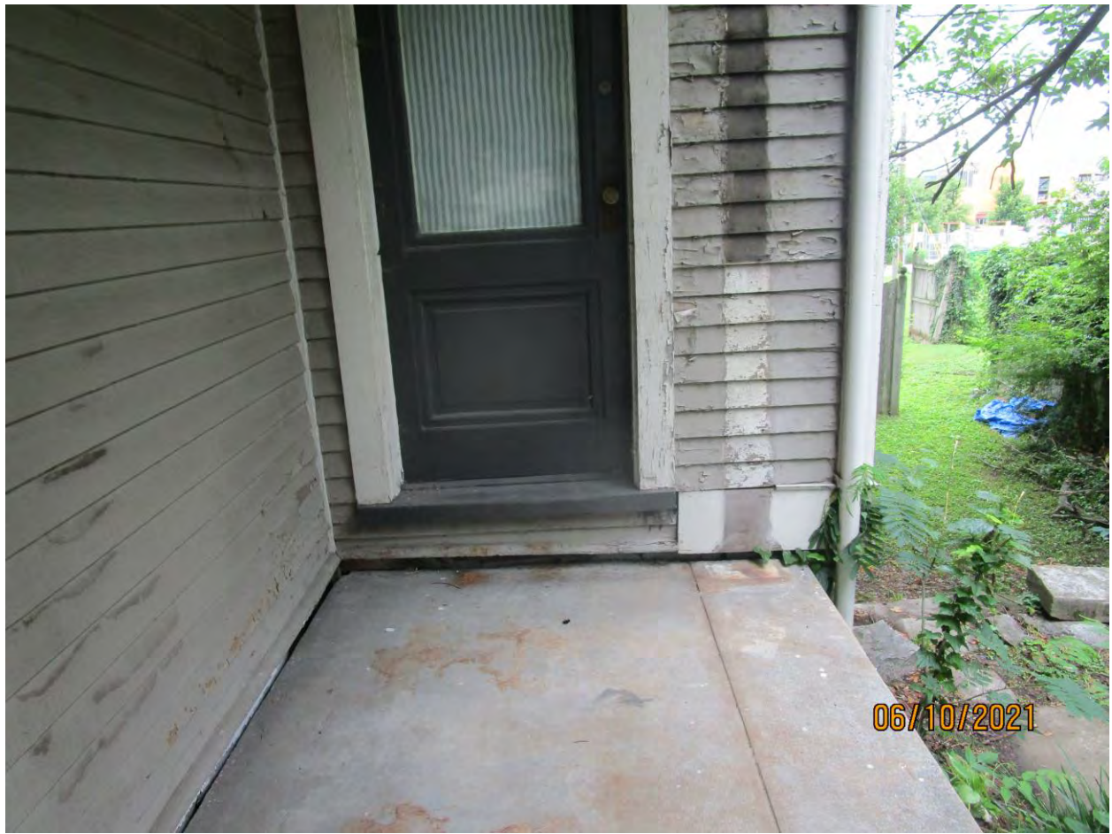
Photograph 9: Vertical settlement of front porch.
