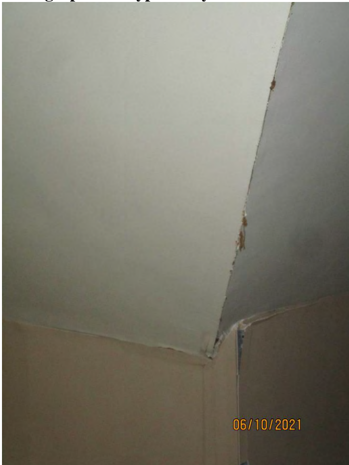
Photograph 92: Typical drywall cracks in master bedroom.
