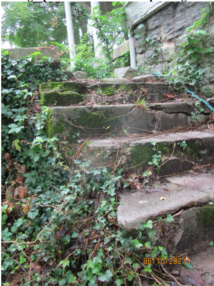
Photograph 30: Deteriorated steps at right side of property.
