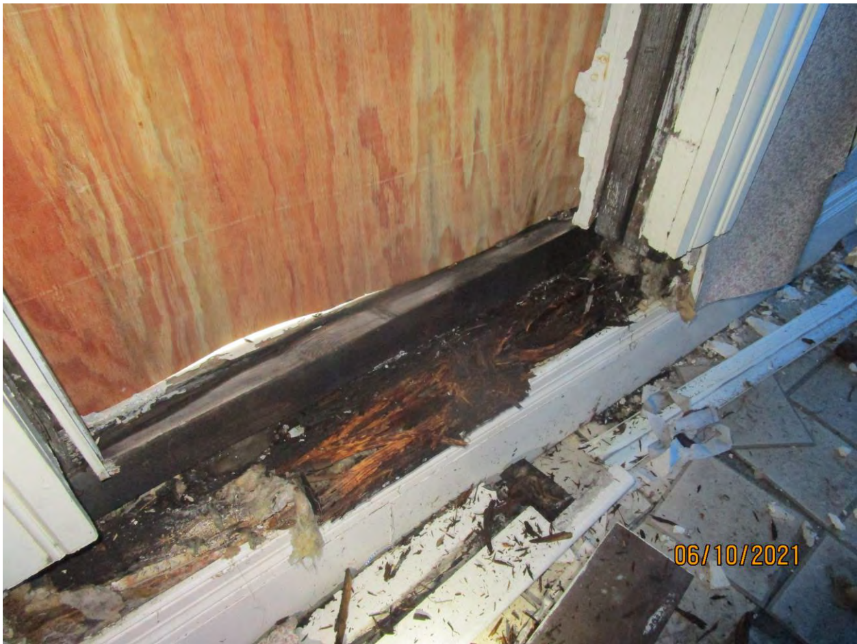
Photograph 89: Rotten wall framing in kitchen.
