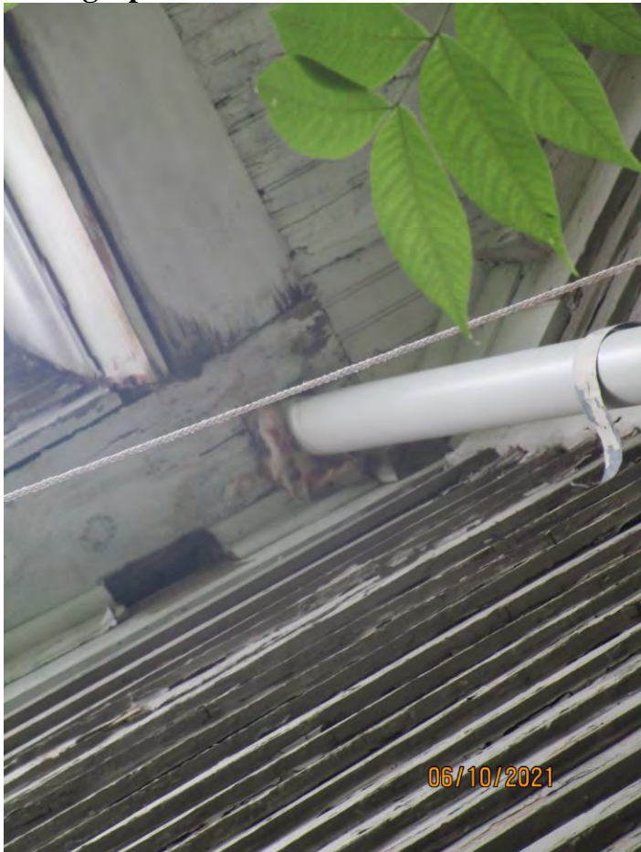
Photograph 26: Rotten soffit at left sidewall at interior gutter.
