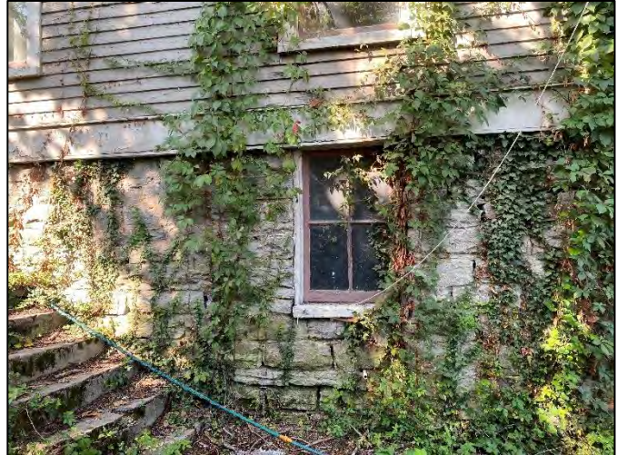
Figure 7: Foundation wall on the east side shows mortar joints that have deteriorated but is overall in good condition.
