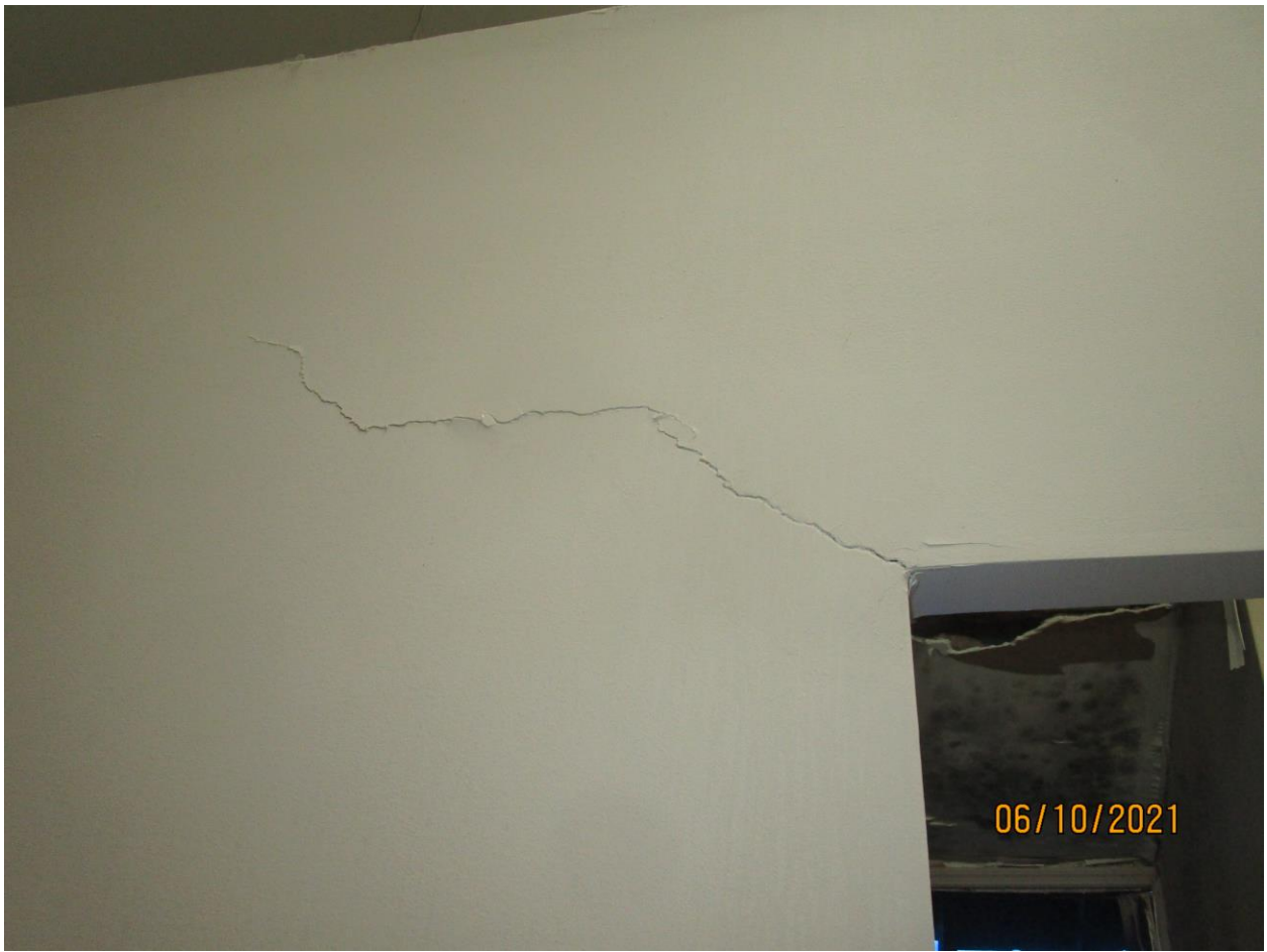
Photograph 101: Typical drywall cracks in master bedroom.
