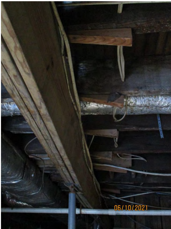
Photograph 39: Previously replaced wood beam (inadequate).
