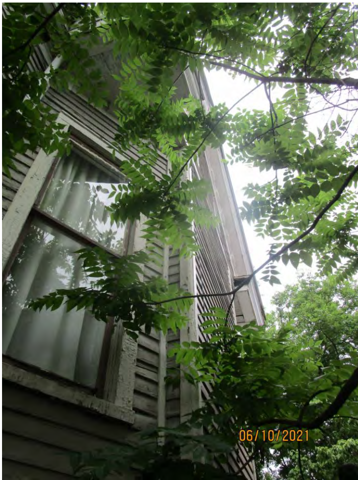
Photograph 27: Rotten soffit at left sidewall.
