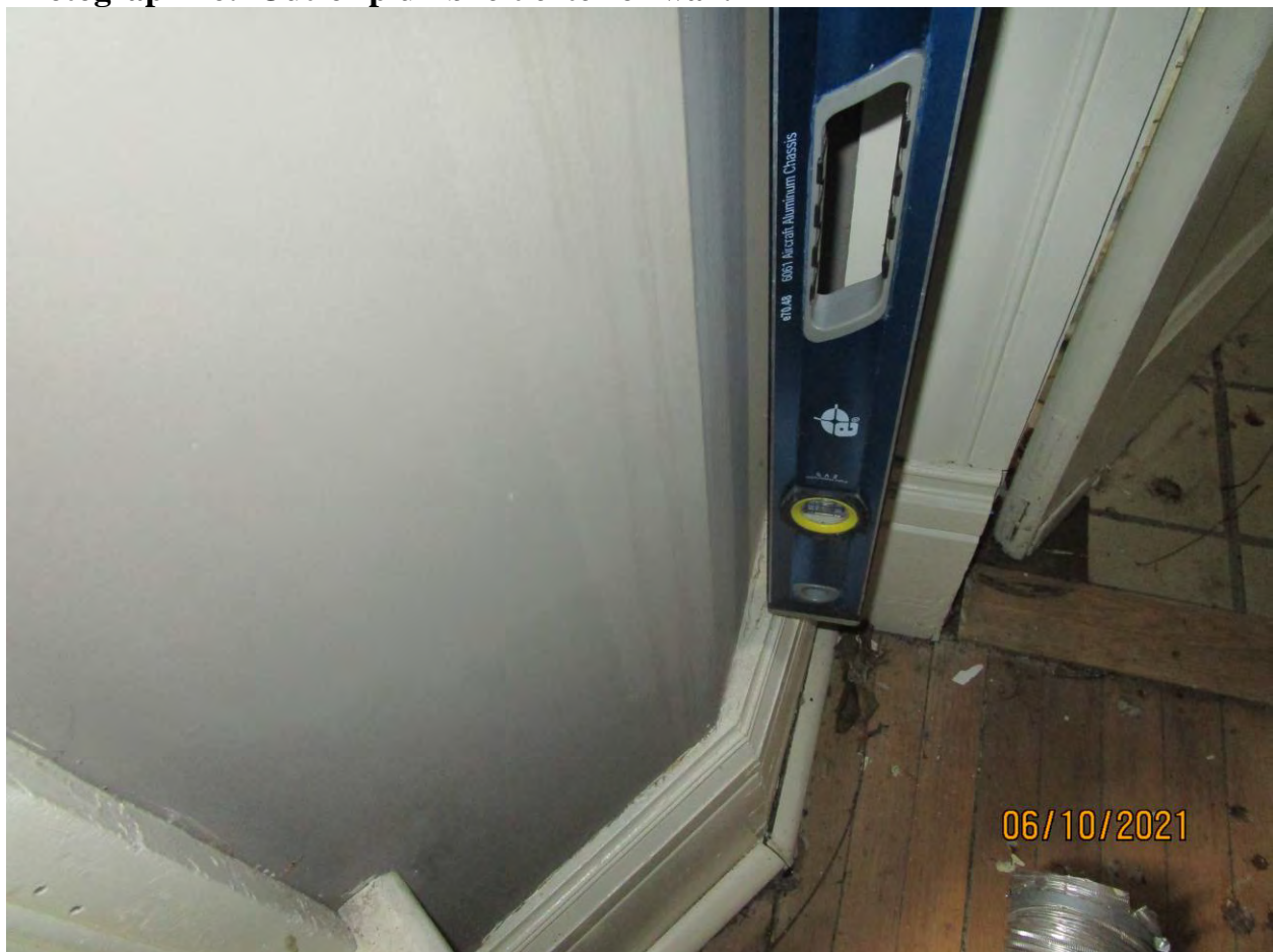
Photograph 76: Out-of-plumb left exterior wall.
