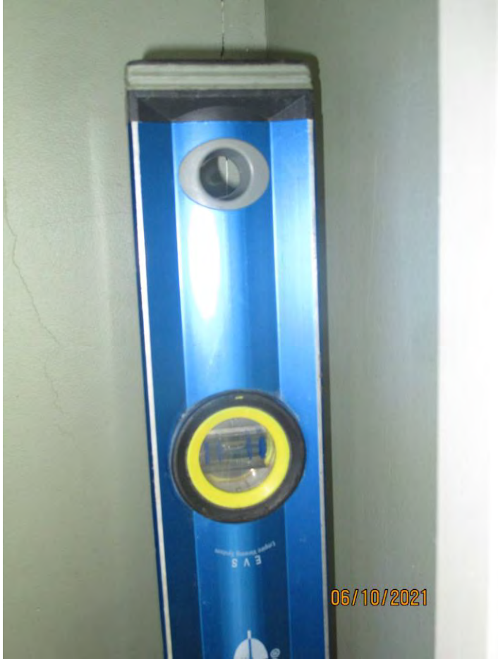
Photograph 78: Out-of-plumb wall at left hallway wall.
