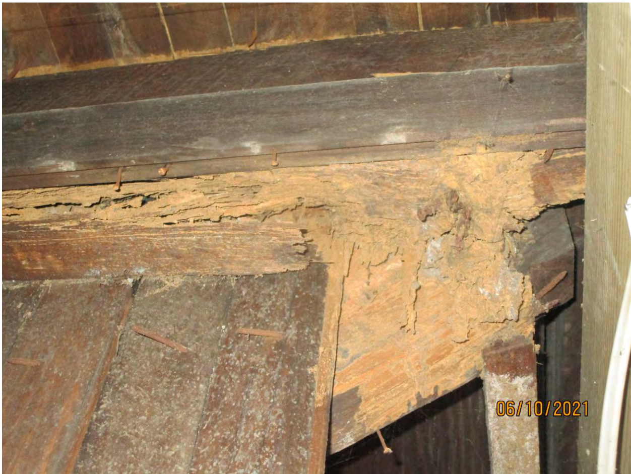
Photograph 53: Typical insect infestation issues with wood joists.
