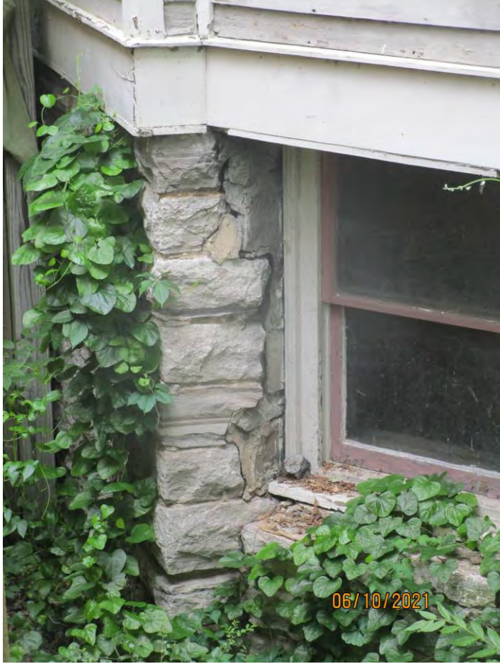
Photograph 34: Settlement of left sidewall at bay window.
