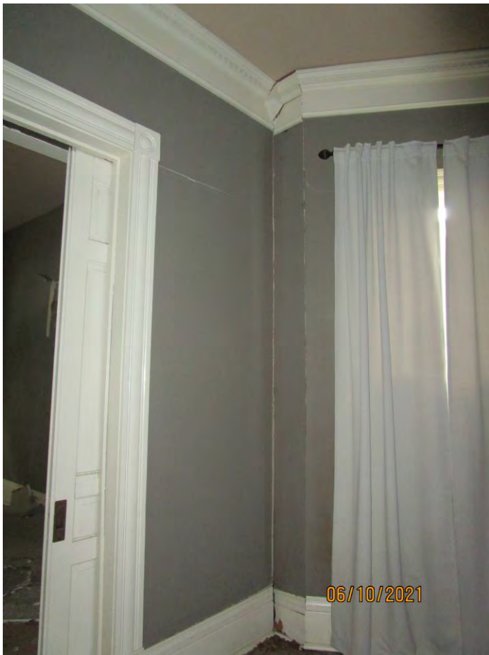
Photograph 81: Typical drywall cracks in dining room.
