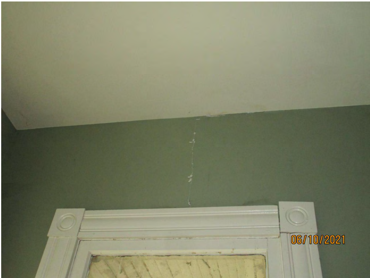
Photograph 79: Typical drywall cracks in dining room.
