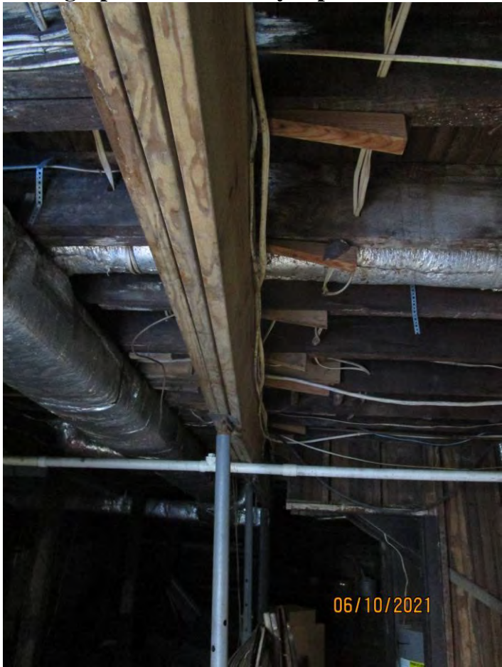
Photograph 38: Previously replaced wood beam (inadequate).
