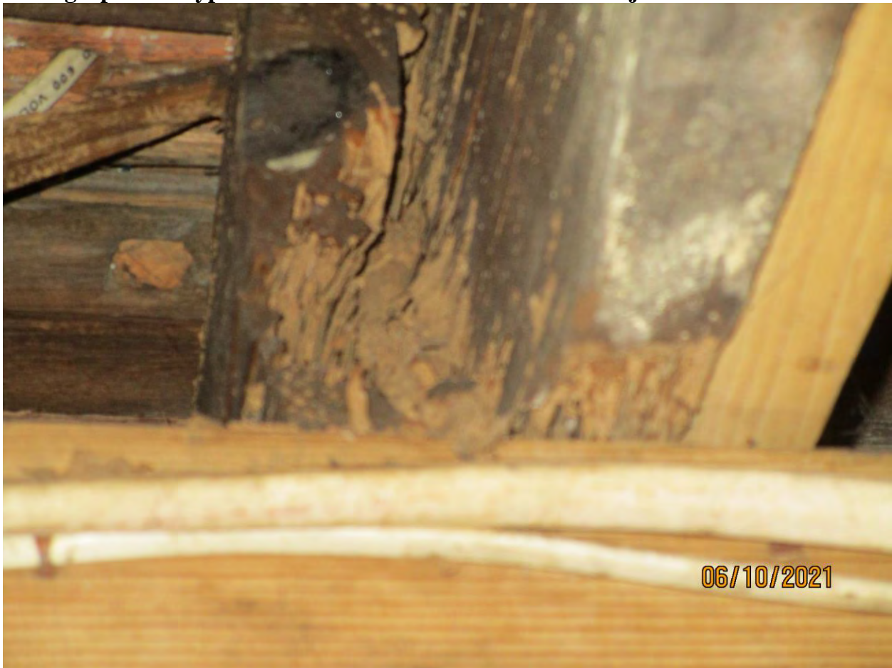
Photograph 54: Typical insect infestation issues with wood joists.
