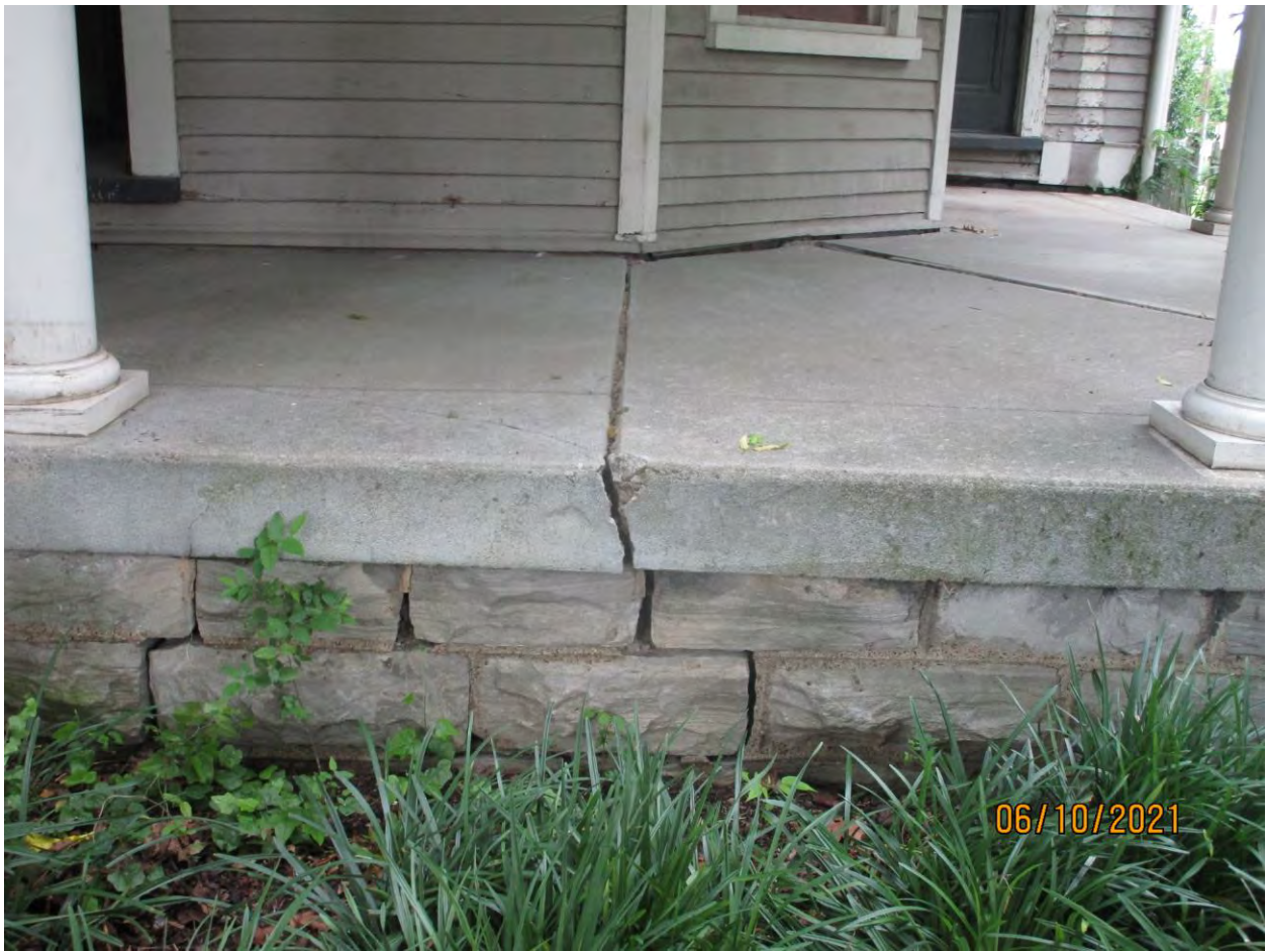
Photograph 13: Settlement of front porch foundation wall.
