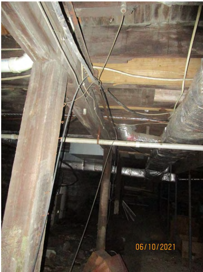
Photograph 41: Original wood beam (inadequate).
