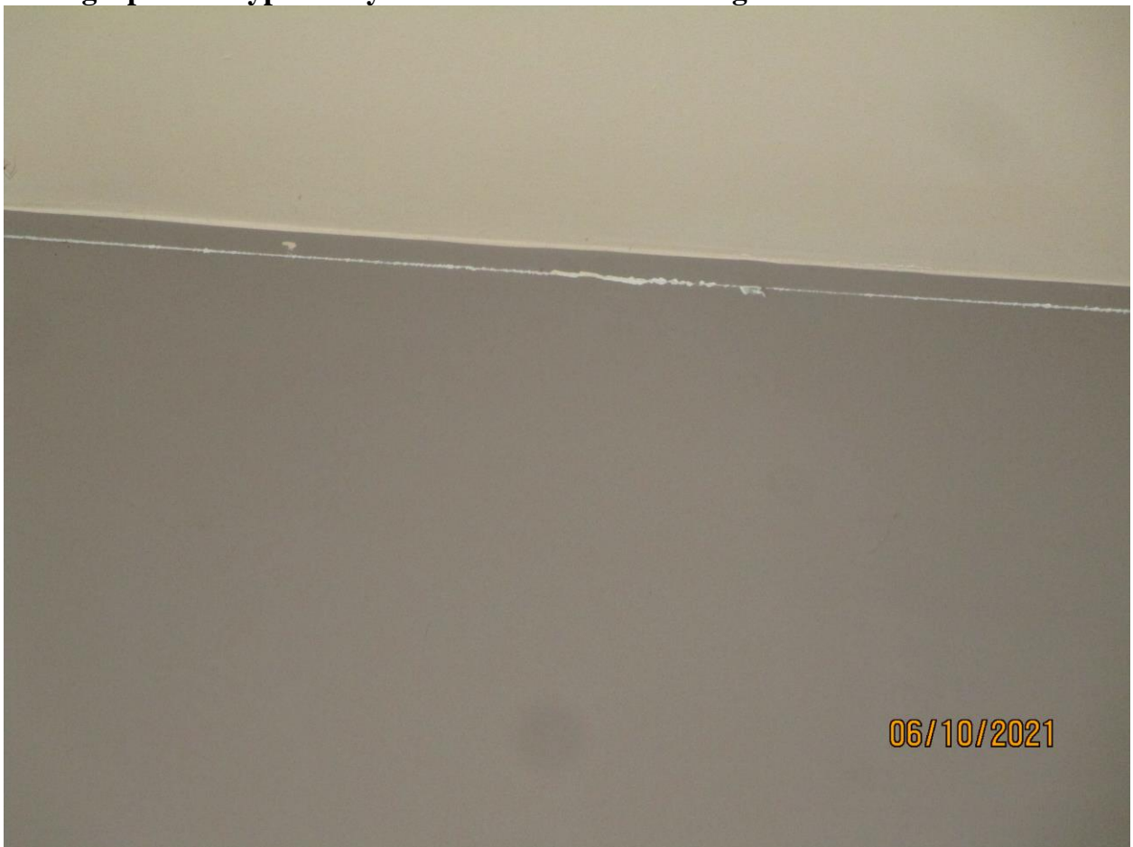
Photograph 72: Typical drywall cracks in formal living room.
