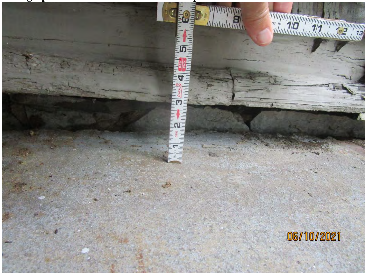
Photograph 10: Vertical settlement of front porch.
