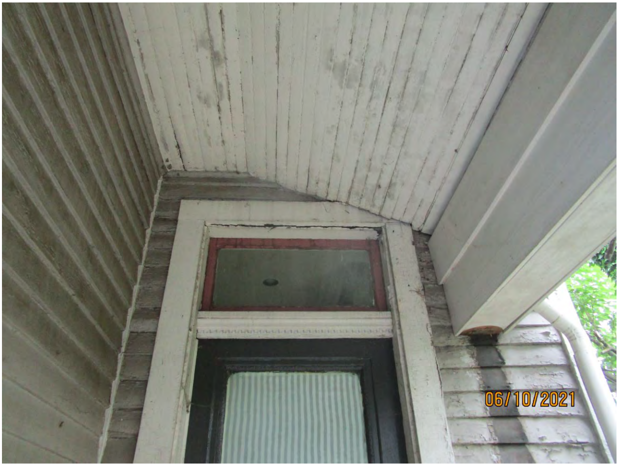
Photograph 11: Rotten wood at side door of porch area.
