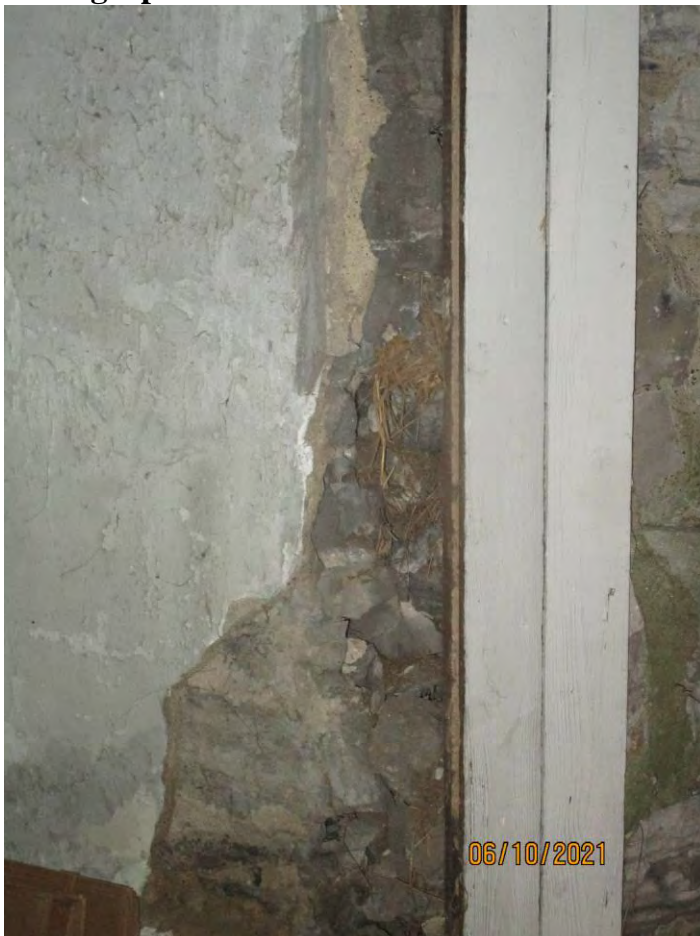
Photograph 52: Left sidewall foundation issues.
