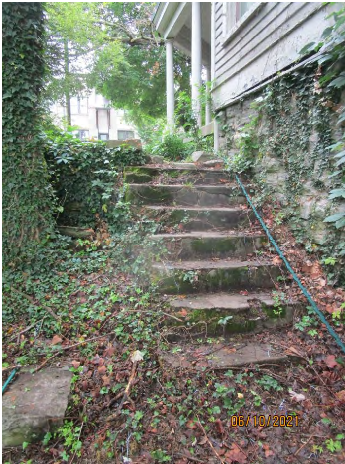
Photograph 29: Deteriorated steps at right side of property.
