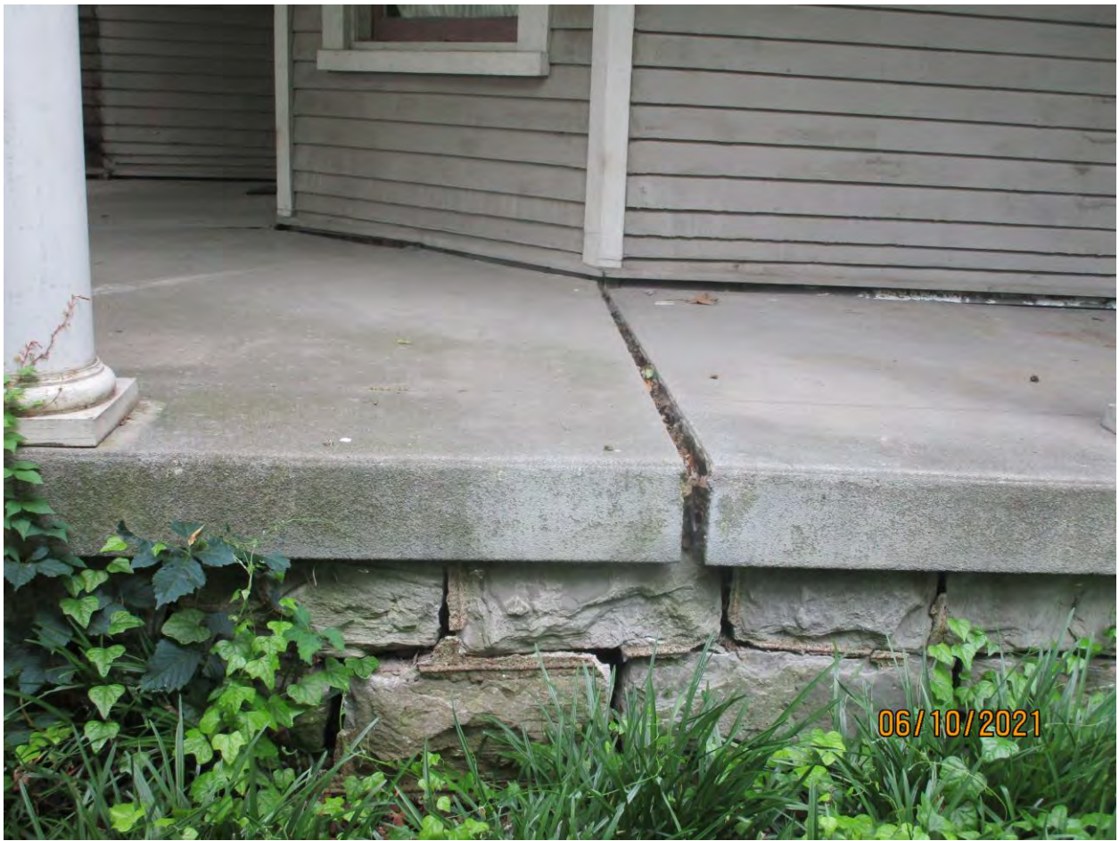
Photograph 15: Settlement of front porch foundation wall.
