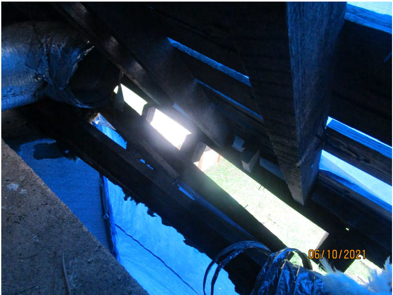
Photograph 99: View of displaced rear wall.
