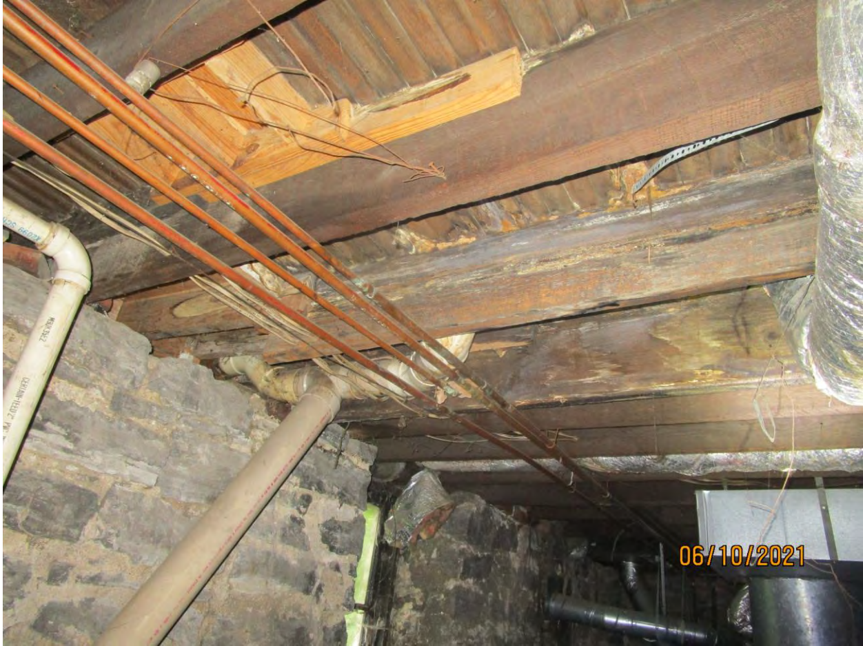
Photograph 44: Right sidewall foundation wall issues.
