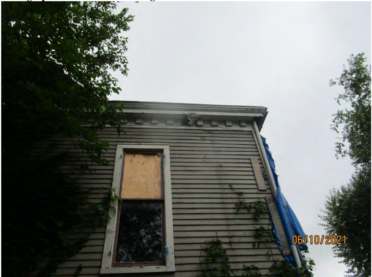
Photograph 18: Rotten soffit at right rear corner.
