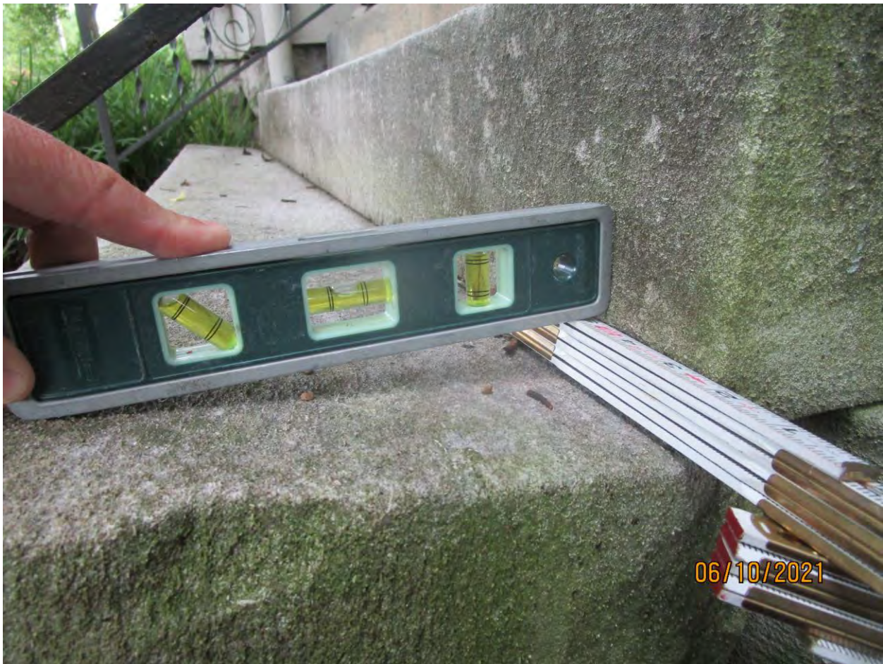
Photograph 3: Out-of-level front steps.
