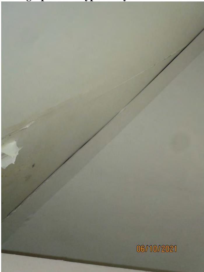
Photograph 100: Typical drywall cracks in master bedroom.
