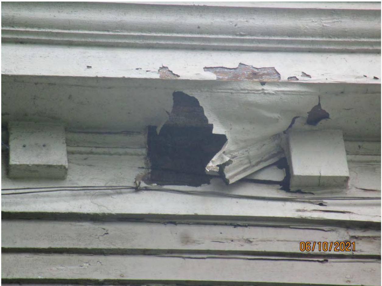
Photograph 19: Rotten soffit at right rear corner.
