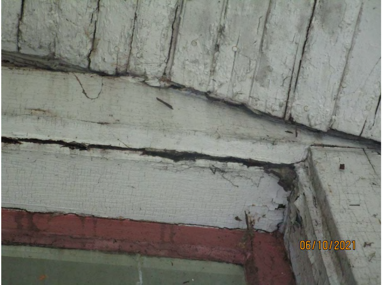
Photograph 12: Rotten wood at side door of porch area.
