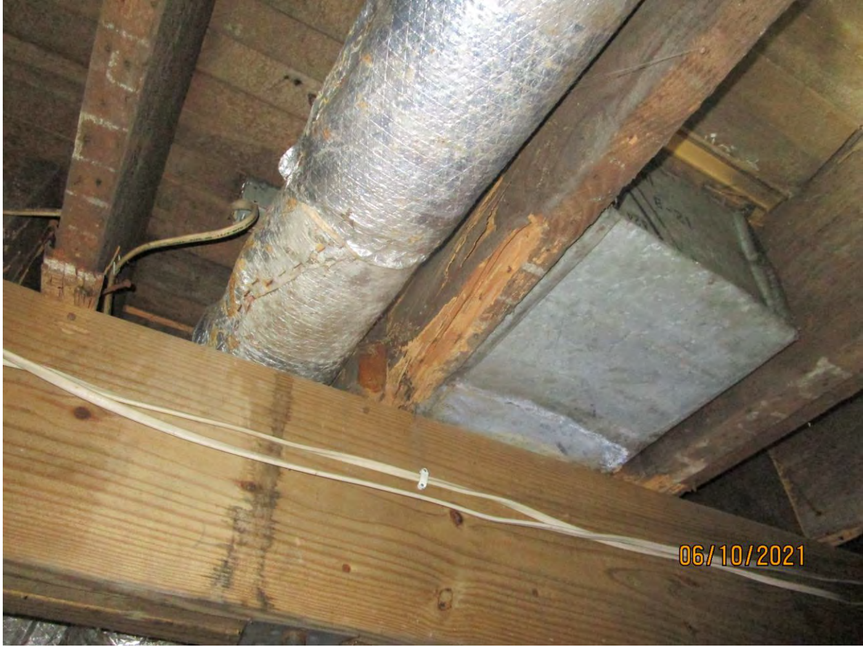
Photograph 50: Typical insect infestation of wood joists.
