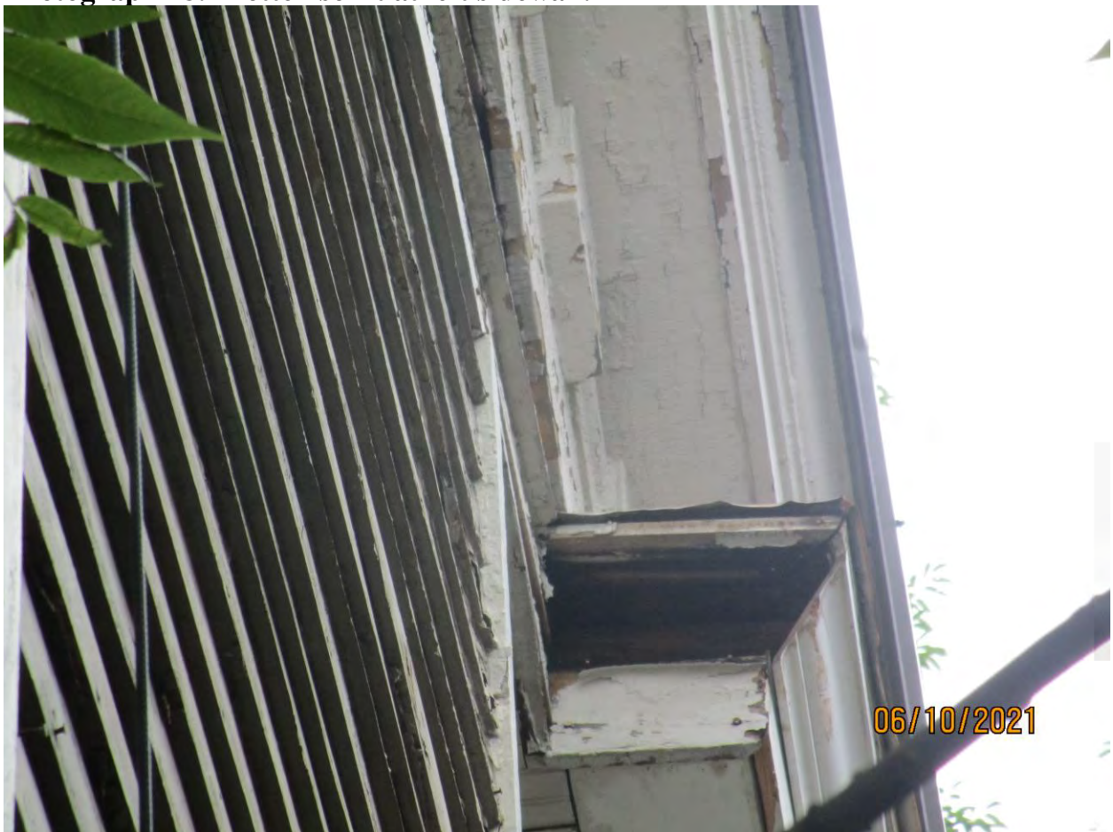
Photograph 28: Rotten soffit at left sidewall.
