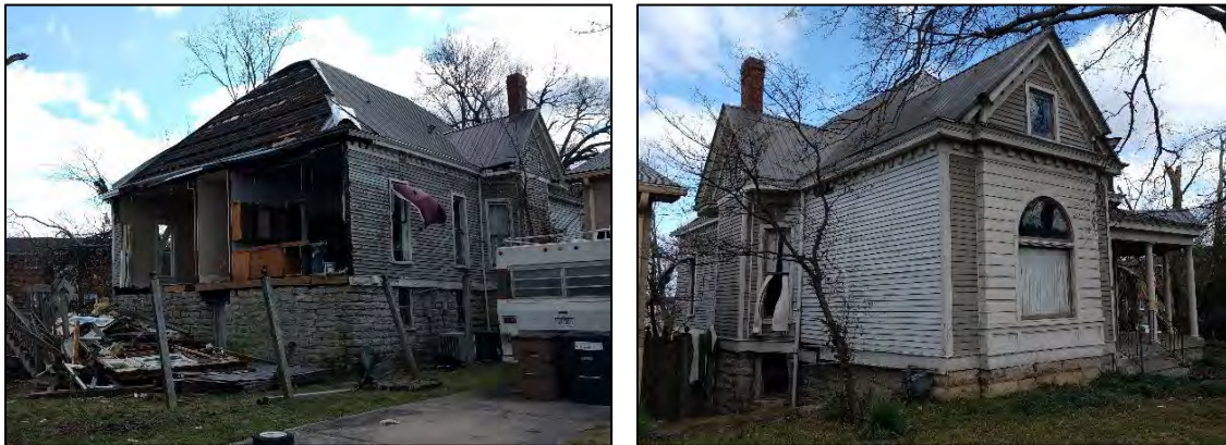
Figures 5 and 6: The house as seen after the storm on March 6, 2020.
