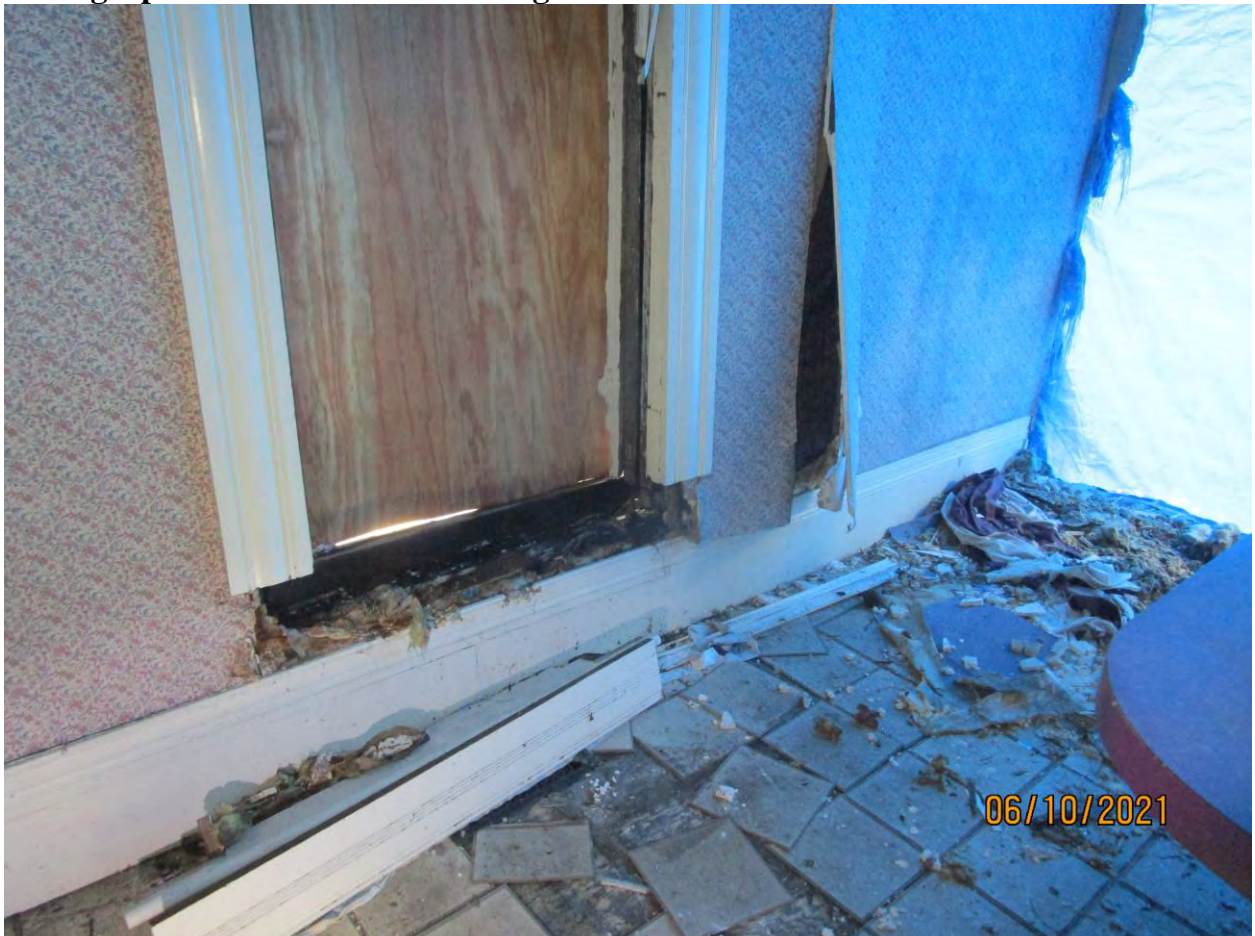
Photograph 88: Rotten wall framing in kitchen.
