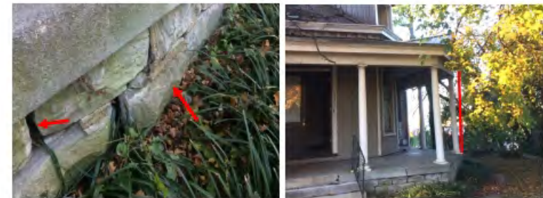
22. The porch section at the front door is cracked in the center and sloping towards the left, directing any water that blows onto the porch surface towards the right side wall of the front living room.
