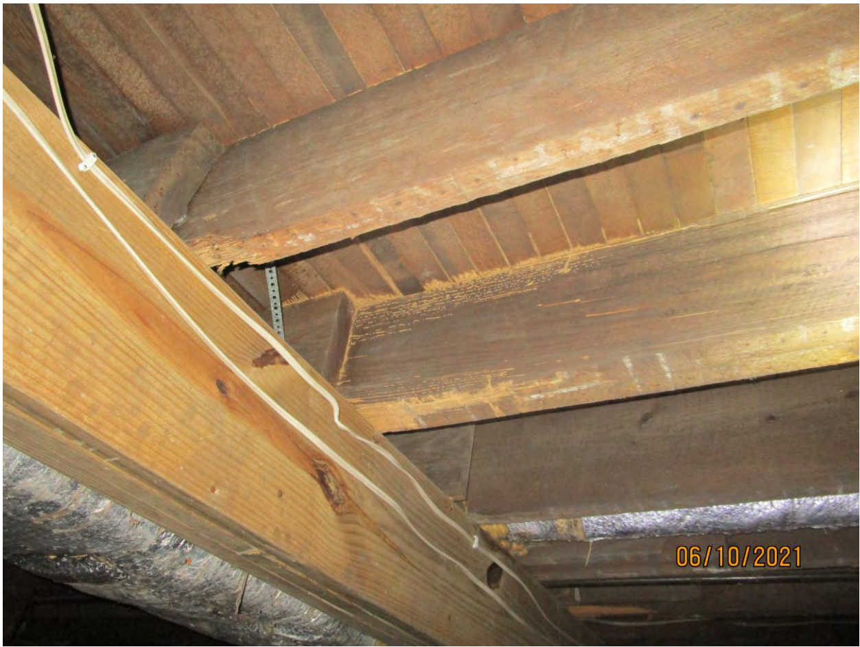
Photograph 51: Typical insect infestation of wood joists.
