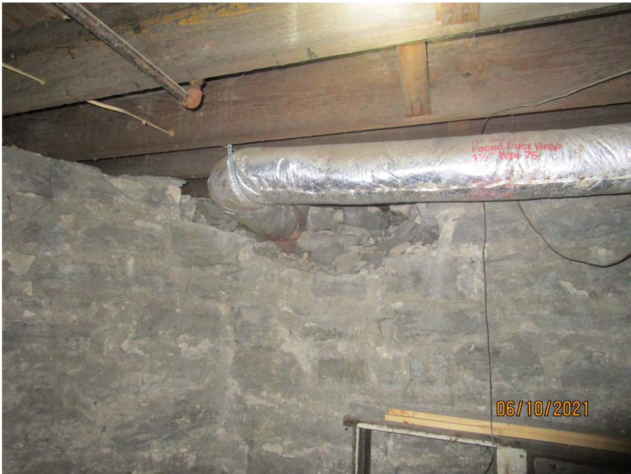
Photograph 47: Front wall foundation wall issues.
