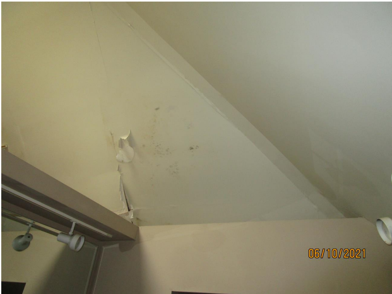
Photograph 97: Typical drywall cracks in master bedroom.
