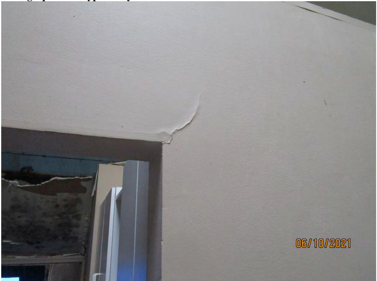
Photograph 102: Typical drywall cracks in master bedroom.
