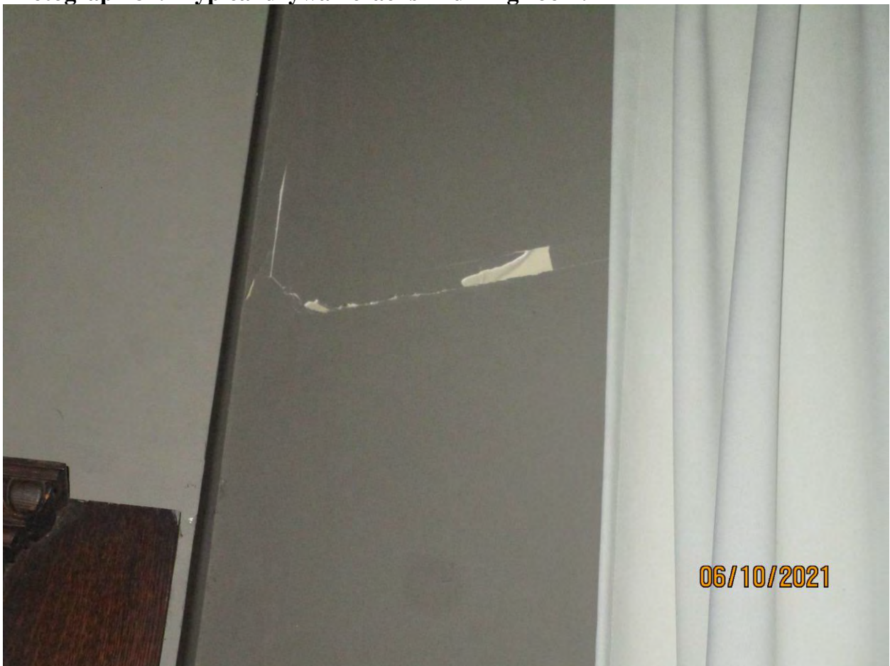
Photograph 84: Typical drywall cracks in dining room.
