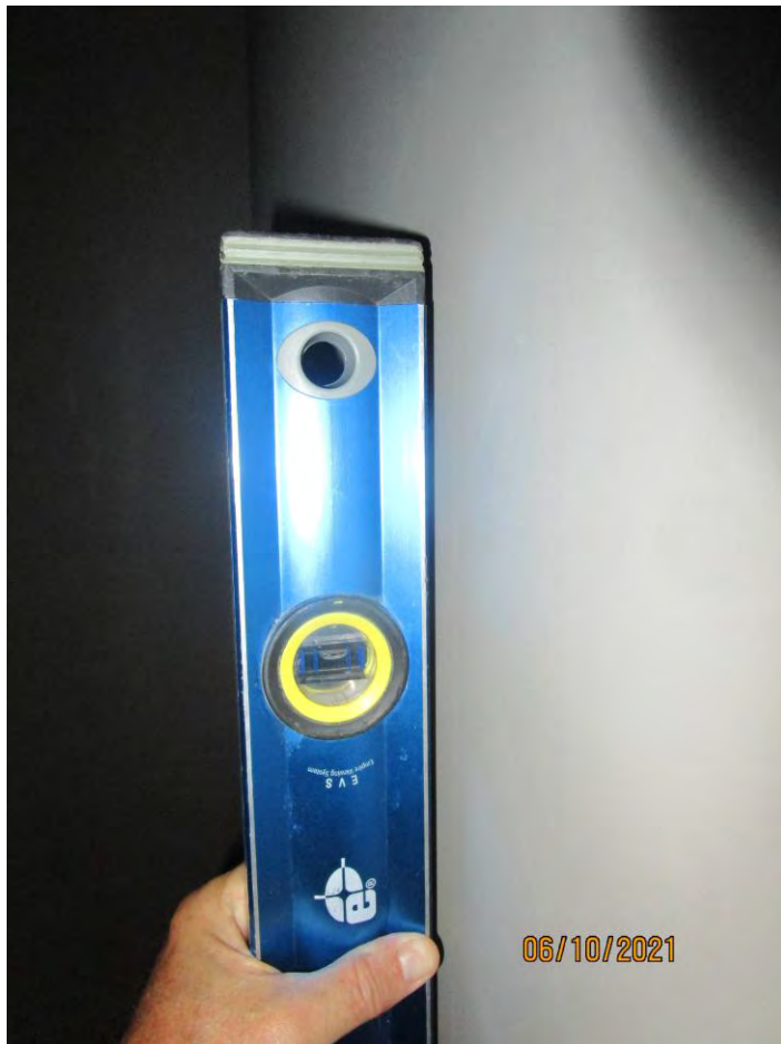
Photograph 75: Out-of-plumb right exterior wall.
