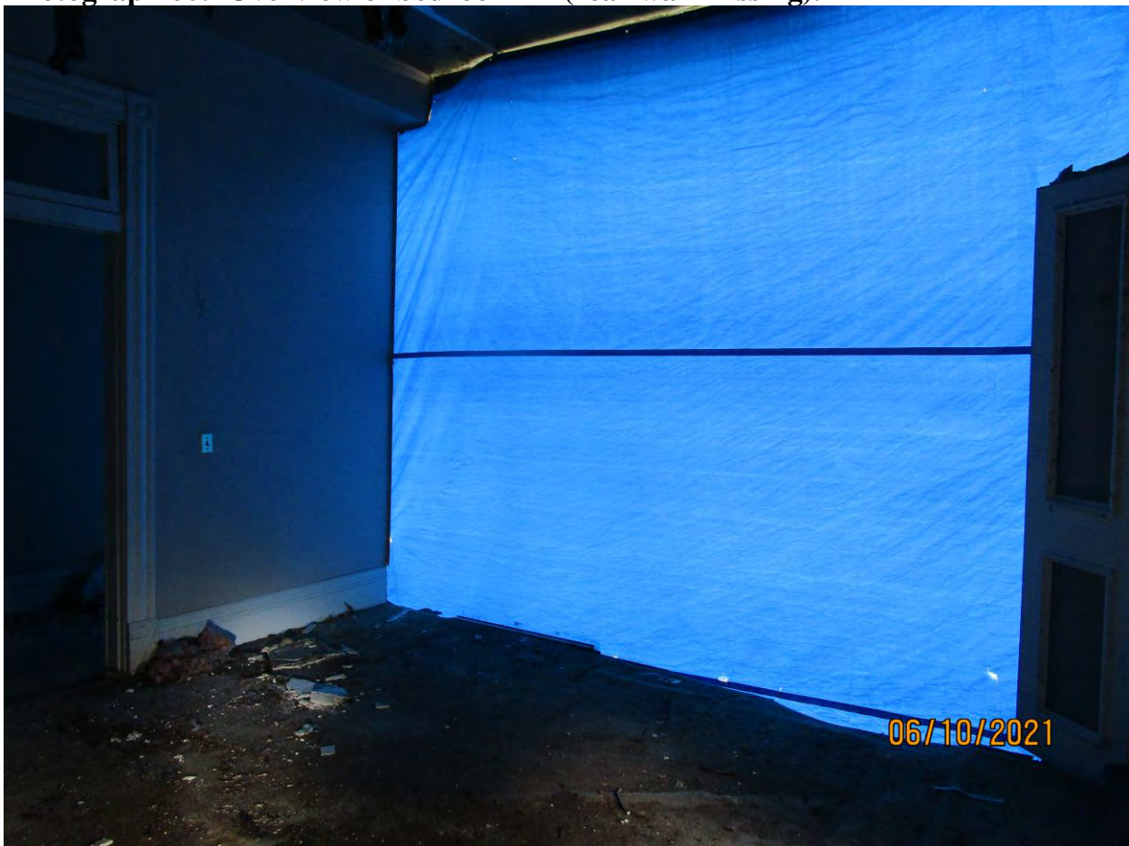
Photograph 60: Overview of bedroom #2 (rear wall missing).
