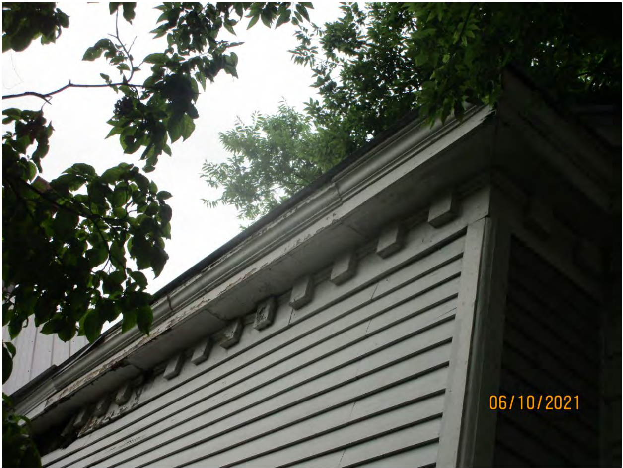
Photograph 35: Previously repaired interior gutter.
