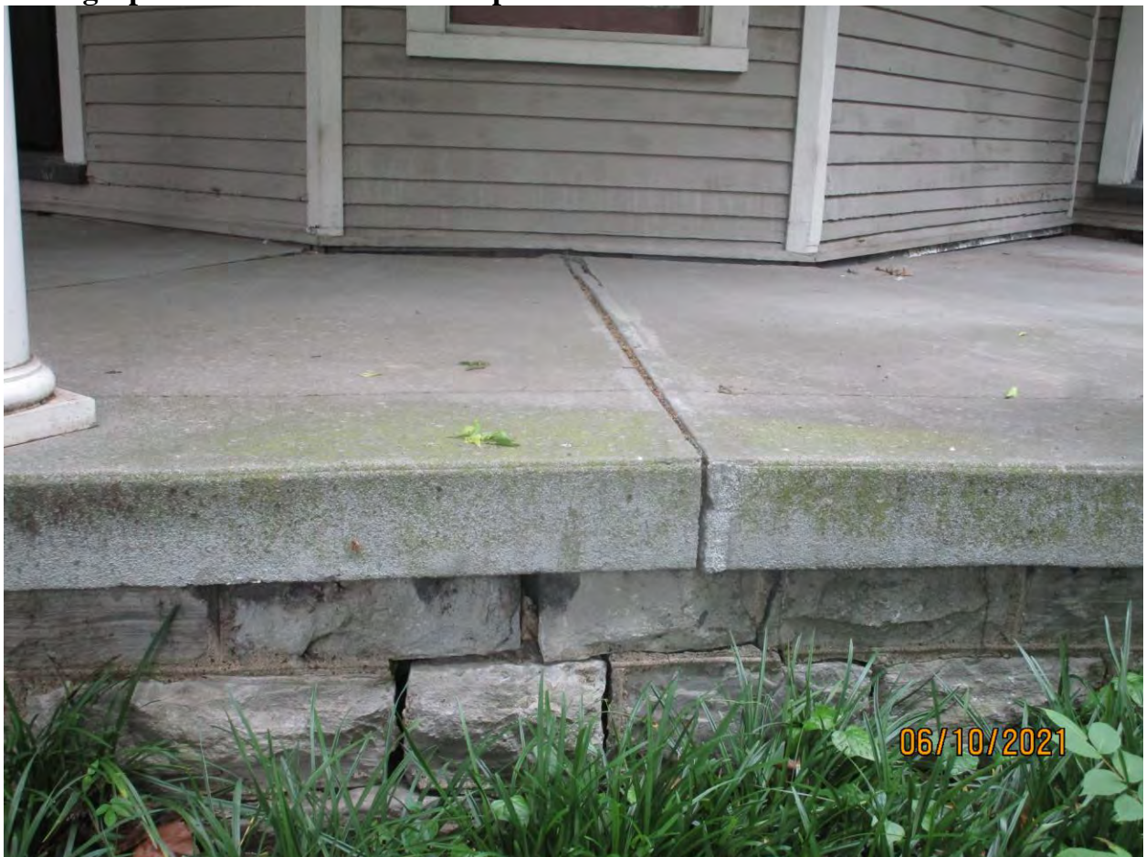
Photograph 14: Settlement of front porch foundation wall.
