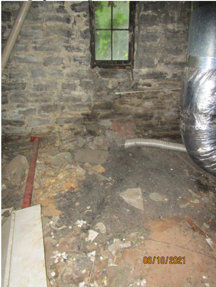
Photograph 46: Right sidewall foundation wall issues.
