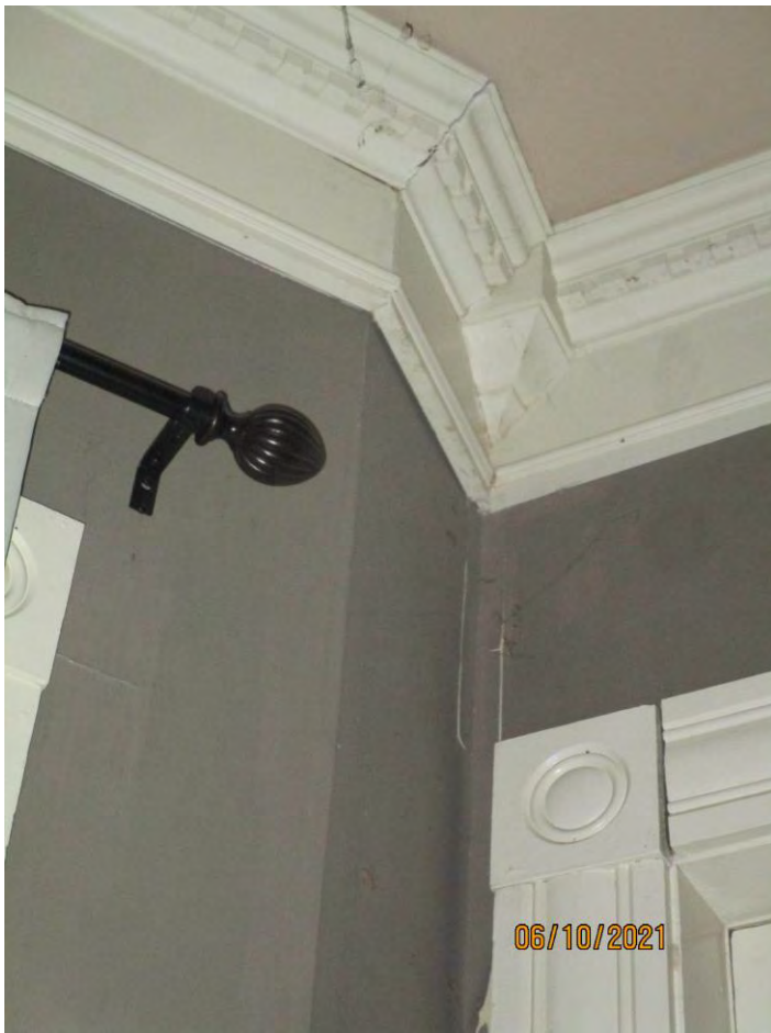
Photograph 85: Typical drywall cracks in dining room.
