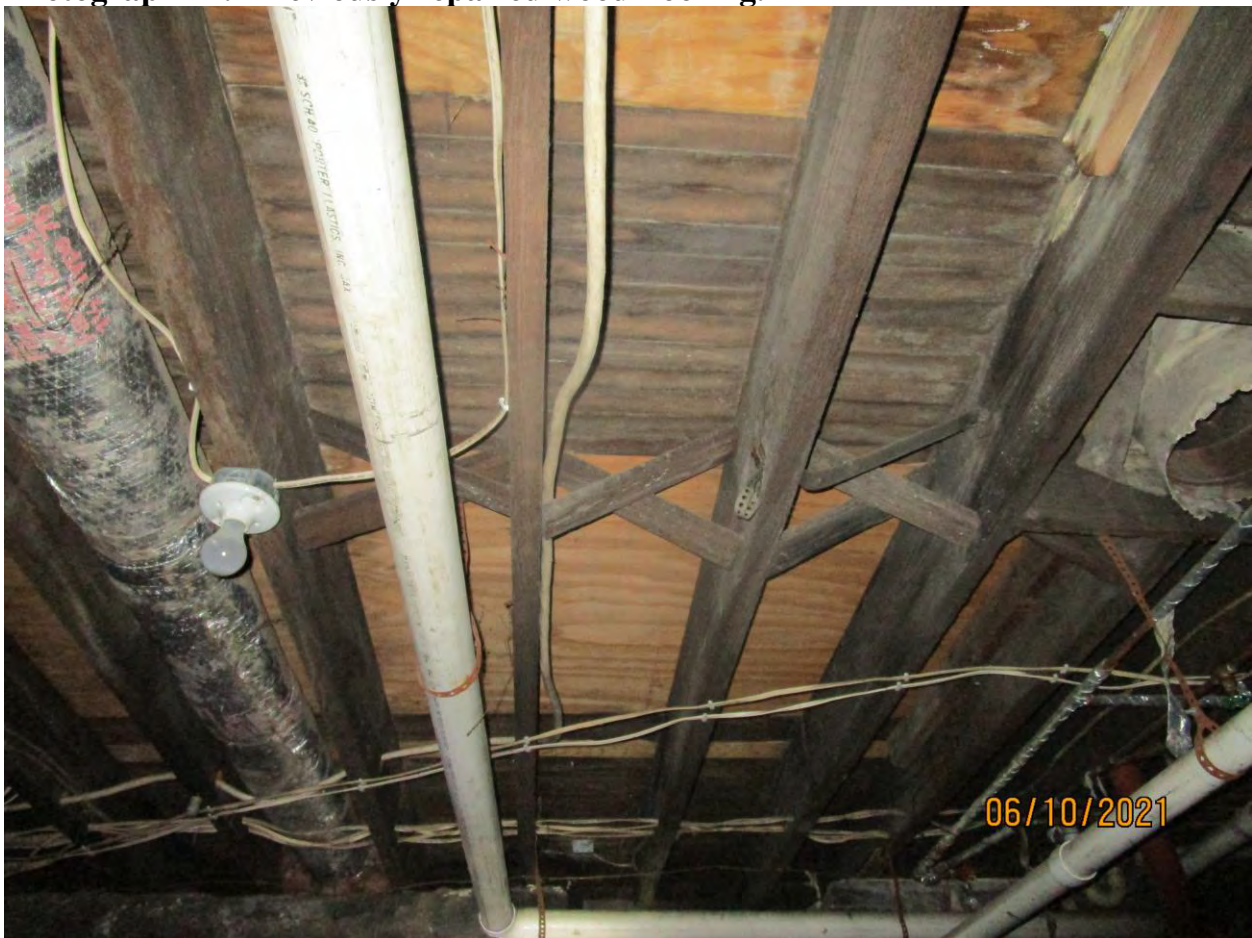
Photograph 42: Previously repaired wood flooring.
