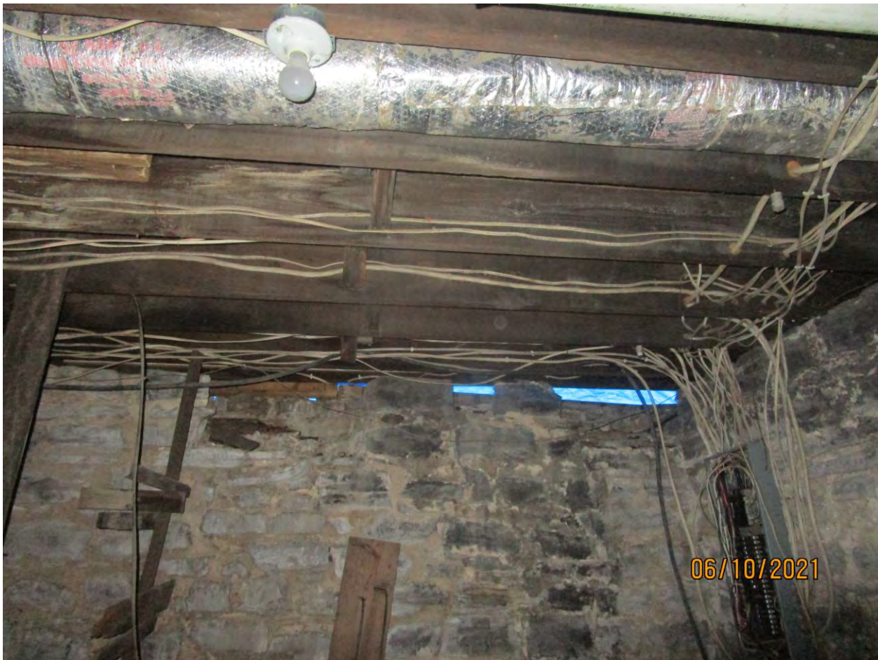
Photograph 43: Rear foundation wall issues.
