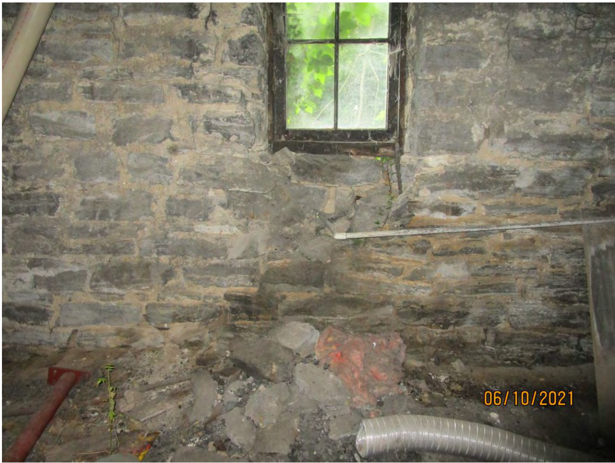
Photograph 45: Right sidewall foundation wall issues.
