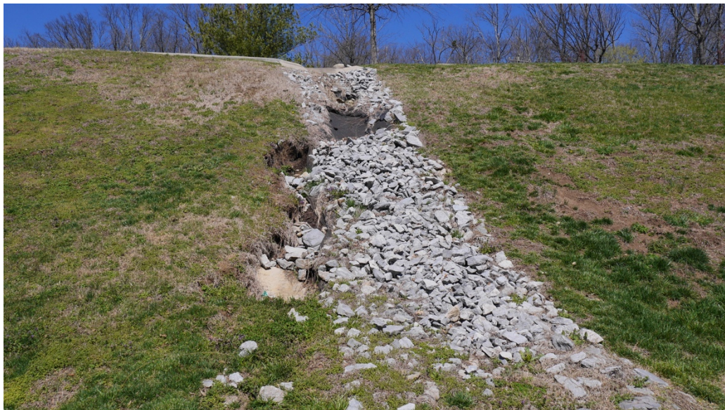
Knob Hill runoff continually breaking down church parking lot gravel gutters
