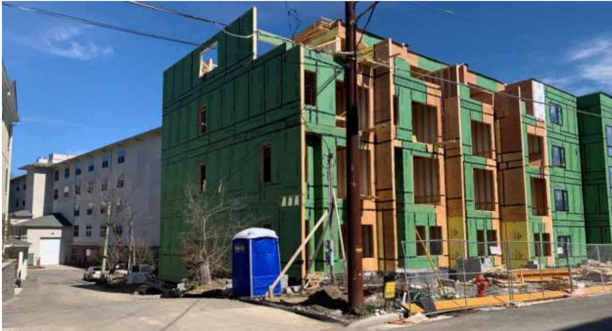
Figure 3: Existing Non-compliant Construction
