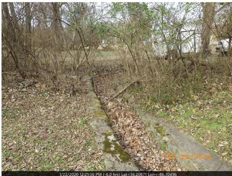
3. View of the D-1 concrete channel at the beginning of the assessed reach, facing upstream.
