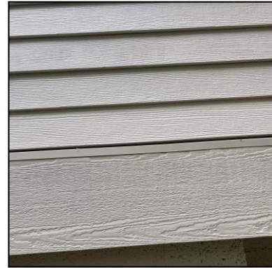
Figure 2: Installed lap siding has a faux grain, specifically called out in the design guidelines as an inappropriate material.
