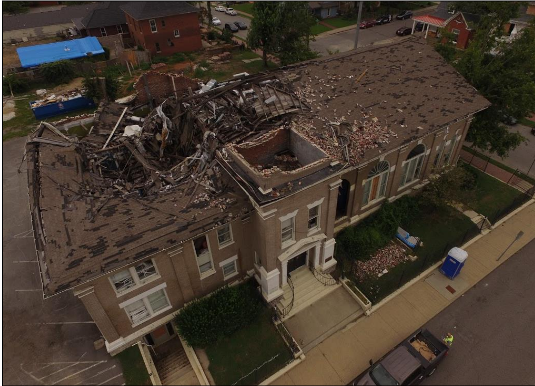
Figure 4. Aerial photo of damage to 1021 Russell Street from March 2020 tornado.
