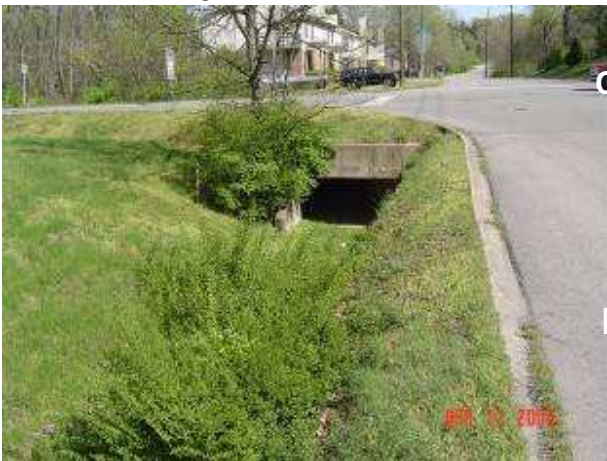
Fig. 1. Northerly view of existing 9' by 4' box culvert (Photo taken by J. Honeycutt, MPW)
