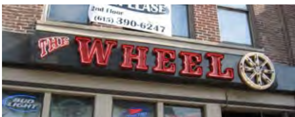
Example of raceway incorporated as sign background
