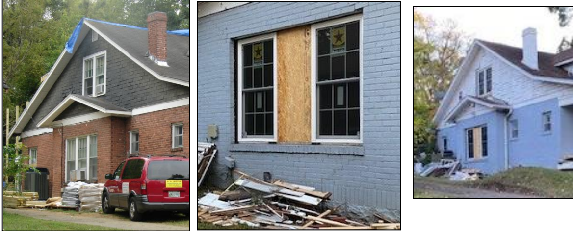
Figures 1-3: The left image shows the original 3-window configuration as seen in 2010 and the two images to the right show the change, under construction.
