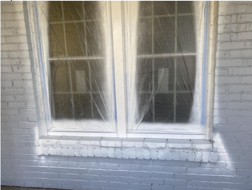
Paired window on front porch. Brick mold was retained, but a row of brick was added to compensate for the incorrect window size.
