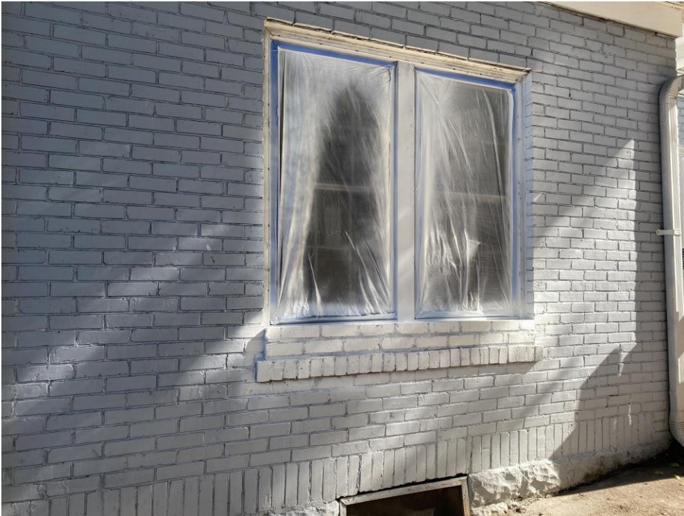
Windows on right side had two rows of brick added to compensate for the difference in height of new windows.
