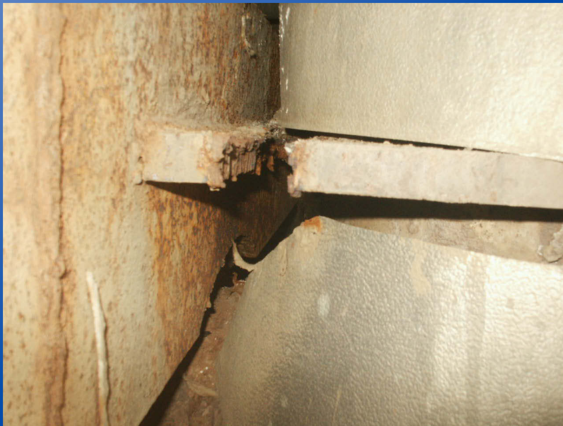
Anchor Plate Failure in MH-L
