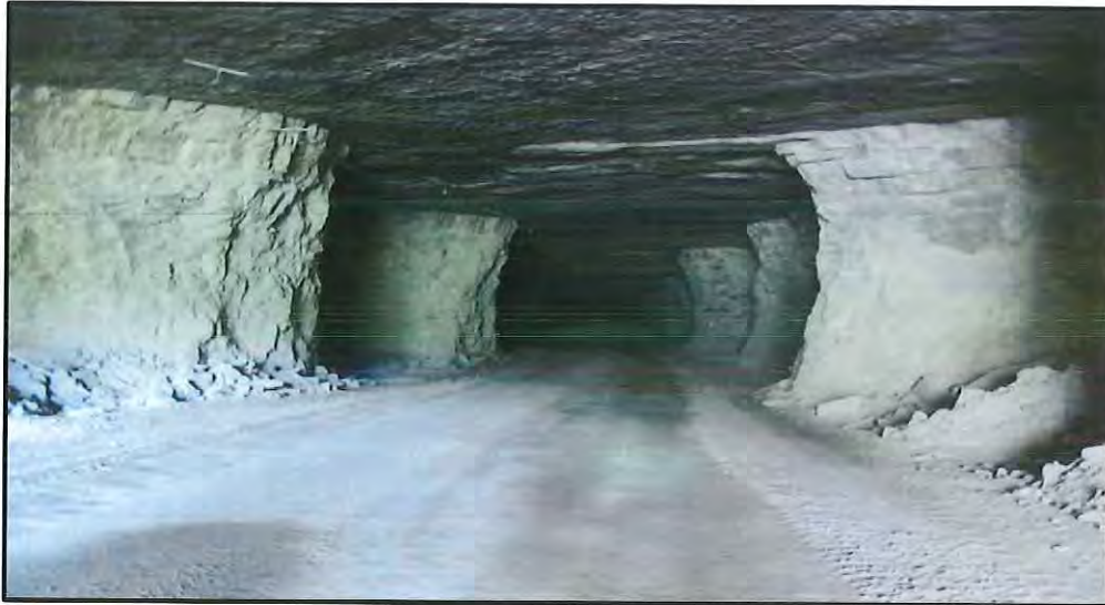
Photograph 1. Typical Opening in an Underground Limestone Mine With Competent Strata Similar to the Carters Limestone
