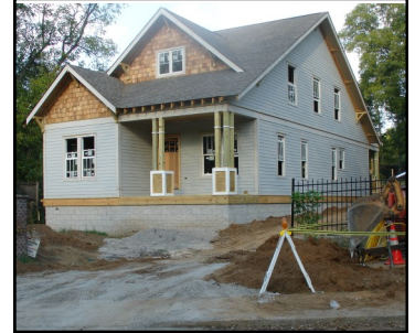
The rise in grade on this lot was not considered, resulting in a foundation significantly higher in the front than what the MHZ approved.
