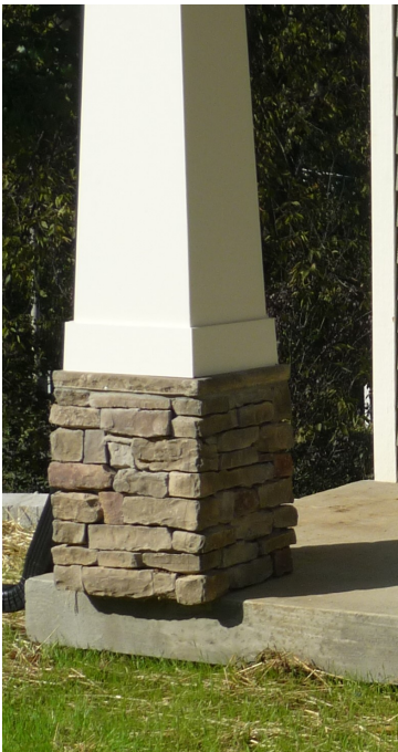
The depth of the stone veneer was not considered, leaving a porch pedestal hanging over the edge of the porch floor.
