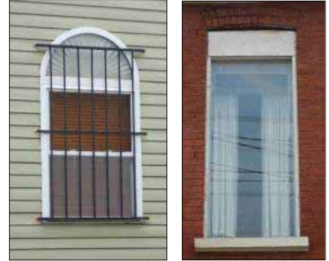
Inappropriate windows alterations.
