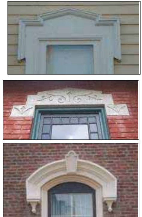
Examples of elaborate window lintels including wood (top), stone (center), and sheet metal (below).
