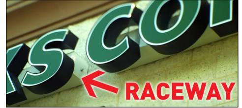
Example of sign with exposed raceway.
