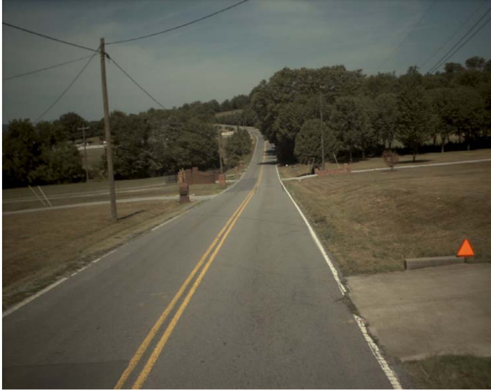
Photo 4.6. Burkitt Road, segment 40524, rutting, weathering, edge cracking, patching, and fatigue cracking.
