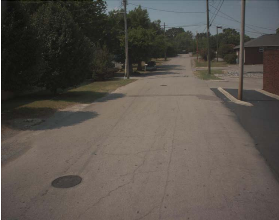
Photo 4.7. Lellyett Street, segment 5, rutting, block cracking, weathering, and linear cracking.
