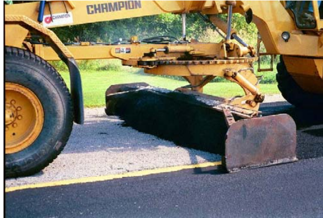
Figure C.2. Application of a scratch coat of a densely graded hot mix by a grader with box-like attachment.
