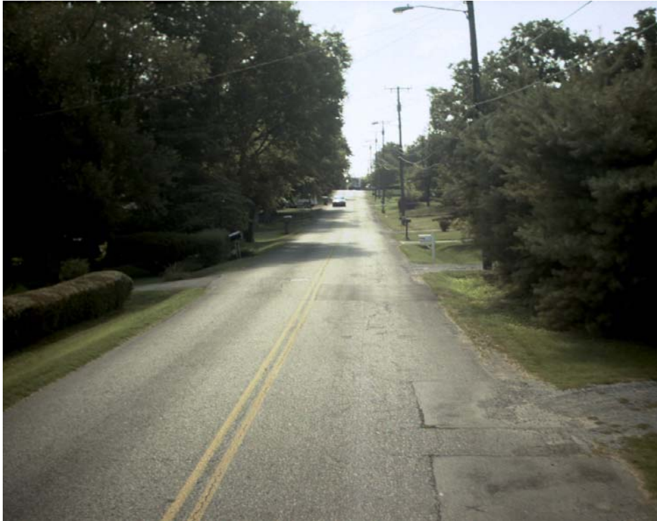
Photo 4.5. Piedmont Avenue, segment 34172, linear cracking, patching, and roughness.
