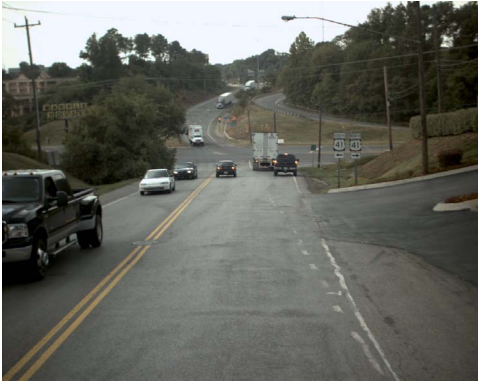
Photo 4.2. Spence Lane, segment 27319, linear cracking, rutting, and roughness.
