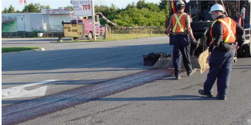
Figure C.8. Pre-treating of a severely raveled centerline joint with a light application of micro-surfacing prior to applying a regular course of micro-surfacing on the entire surface.
