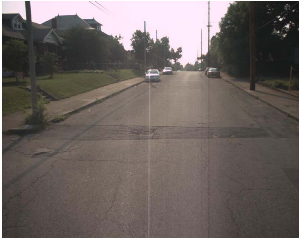
Photo 4.1. Forrest Avenue, segment 3747, block cracking, patching, and linear cracking.
