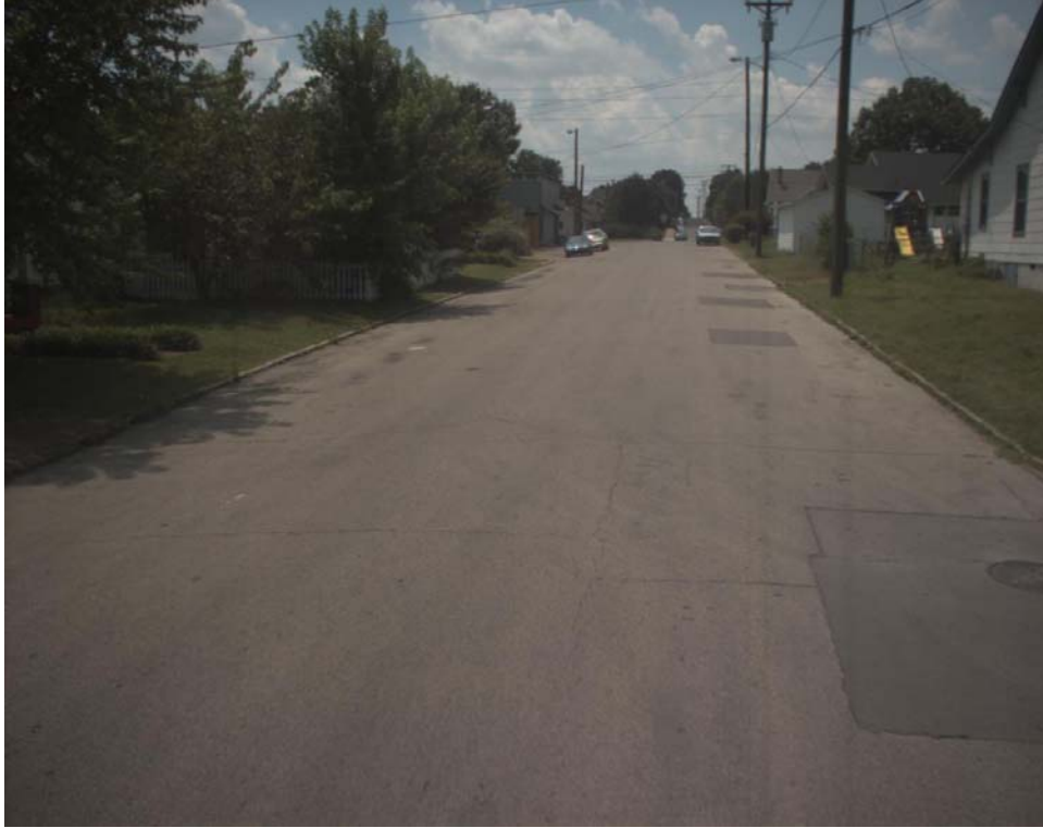
Photo 4.4. Ordway Place, segment 5870, patching, rutting, linear cracking, and block cracking.
