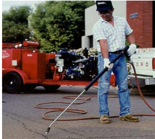
Figure C.22. Routing and cleaning are important to good seal performance.
