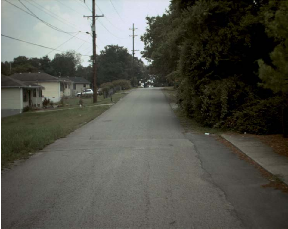
Photo 4.8. North DuPont Avenue, segment 13, rutting, patching, and linear cracking.
