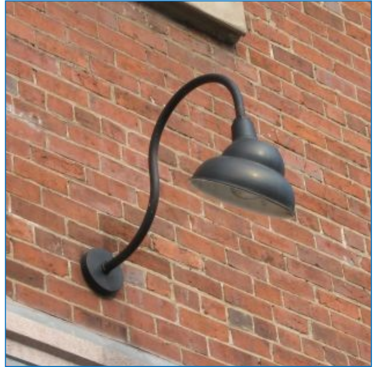
The simple design, inward direction of the light, and dark metal construction of this light fixture make it appropriate.
