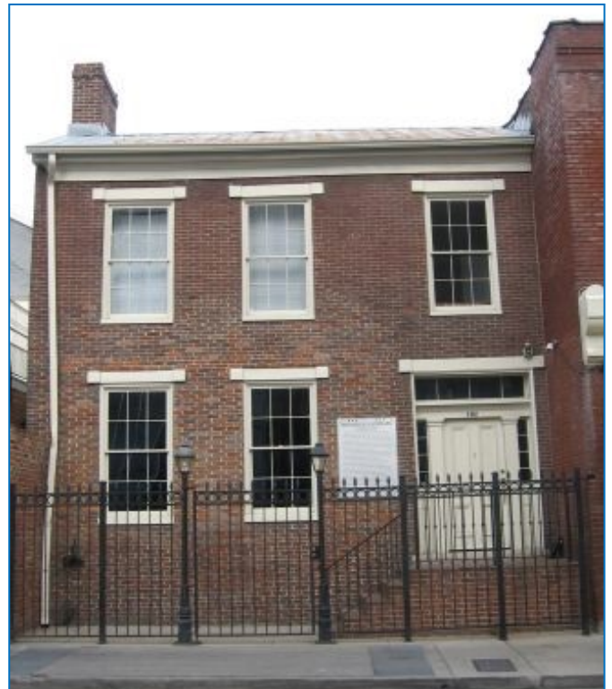
The replacement bricks and brickwork in the lower left portion of this building façade used appropriate bricks, laying pattern, joinery, tooling, and mortaring.
