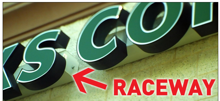
Example of sign with exposed raceway.
