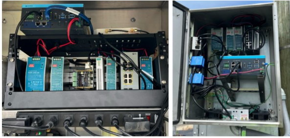
Figure 6. Two styles of pre-fabricated lidar equipment installations developed during Stage I. Left: a drop-in rack mount with lidar equipment, for traffic cabinets with sufficient space. Right: an accessory cabinet affixed onto existing signal cabinets.
